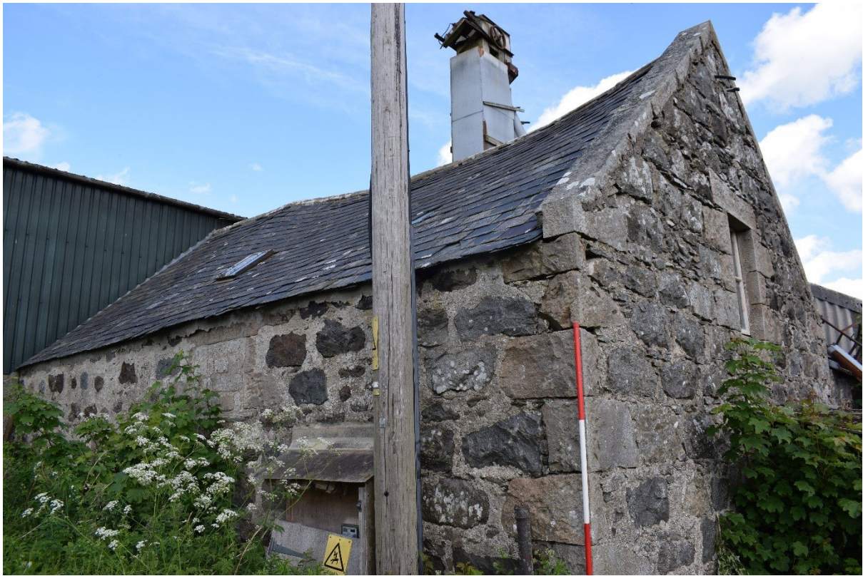
Illus 11 Rooms 4 and 5 with blocked W1 (left), W15 (right) and chute F3 (top centre); facing NW
