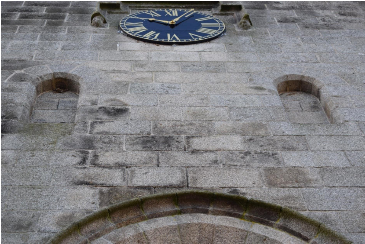
Illus 12 W15 (bottom, W21, W20 with clock F18 with hood moulding F24 with sandstone heads; facing SW
