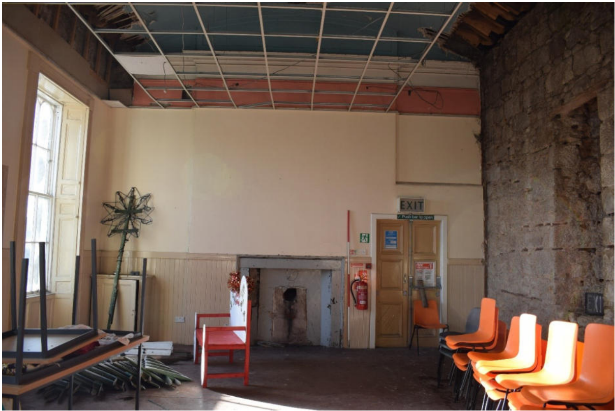
Illus 16 Room 5 SW wall W1 (left), fireplace F7, Phase 3 door D5 and F5 (right); facing SW
