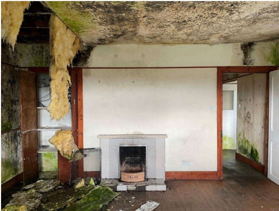
Illus 12 Room 6 N wall fireplace F14 showing collapsing ceilings and rotten floorboards; facing N
