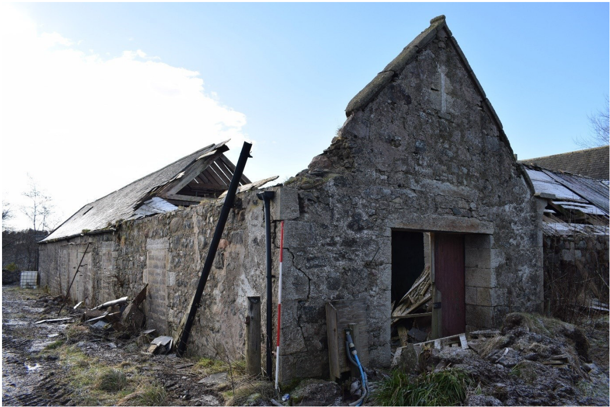
Illus 8 Room 6 NNW end showing collapse of roof; facing SW
