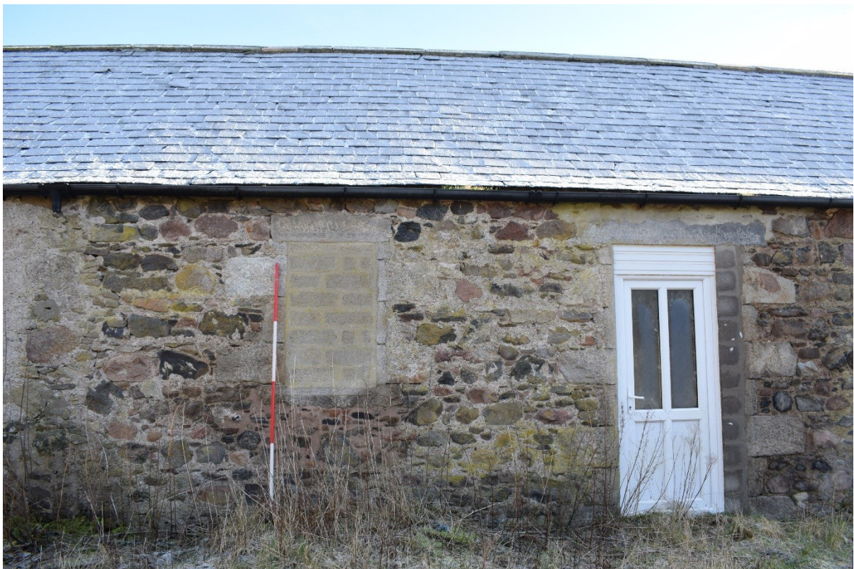
Illus 20 Room 7 WSW wall W6 (left) blocked with breeze blocks and D11 (right); facing ENE
