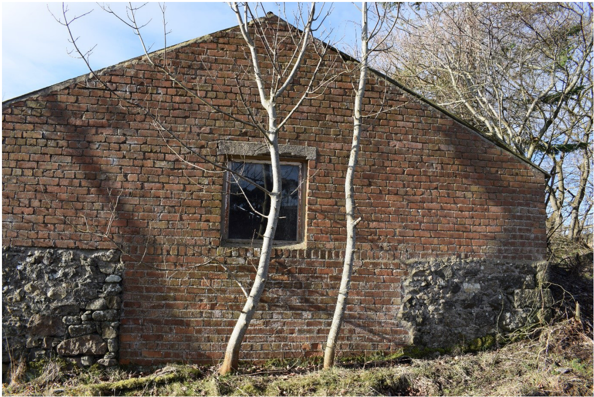
Illus 30 Building 2 ENE wall with W33 (centre) and Phase 1 stone walls; facing WSW
