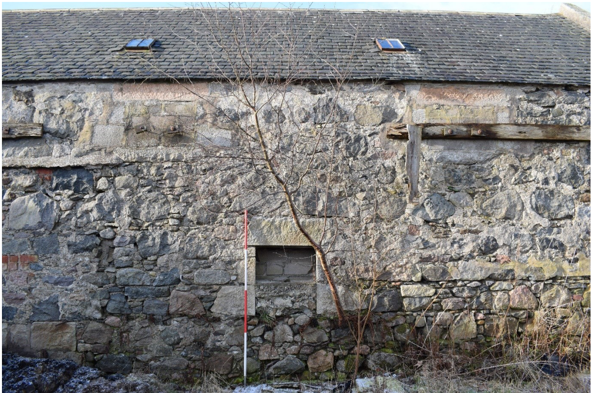
Illus 12 Room 5 ENE wall aperture F13 (centre) with W26 (top left) and W27 (top right); facing WSW
