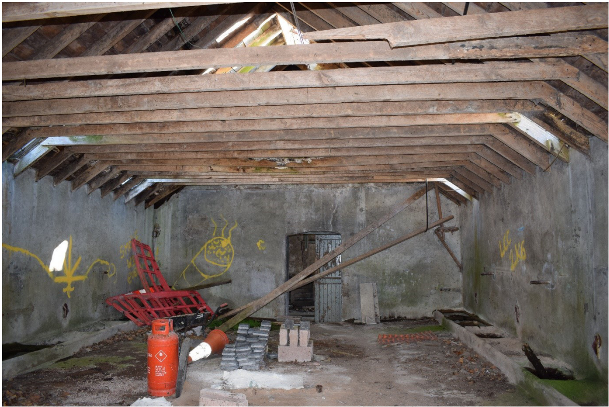
Illus 19 Room 4 ENE wall D24 showing concreted walls and concrete feeders F20; facing ENE
