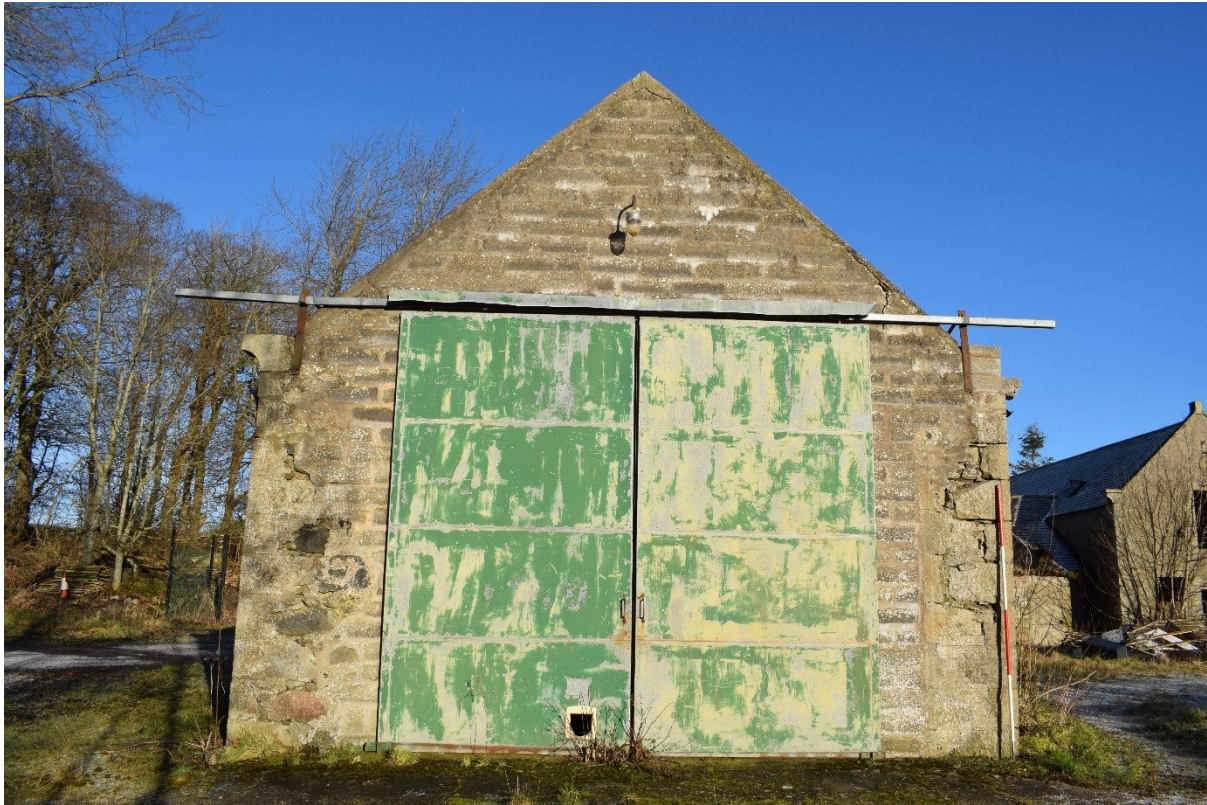
Illus 18 SSE gable Room 1 D1 with rebuilding in breeze block; facing NNW
