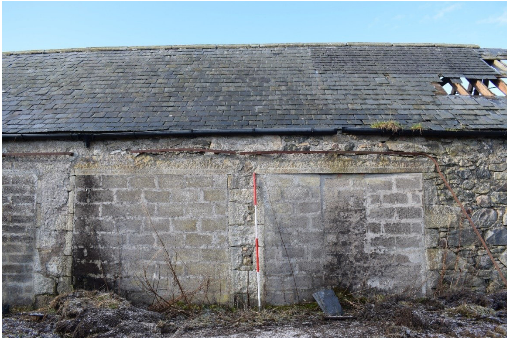
Illus 22 Room 7 ENE wall D16 (left) D17 (right) former cart doors infilled with breeze blocks; facing WSW
