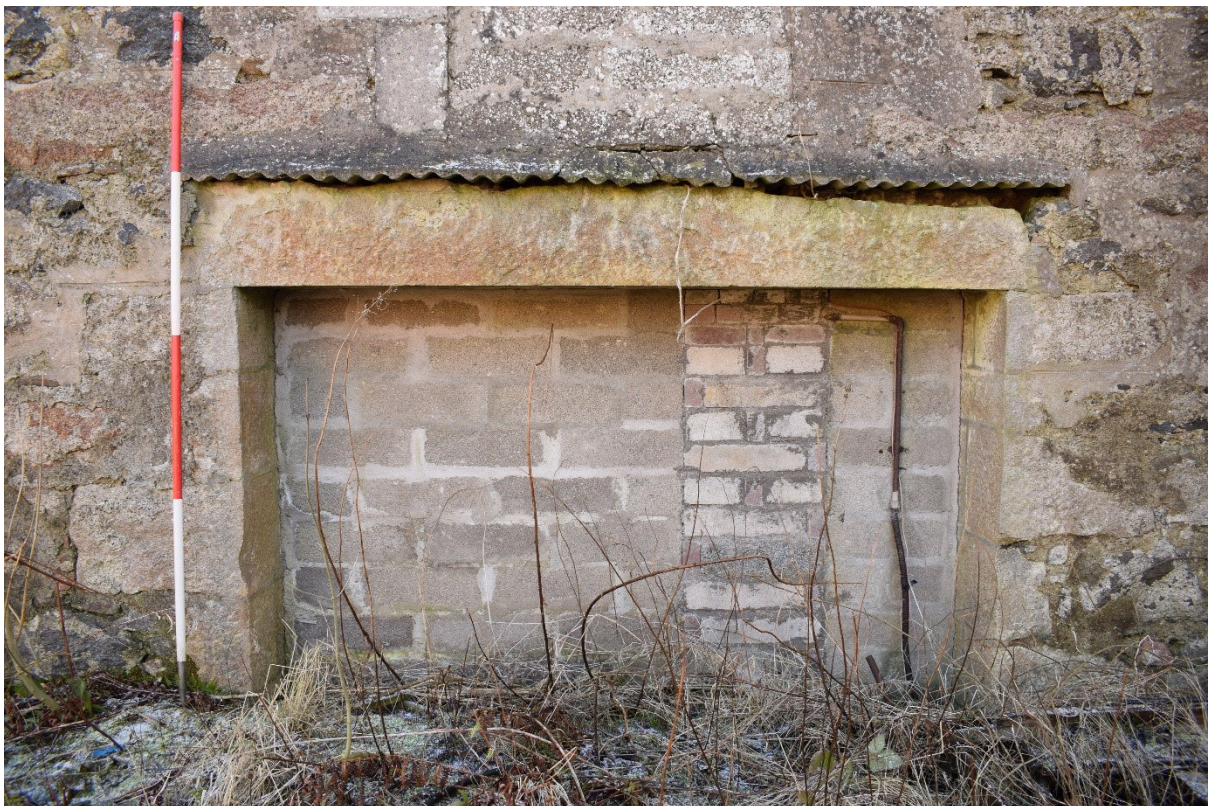
Illus 13 Room 5 NNW wall D27 with infilled W28 above; note foreground infilled with soil; facing SSE
