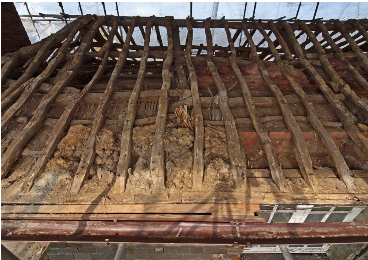
Fig 18 Roof: south side, towards west end (note lath and plaster ceiling, evidence for partition and cob wall-top between rafters)
