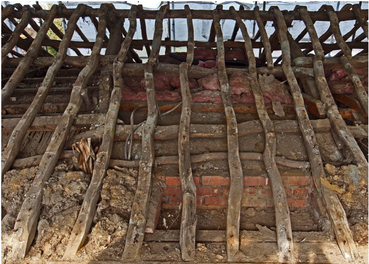
Fig 19 Roof: south side, left (west) of centre (note lath and plaster ceiling, evidence for partitions left and right, cob wall-top between rafters, brick rebuild over inner window lintel and treenail hole in outer lintel)
