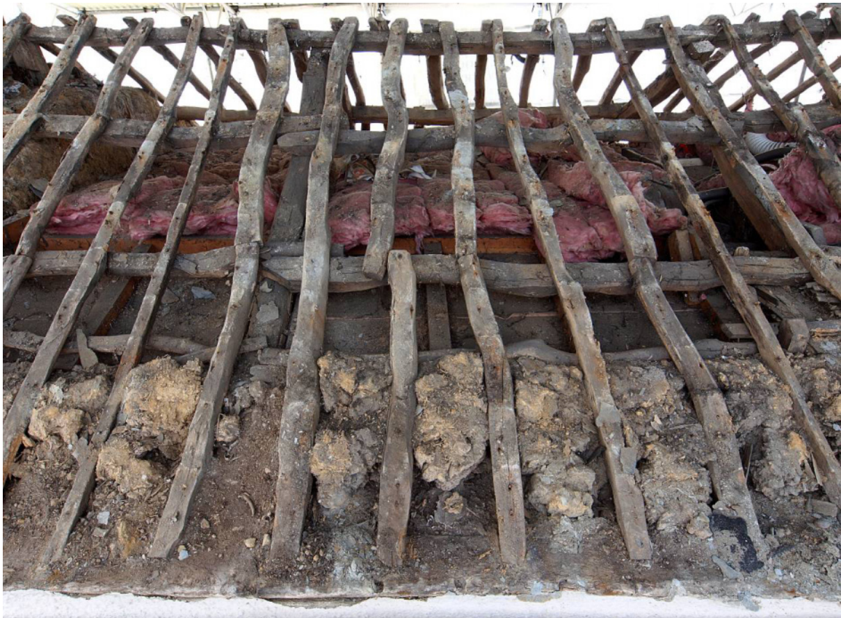
Fig 12 Roof: north side, east end: random (grown) shapes denote probable local oak; straighter common rafters are reused ship's timbers (note purlins and some common rafters span short distances)
