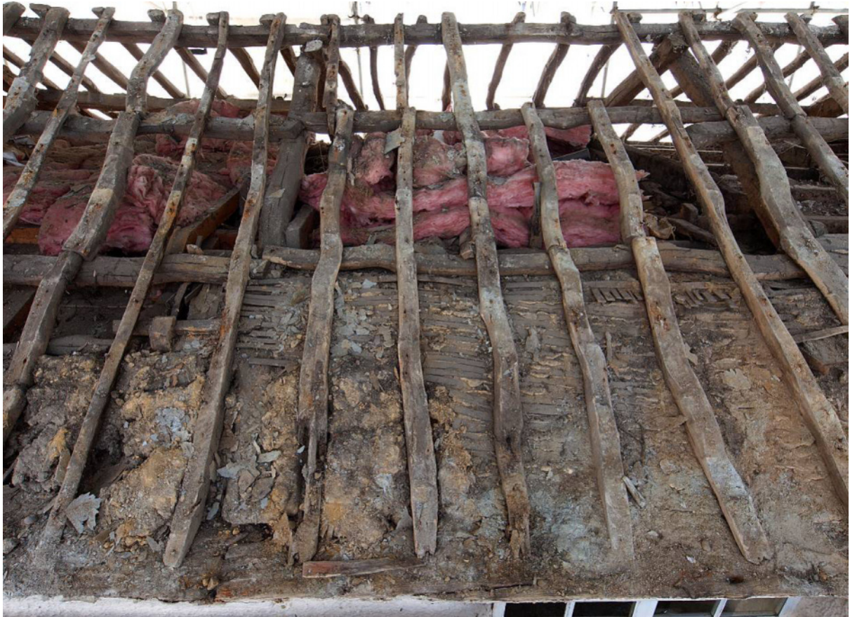
Fig 13 North roof slope right (west) of centre (note upper part of partition left of left-hand roof truss and remains of lath and plaster ceiling right of same truss)
