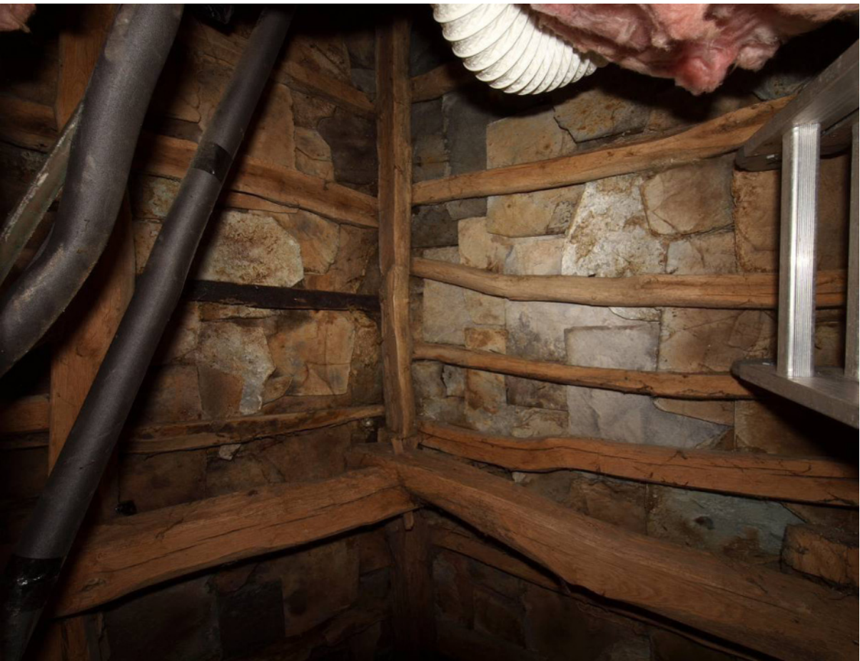
Fig 10 Roof from below (note reused ship's timbers as common rafters left of ridge)
