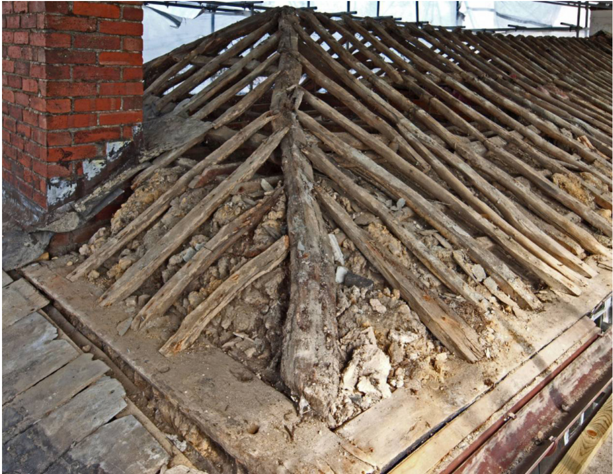
Fig 17 Roof structure from S (note treenail holes in reused wall-plate at hipped end)
