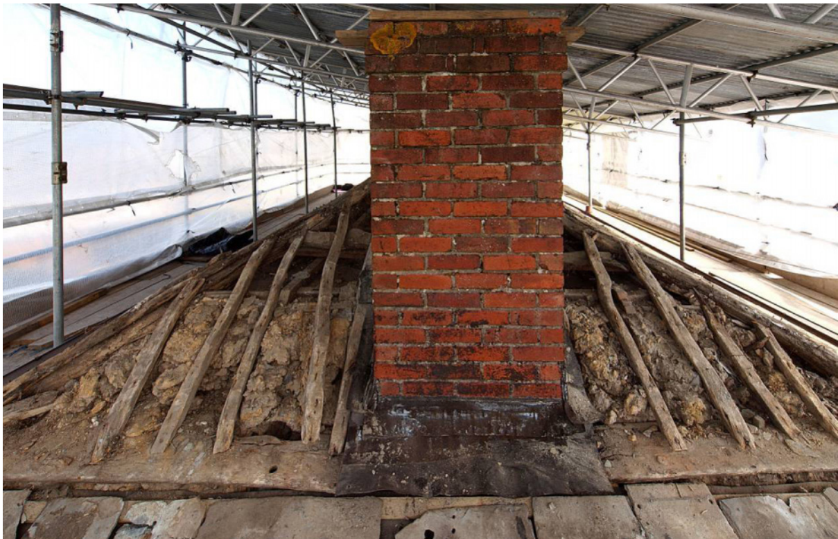
Fig 16 Roof structure of hipped SW end: central part of wall-plate (reused ship's timber) of hip cut away when present brick stack constructed
