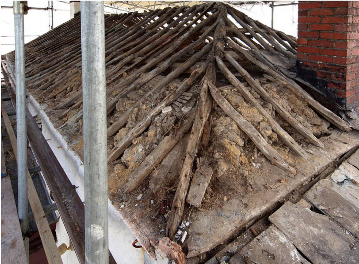
Fig 15 Roof structure from W: central part of wall-plate (reused ship's timber) of hip cut away when present brick stack constructed
