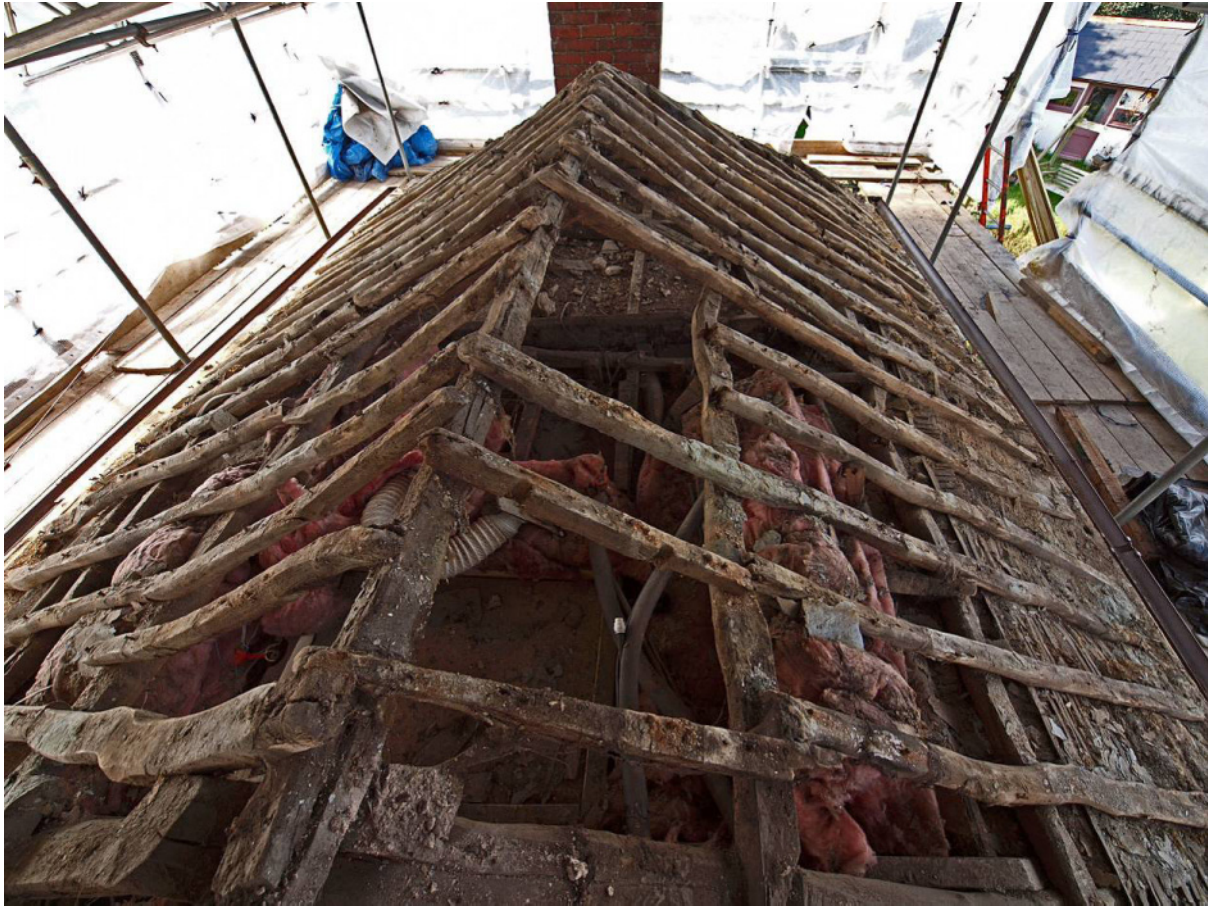
Fig 21 Roof from above facing west (note reused notched rafter at centre of image)
