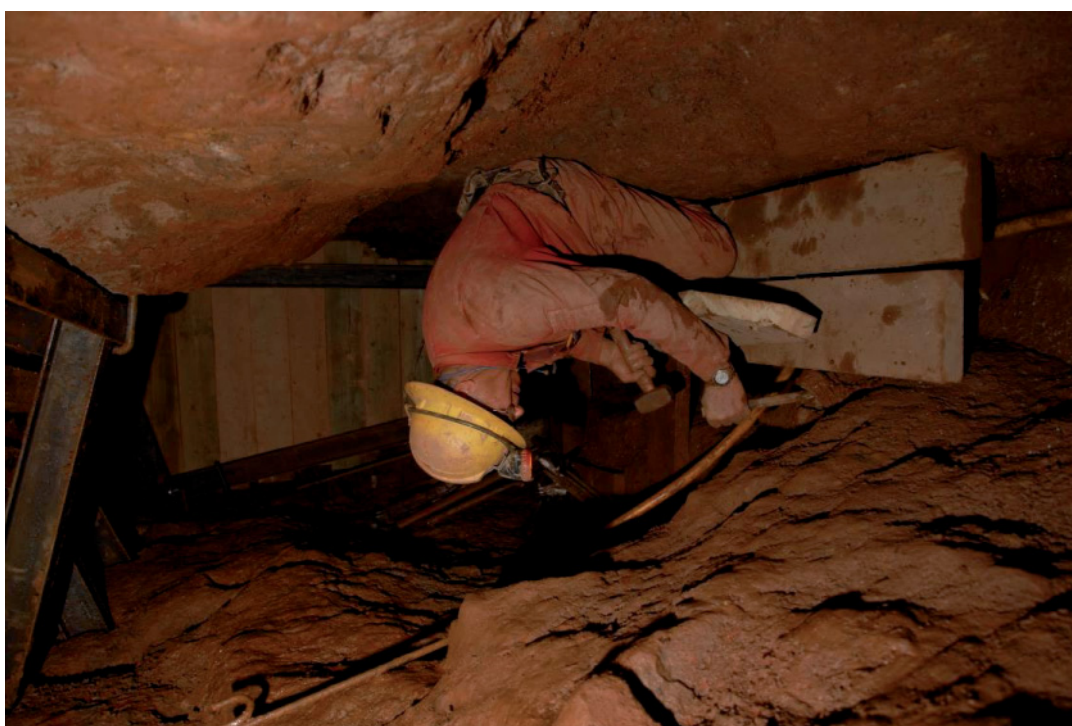
Fig 37. Mervyn Brakespear constructing the planked floor at the southern end of the eastern drive.
