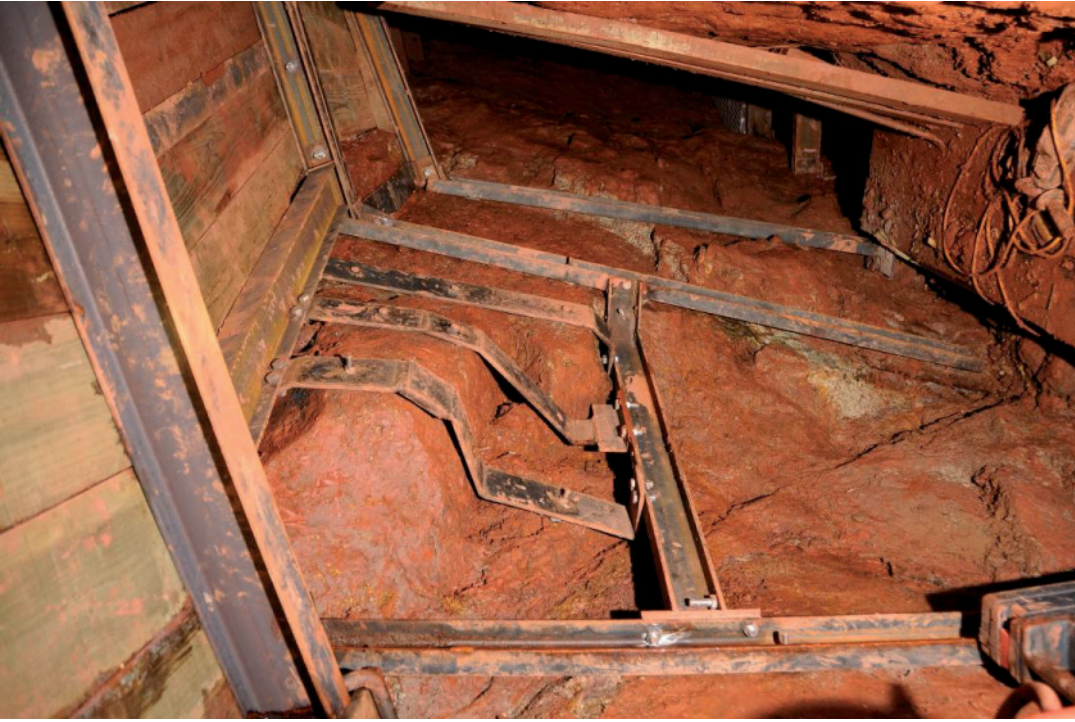
Fig 40. The steel channels and strapping used to create the necessary support for the weak section of the hanging wall in the eastern stope.
