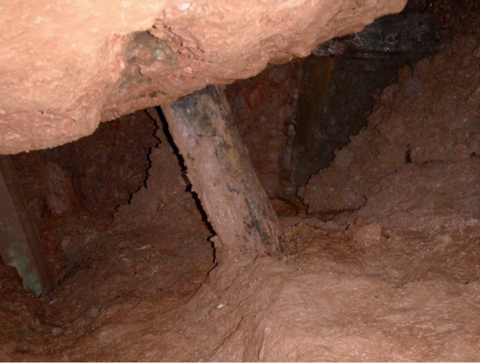
Fig 20. Some of the original timber stulls in the eastern drive. Note also the timber support lower right, which supported an overhanging section of the hanging wall.
