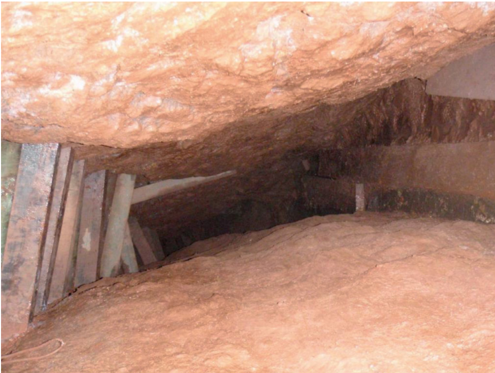
Fig 19. Looking up the eastern drive at an early stage of the works, showing the timber stulls on which the cover boards were set. The planks on the floor kept the contractors from sinking into the slimes filling the base of the stope.
