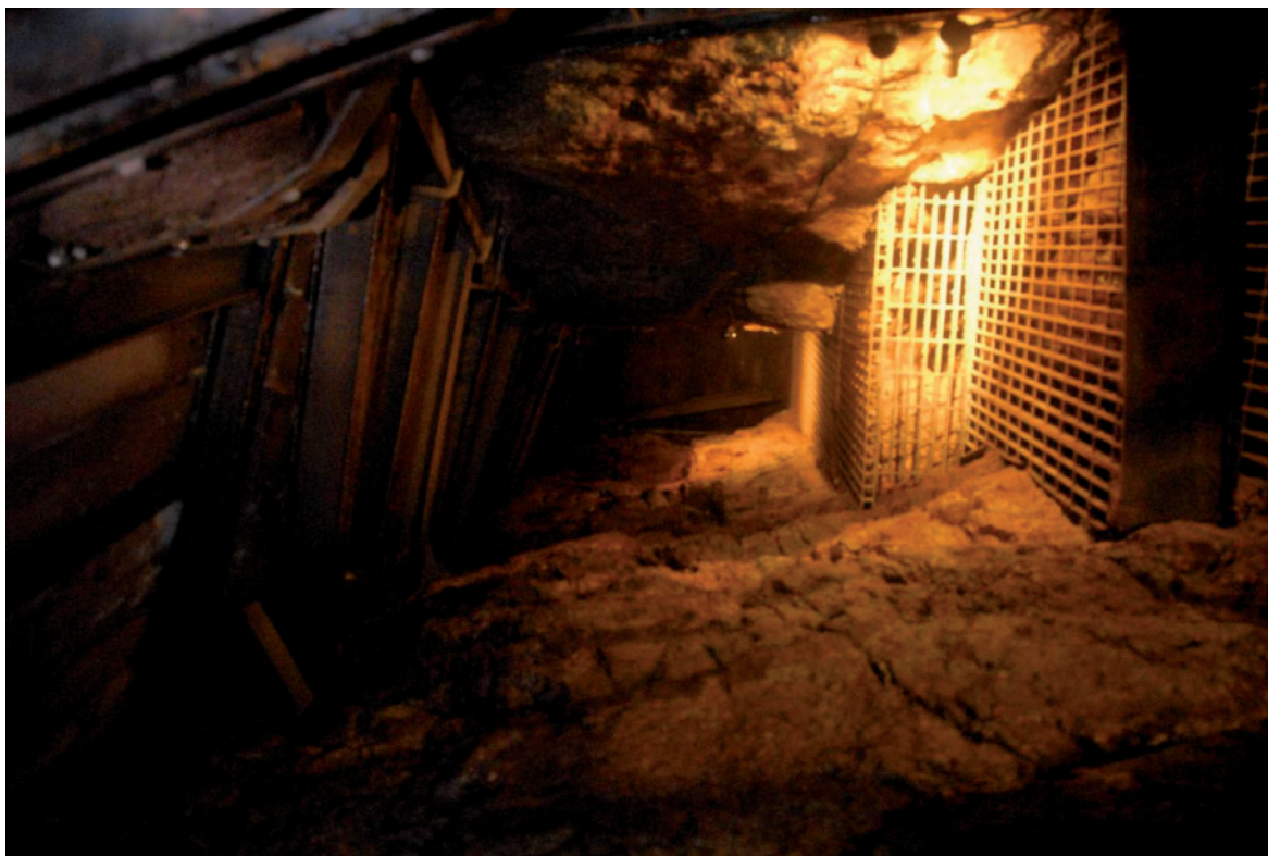
Fig 67. Looking south along the eastern drive showing the mesh flooring over the stope and the steel roof supports.
