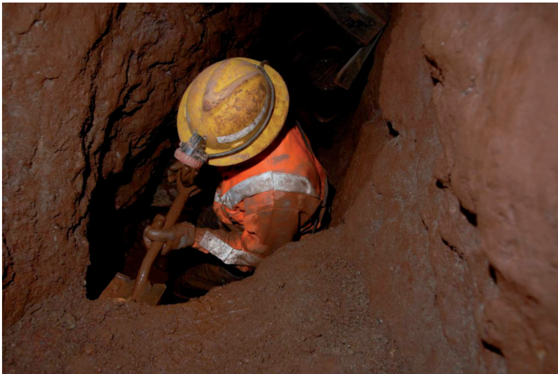
Fig 22. Nick Hall, one of the CSM students working with the contractors, excavating spoil from the western branch of the adit system.
