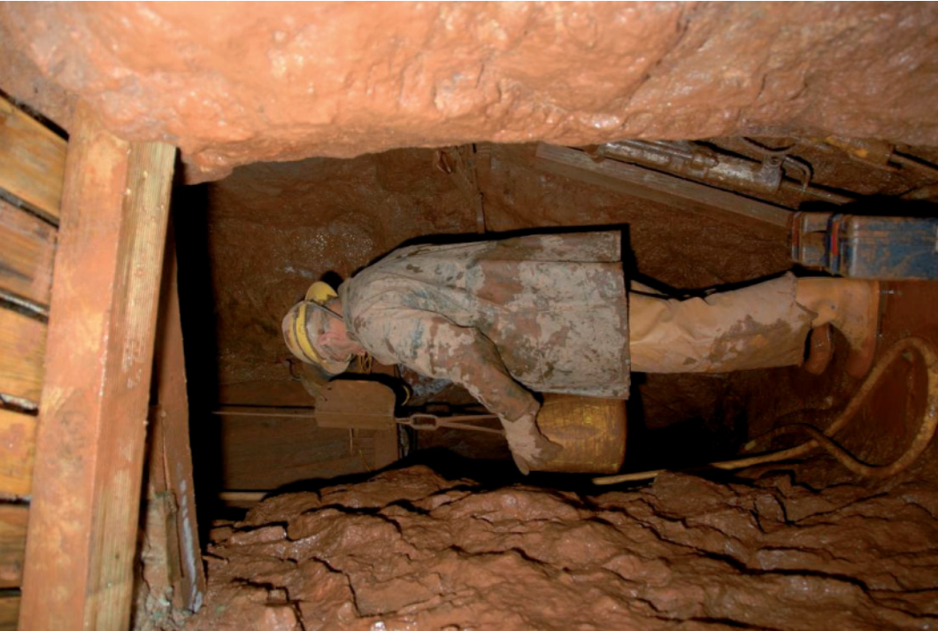
Fig 23. Mervyn Brakespear (Drillserv) attaching a bucket of spoil excavated from the eastern drive to the hoisting cable in East Sulphide Bay Shaft prior to it being hauled to surface for disposal.
