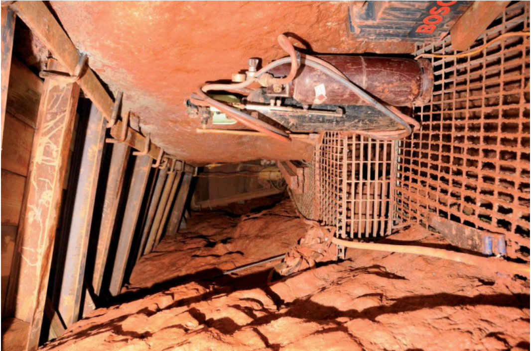
Fig 41. The completed steel mesh flooring in the eastern stope, showing the greatly reduced headroom between the floor and the roof support at this point in the adit system.
