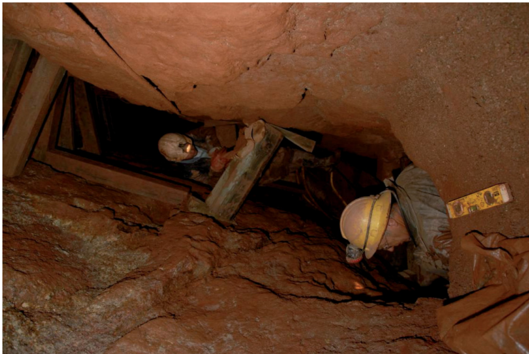
Fig 32. Work under way in the eastern drive, showing the permanent and temporary timberwork to support the hanging wall (Mervyn Brakespear and John Dowling shown at work).
