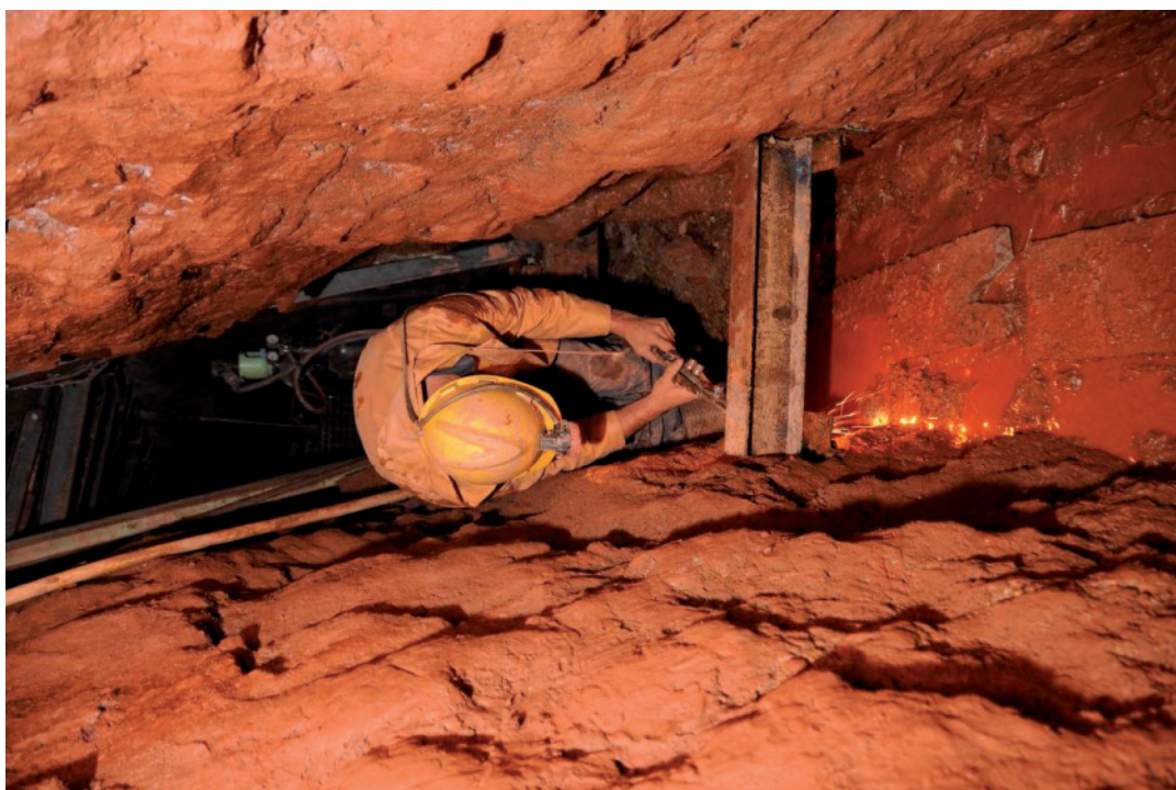
Fig 38. Pat Orient flame cutting a low level floor support UB to length in the eastern drive.
