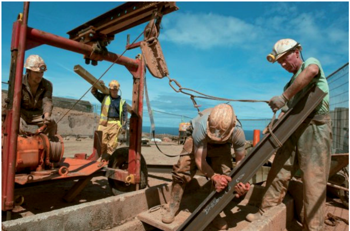
Fig 26. The air winch was also invaluable in getting heavy or bulky materials underground, in this case the UBs used to support the coverings over Windlass Shaft. From L-R Colin Davies, Douglas Wheatcroft, John Dowling and the Author. Photo © and courtesy of Bernie Petterson.
