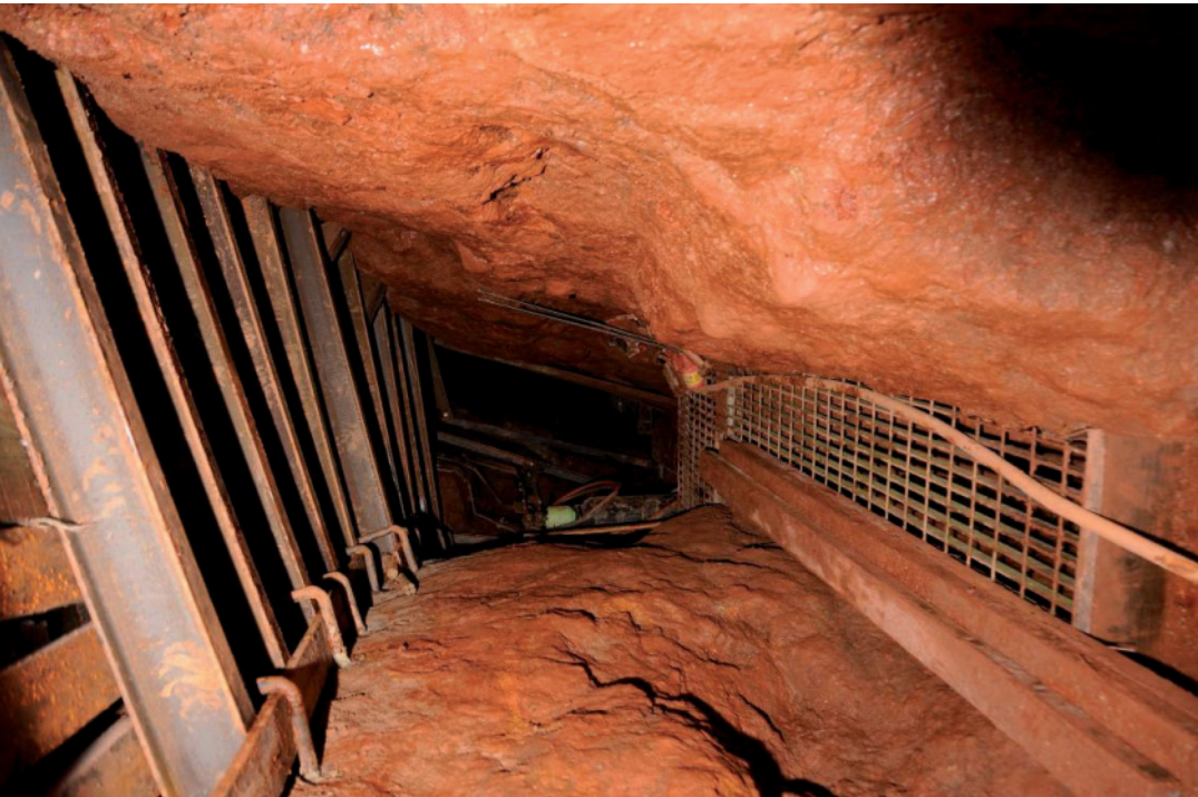
Fig 39. The steel mesh floor set on UBs installed over most of the length of the eastern stope.
