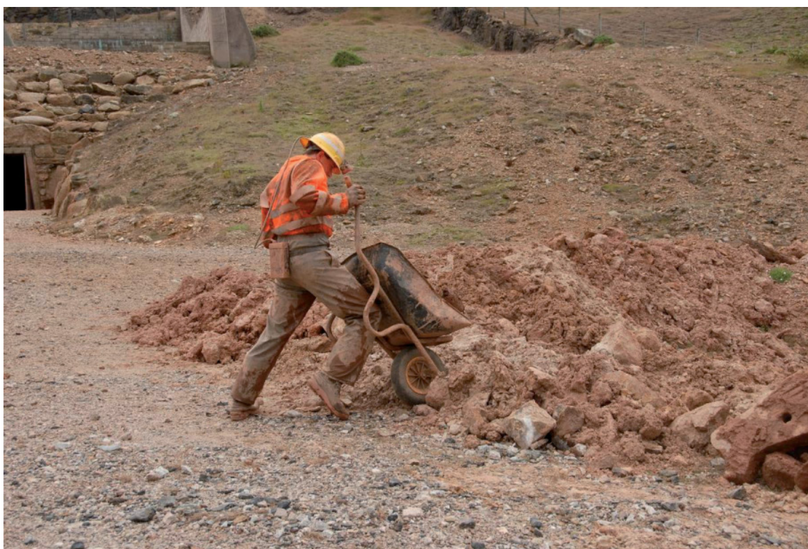
Fig 28. Once carried by bucket to the adit exit, the material was barrowed to the agreed dumping area not far downslope (Nick Hall tipping the barrow).
