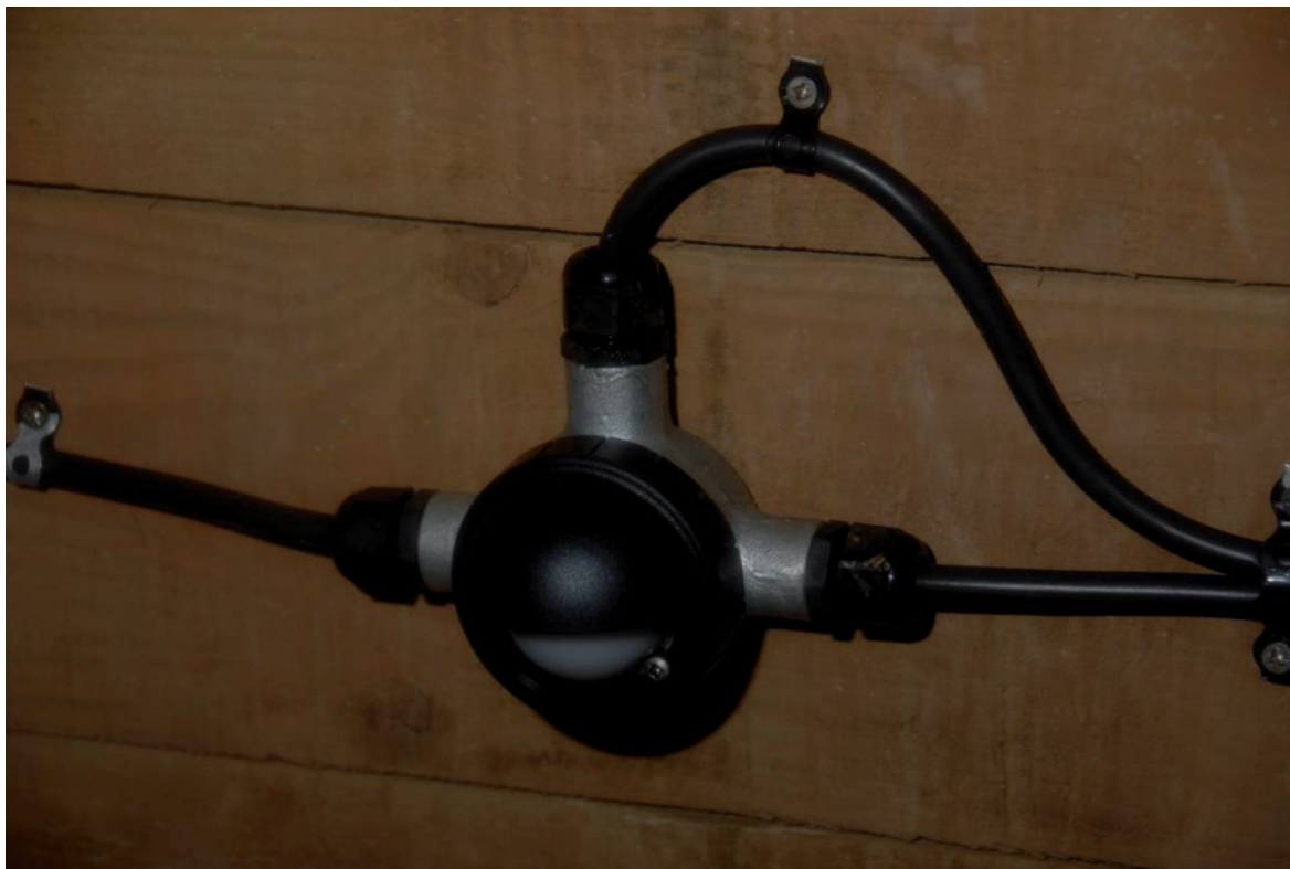
Fig 64. One of the Blue Dome LED lighting units, fitted with a cowl which effectively directs the light. The majority of the cowls on the low level lights were angled so as to light the route ahead.
