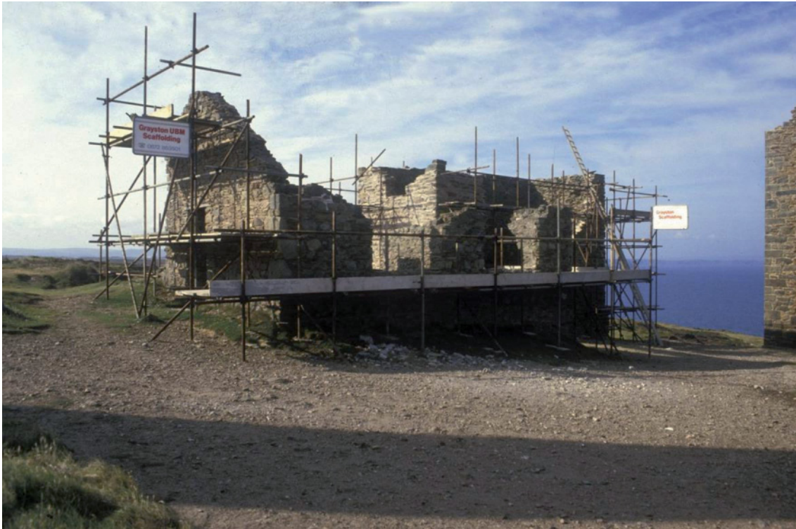
Fig 96. Conservation work under way on the horizontal whim engine house [190376] (foreground) and all-indoor beam whim engine house [190378] (behind) during 1986. Adam Sharpe Collection.
