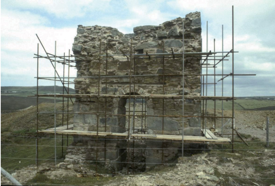
Fig 135. The bob wall of Great Wheal Charlotte pumping engine house in 1987 during conservation works undertaken by the NT. Adam Sharpe Collection.
