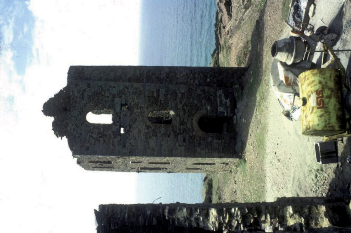
Fig 92. A view of the stamps engine house [190381] prior to its conservation in 1986. Adam Sharpe Collection.
