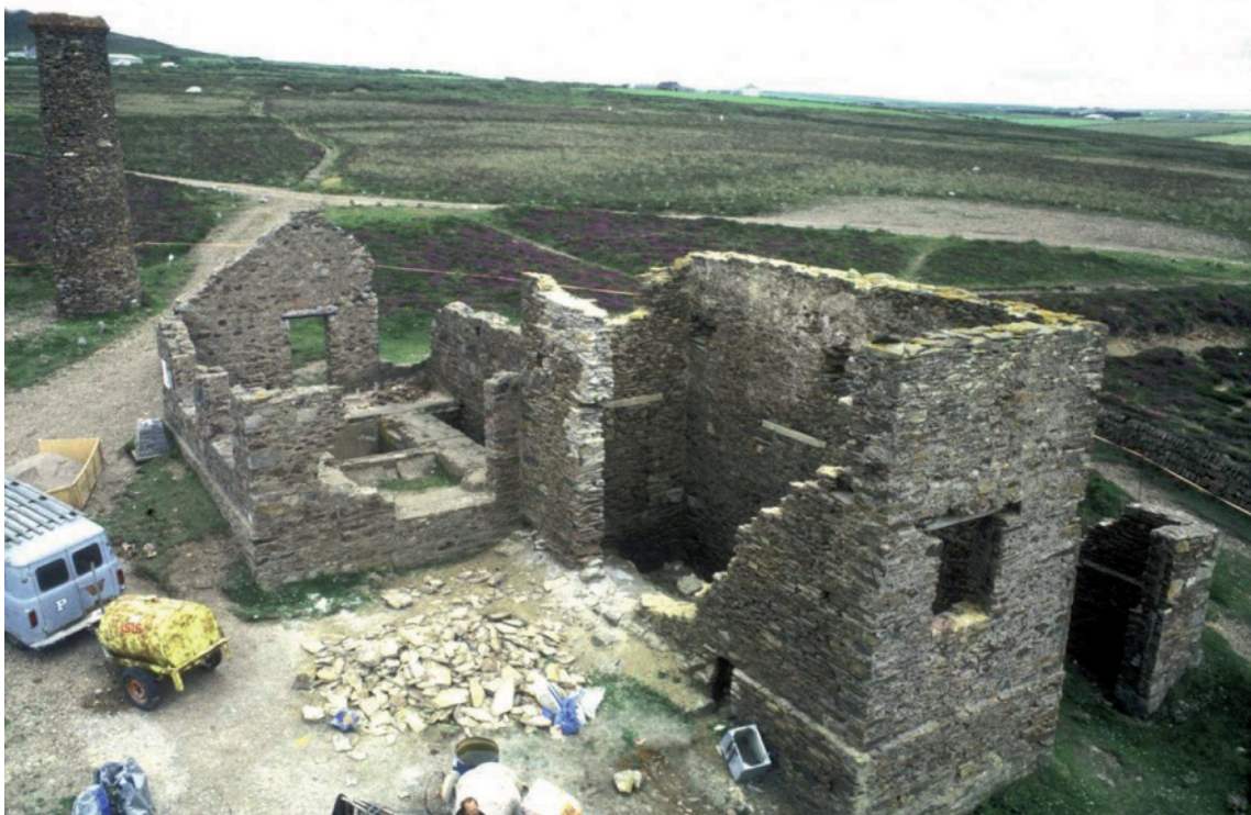
Fig 95. Conservation work under way to the horizontal whim engine house [190376] (left) and all-indoor whim engine house [190378] (right) during 1986. Adam Sharpe Collection.
