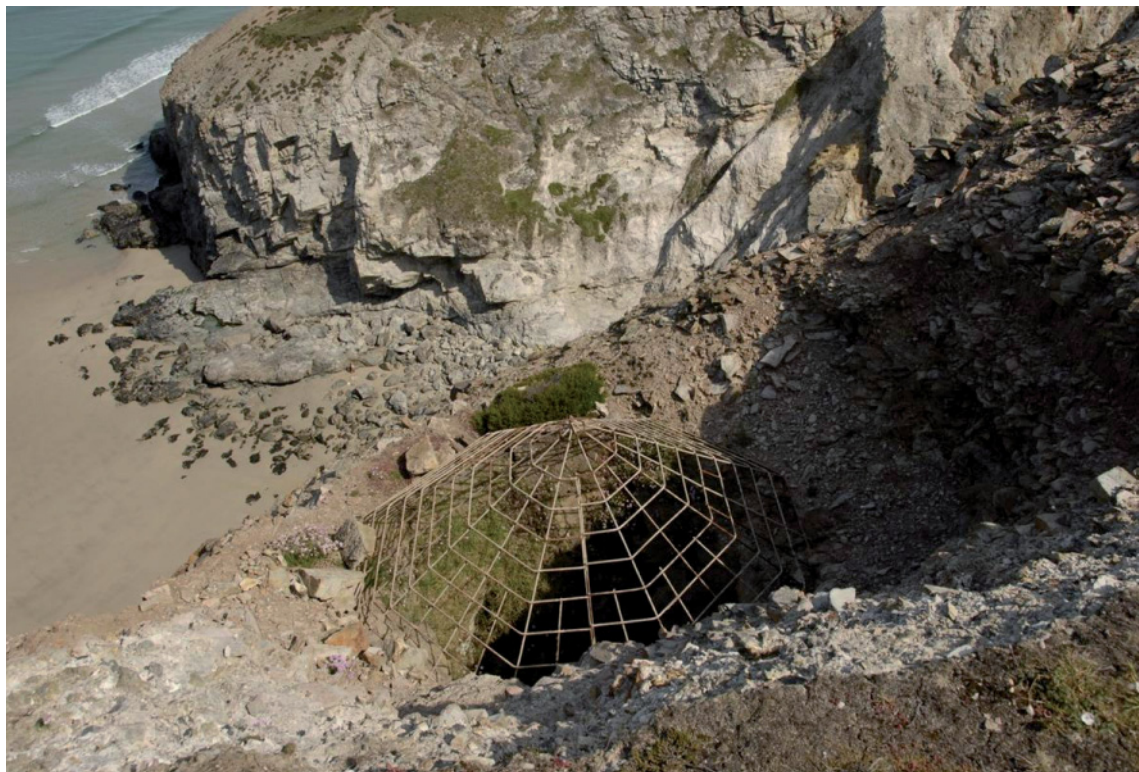
Fig 126. Midwinter's Shaft and its Chyd Cap set right on the edge of the cliff above Porthgwidden Cove. The shaft is open to at least adit level below. HE Archive.
