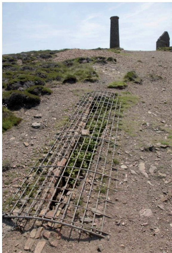
Fig 99. The collapsed near-surface section of the brick-arched calciner flue [190349] with the galvanised grille placed over it to protect visitors from injury. HE Archive.
