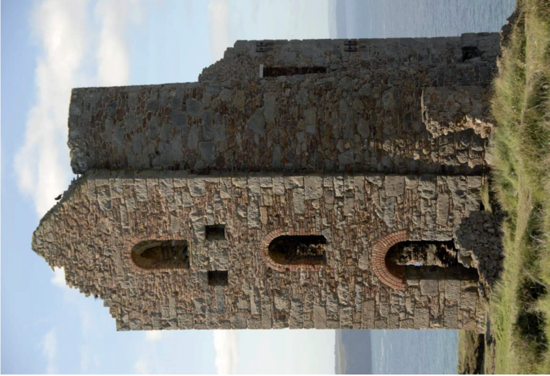
Fig 93. The stamps engine house [190381] following its conservation. On this elevation the replacement of some failed pointing and minor rebuilding of the cable were all that were undertaken. HE Archive.
