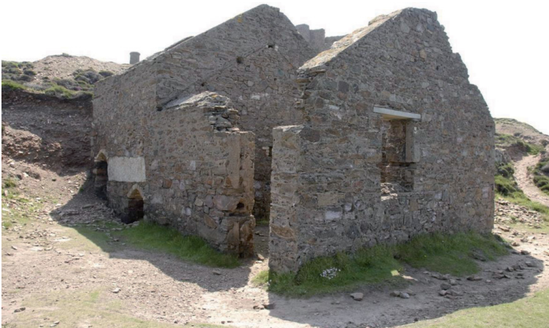
Fig 97. The reverberatory arsenic calciner [190346] seen from the north-west. The nearest section of the building housed the stoking area, whilst the calcining beds are in the farther section of the structure. The arched opening at the rear gives onto one of the twin hearths, whilst the nearer arch is the discharge opening. Matching openings are found on the opposite side of the building. HE Archive.
