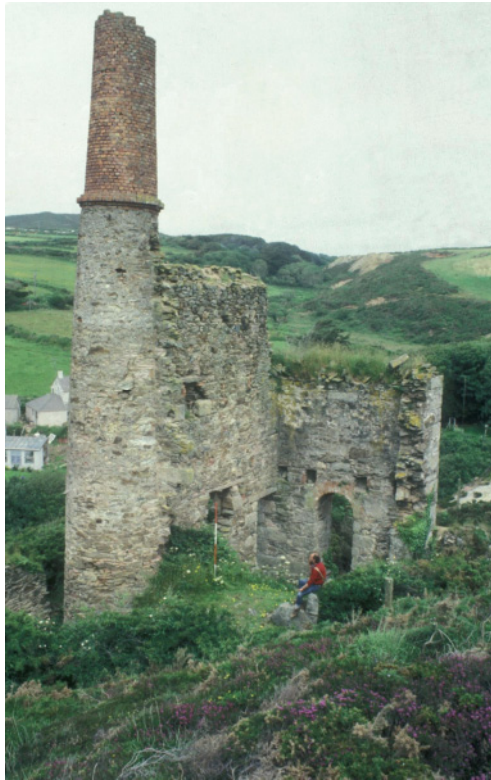
Fig 145. Charlotte United pumping engine house [190616] from the south-west prior to its conservation between 1989 and 1993. Although the building has now been stabilised, its boiler house [190617] still requires attention, and the expanding shaft cone threatens to undermine the bob wall. Adam Sharpe Collection.
