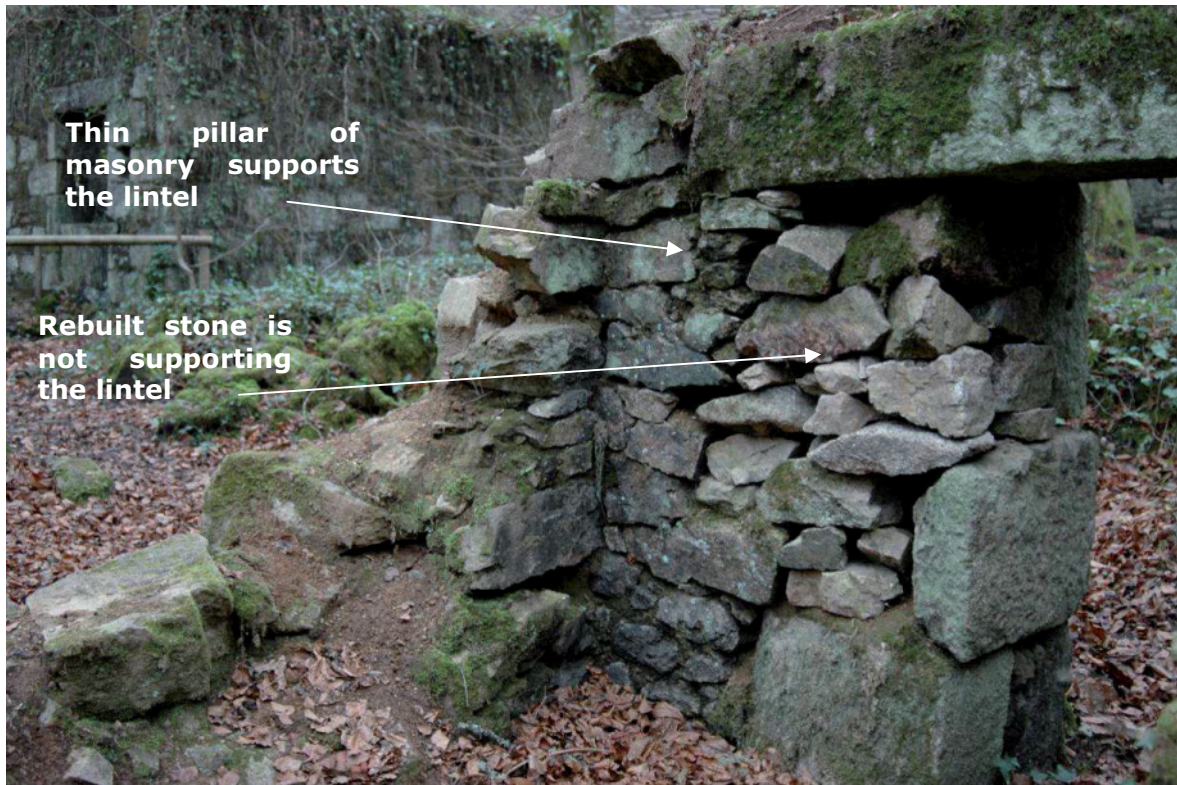
Fig 11 Barely supported lintel of cask house
