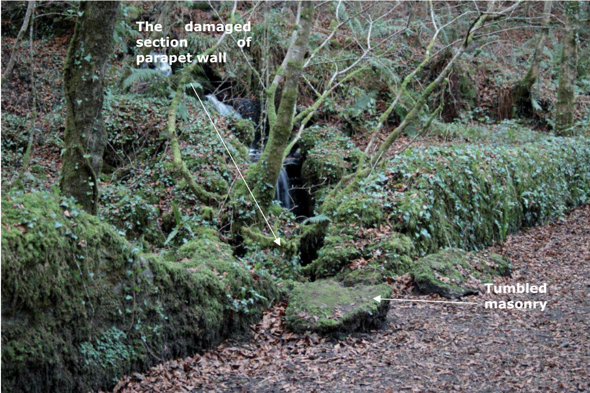
Fig 20 Damaged parapet of causeway leading to bridge, from the east (above) and from the south (below)
