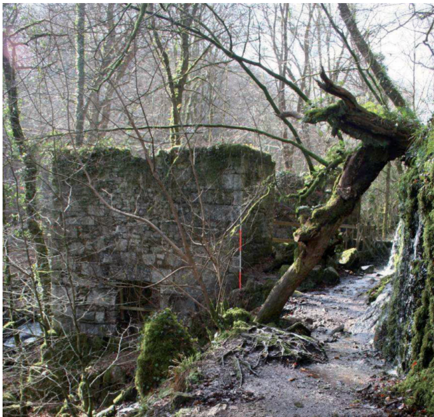
Fig 23 Examples of tree damage at Kennall Vale: the top picture shows where a tree rooted into a bridge abutment has fallen and taken a large quantity of stone with it; the lower shows where a tree has fallen onto the path which runs beside the leats, linking the incorporating mills. This path is used by most visitors
