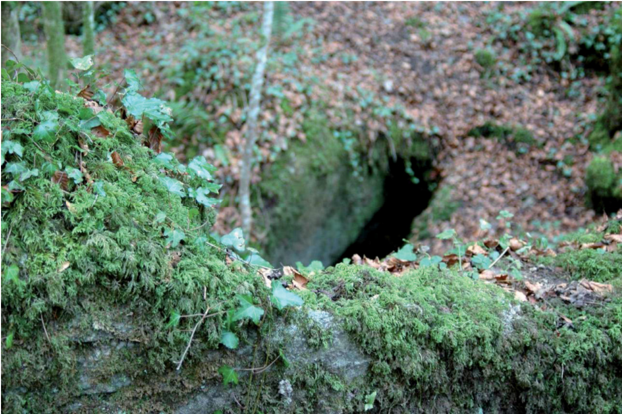
Fig 18 Hole above culvert adjacent to bridge
