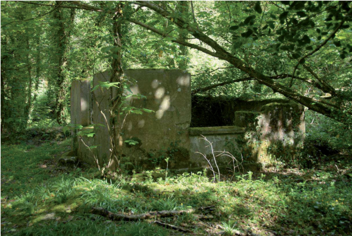
Fig 48. The ruinous rendered blockwork building [28] to the east of Big Wheel Mill. HE Digital Image Archive.
