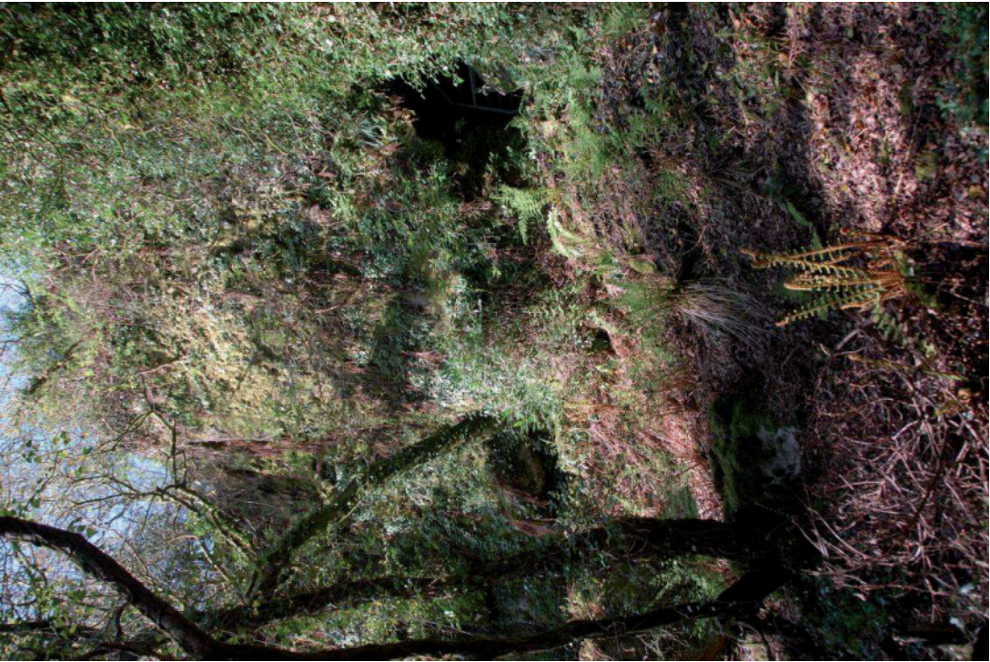
Fig 27 A typical view in the secluded interior of Wheal Arthur Quarry [1]. The quarry lies outside the area managed by the Tregargus Trust. HE Digital Image Archive.
