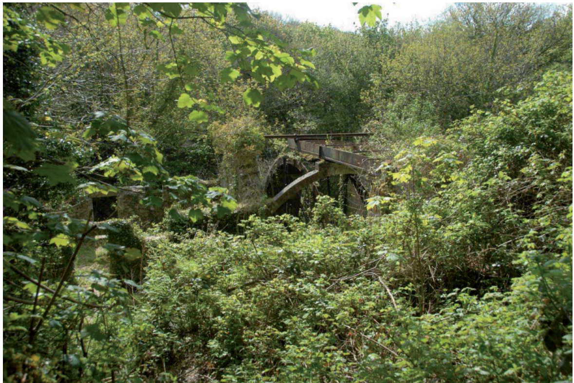
Fig 63. The iron launder serving the central water wheel at Big Wheel Mill, seen from the site of its reservoir just to the west. HE Digital Image Archive.
