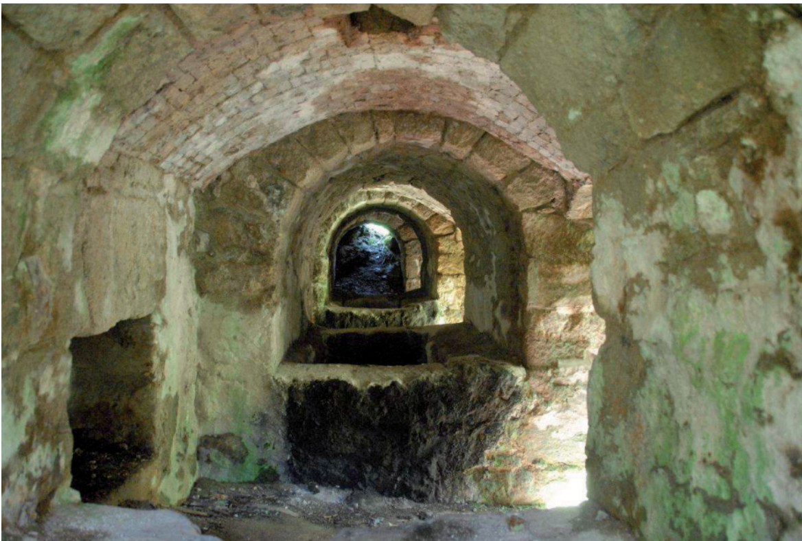
Fig 65. The ground level power vault running beneath Big Wheel Mill. HE Digital Image Archive.
