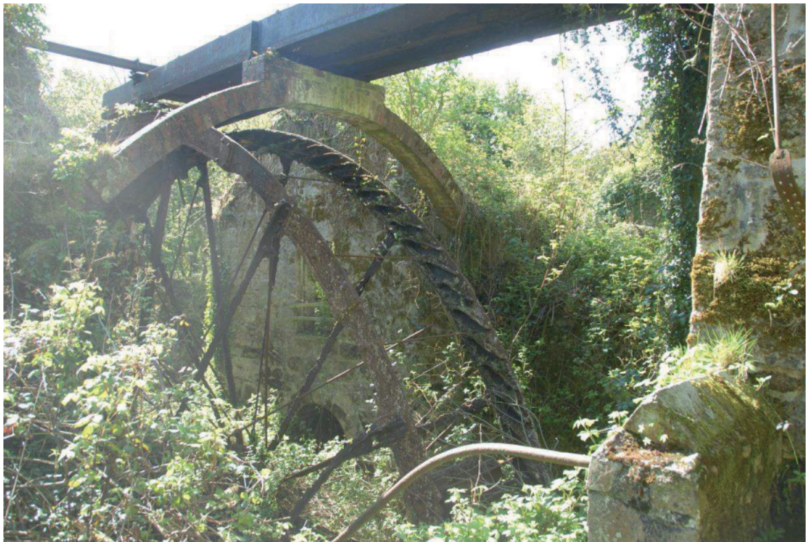
Fig 67. The central water wheel, arched brick launder support and cast iron launder at Big Wheel Mill, seen from the north-west. HE Digital Image Archive.
