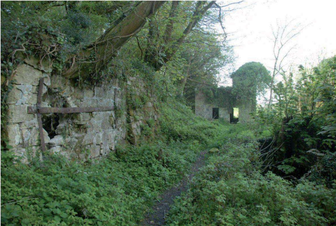
Fig 76. Trees growing out of the stonework of the Trevear Mill reservoir [33] are already causing significant damage to it. Their collapse would also damage Trevear Mill immediately to the right. HE Digital Image Archive.
