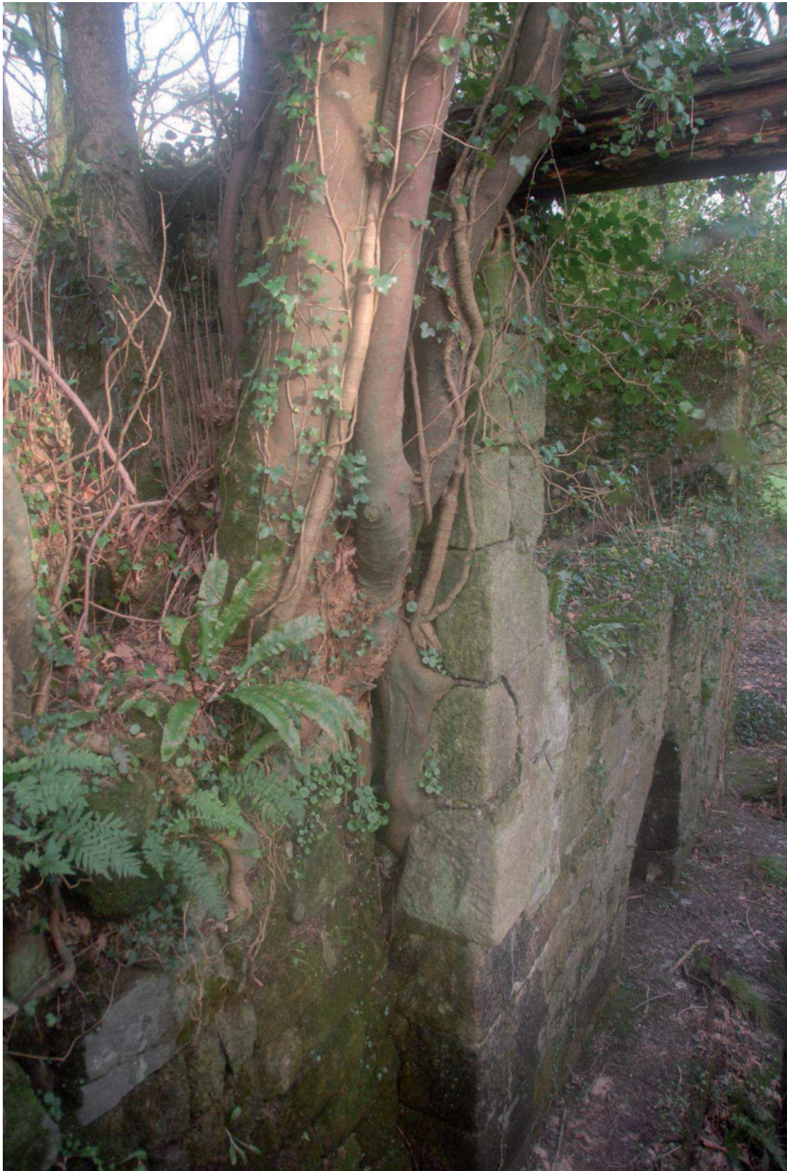
Fig 92. Tree roots infiltrating the masonry on the northern side of the wheelpit at Mica Mill exemplify the types of problems affecting sites at Tregargus which require urgent attention if this rare group of structures are not to suffer severe deterioration. HE Digital Image Archive.
