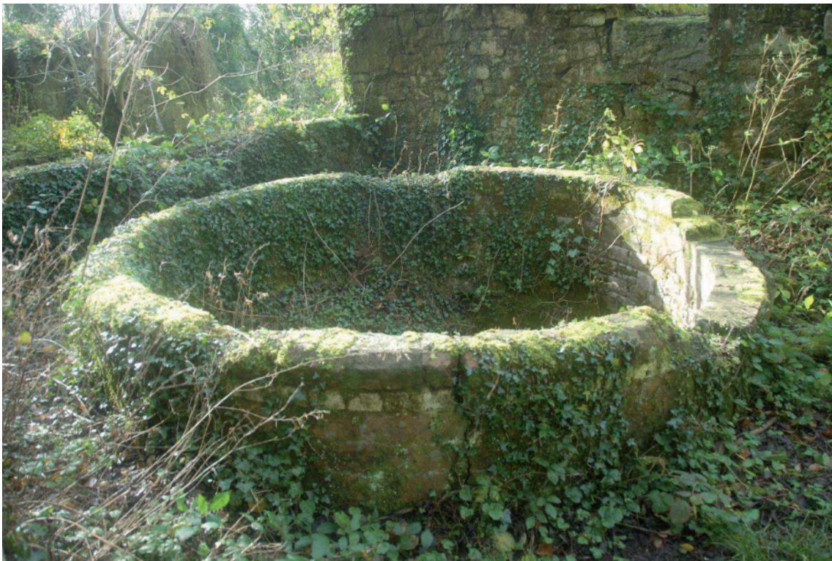
Fig 77. One of the brick-built grinding pans in the northern section of Trevear china stone mill. HE Digital Image Archive.
