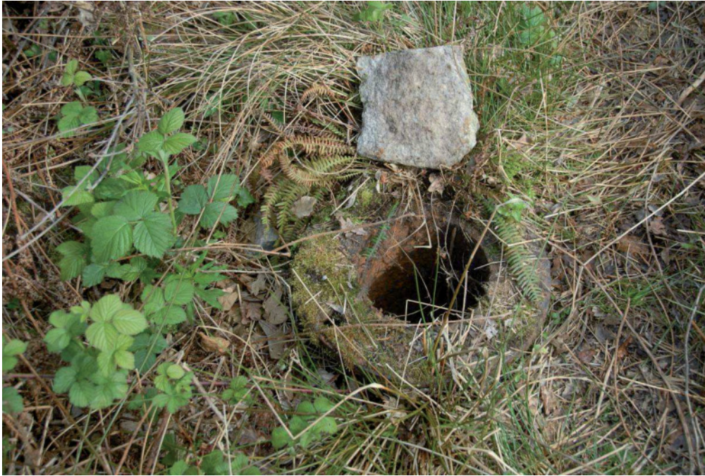
Fig 38. The top of the cast iron rising main adjacent to the pumping shaft [8] at Wheal Arthur mill. HE Digital Image Archive.
