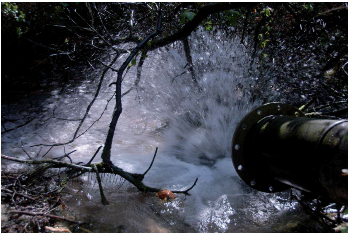
Fig 30. The overflow water discharge from the pond above the Wheal Arthur complex, just to the north of the area managed by the Tregargus Trust. HE Digital Image Archive.
