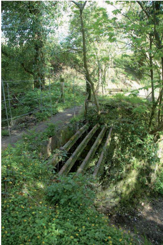
Fig 85. A view of the aqueduct/tramway bridge [38] seen from the south. The cast iron leat bridge has been infilled to form a path, whilst the deck of the tramway has been lifted, leaving only its support rails. HE Digital Image Archive.
