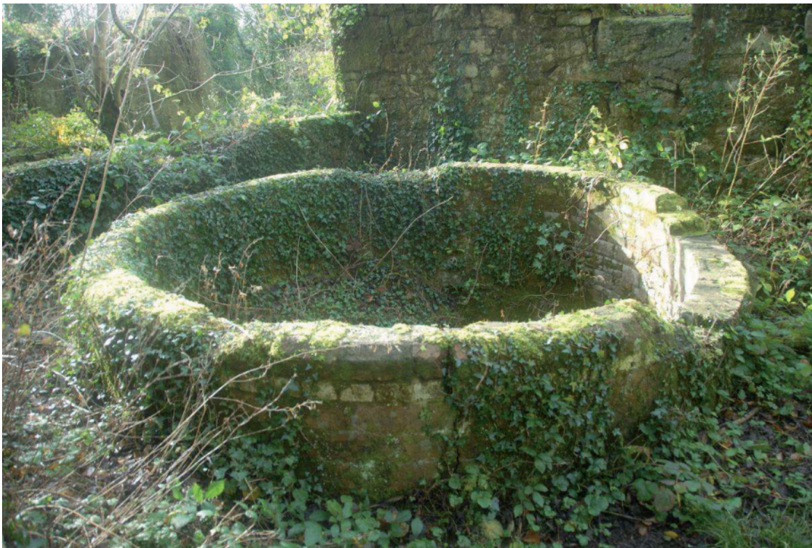
Fig 77. One of the brick-built grinding pans in the northern section of Trevear china stone mill. HE Digital Image Archive.
