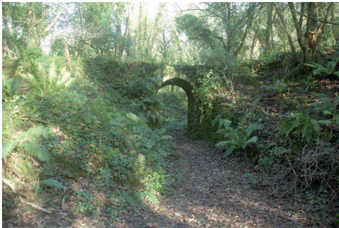
Fig 51. The recently-consolidated tramway bridge over the roadway to the east of Big Wheel Mill. HE Digital Image Archive.
