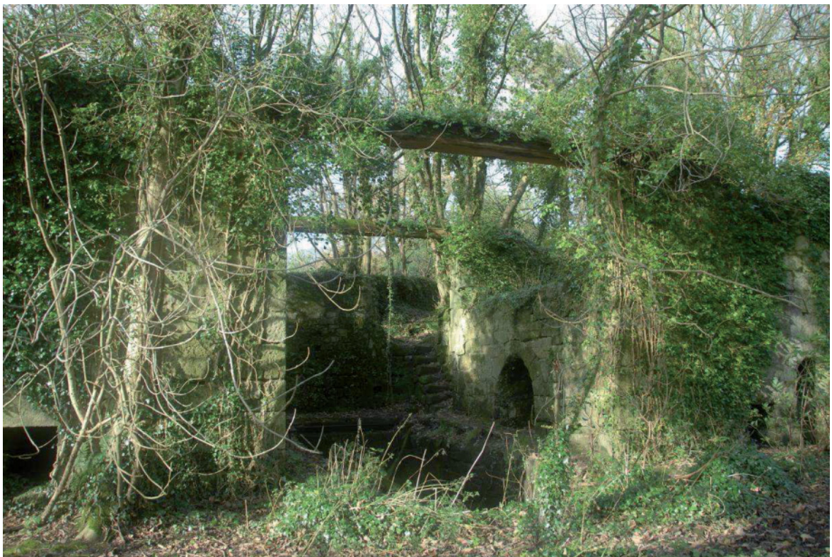
Fig 87. The central wheelpit at Mica Mill [39] seen from the east. The surviving spanning timbers can be seen in this view. HE Digital Image Archive.
