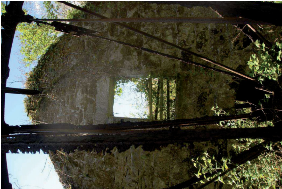
Fig 70. The southern side of the wheelpit at Big Wheel Mill. The water wheel spokes in the foreground demonstrate the need for very urgent remedial works. HE Digital Image Archive.
