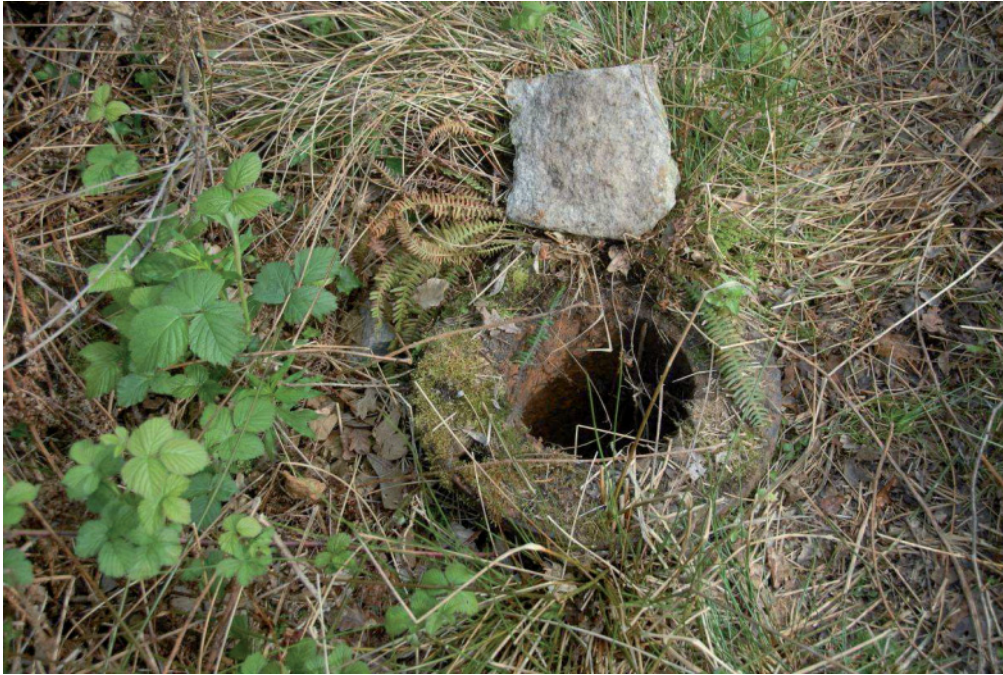
Fig 38. The top of the cast iron rising main adjacent to the pumping shaft [8] at Wheal Arthur mill. HE Digital Image Archive.
