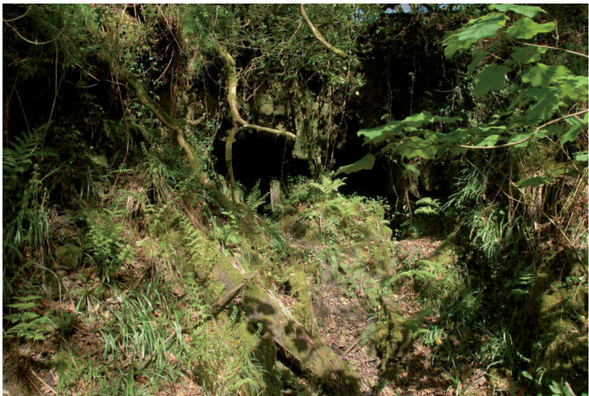
Fig 55. The partially-collapsed entrance to the adit [18] leading into Rescrowsa china clay pit. HE Digital Image Archive.
