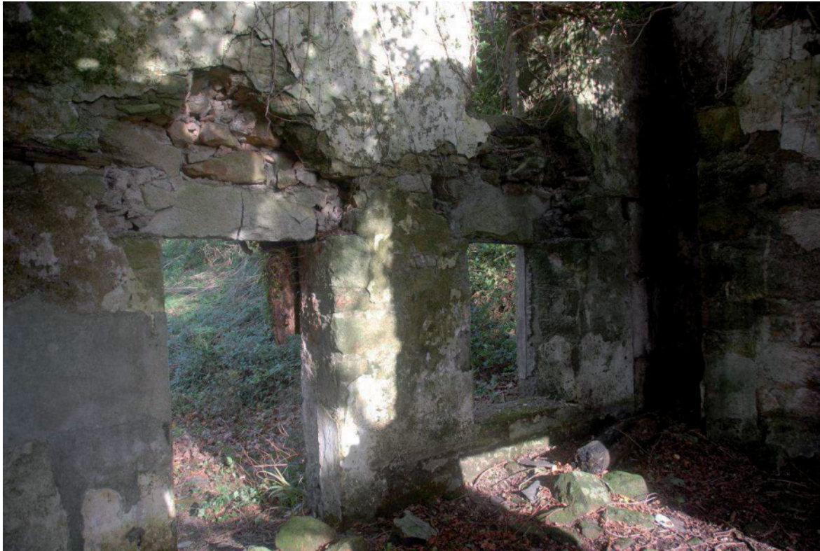
Fig 80. The internal face of the northern wall of Trevear Miller's Cottage [35], showing the surviving lime-washed plaster, but also the cracked granite lintels and lost masonry. HE Digital Image Archive.
