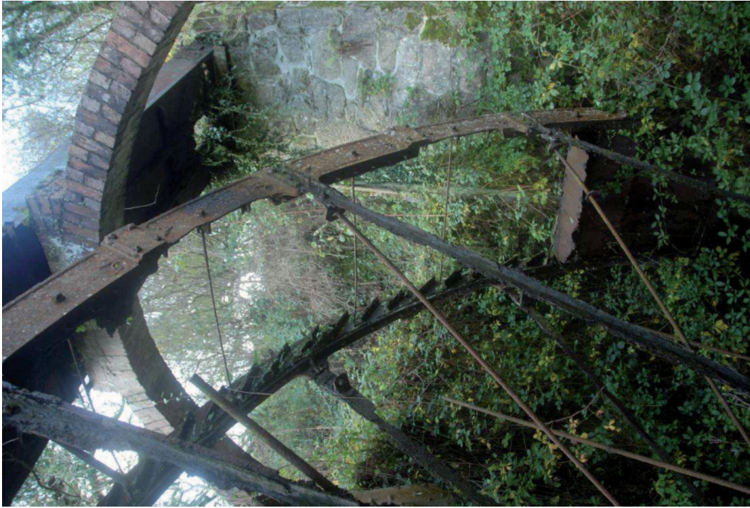
Fig 69. The western end of the central water wheel at Big Wheel Mill, showing the almost complete loss of the buckets and very poor states of the iron spokes. HE Digital Image Archive.
