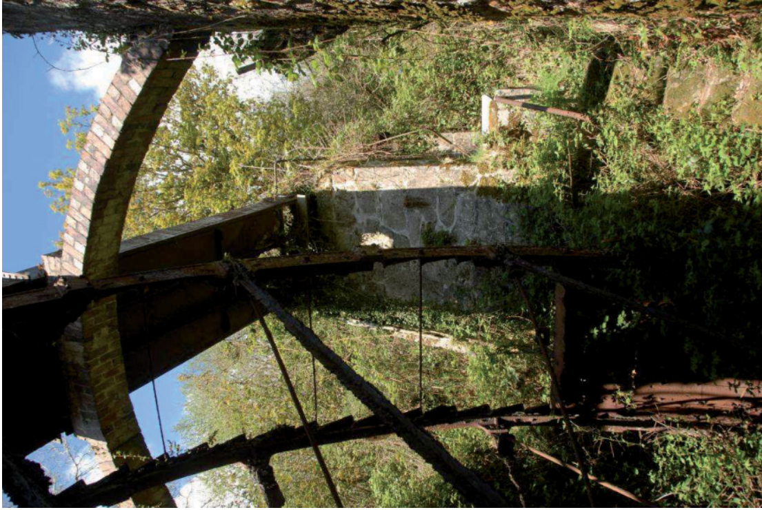
Fig 71. The western end of the wheelpit at Big Wheel Mill, showing the laundry support and the very poor state of the water wheel. HE Digital Image Archive.
