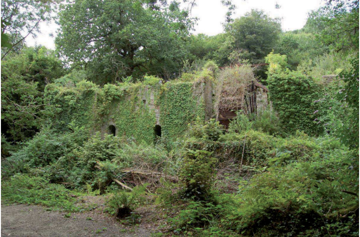
Fig 58. Big Wheel Mill [29] from the east showing the vegetation growing over and adjacent to it. HE Digital Image Archive.
