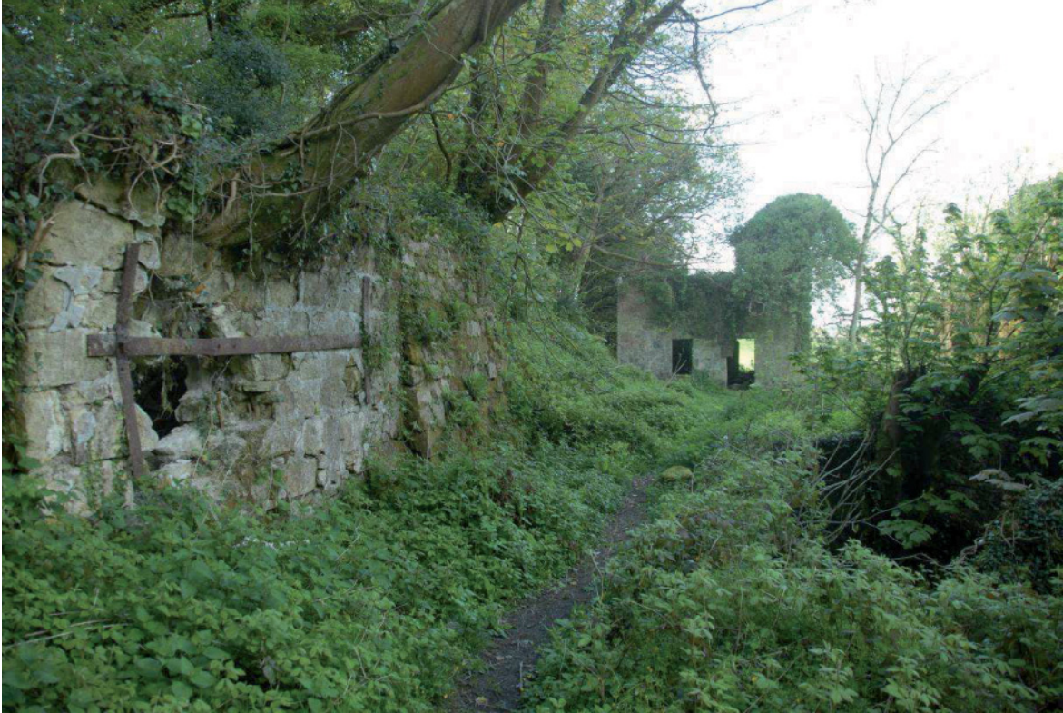
Fig 76. Trees growing out of the stonework of the Trevear Mill reservoir [33] are already causing significant damage to it. Their collapse would also damage Trevear Mill immediately to the right. HE Digital Image Archive.
