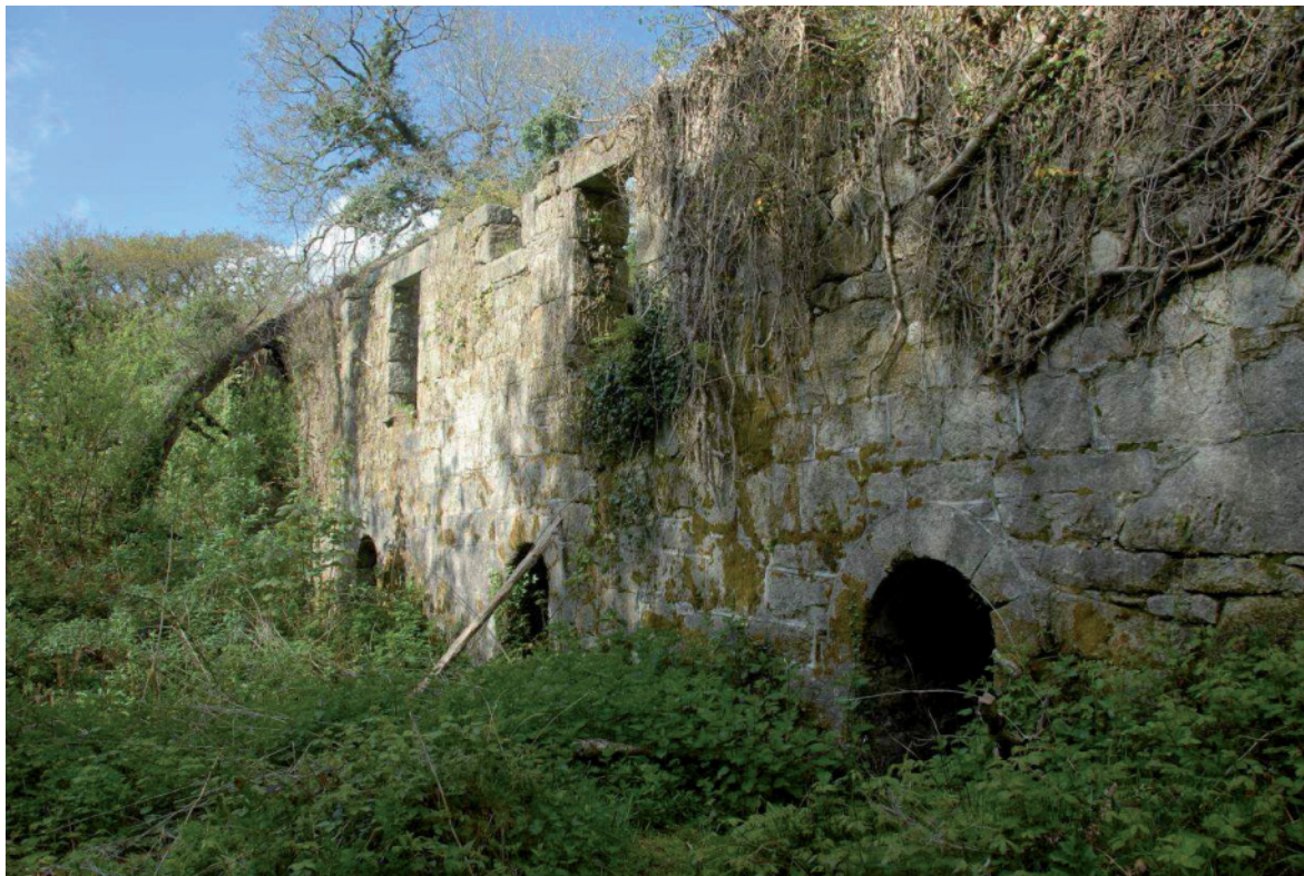
Fig 57. Big Wheel Mill [29] from the north-east, showing the overgrown water wheel and the eastern face of the building, partly cleared of ivy growth. HE Digital Image Archive.
