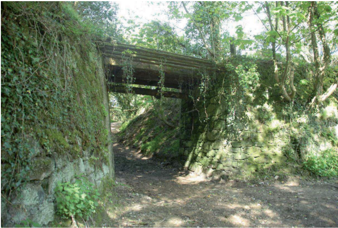
Fig 84. The tramway bridge/aqueduct [38] immediately to the north of Mica Mill which carried leat [36] seen from the south-east. A more recent pipeline runs under the bridge. HE Digital Image Archive.
