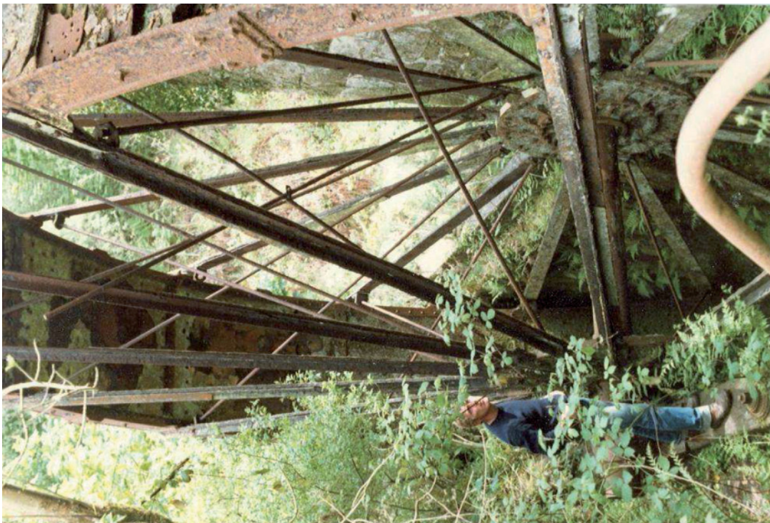
Fig 68. The report author inspecting Big Wheel Mill water wheel circa 1985. HE Digital Image Archive.
