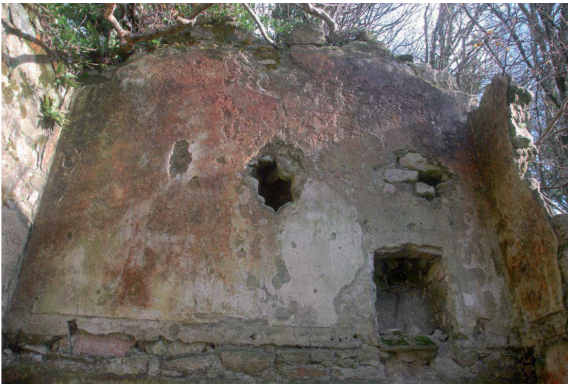
Fig 81. The interior of the upper floor on the eastern wall of Trevear Miller's Cottage, showing the surviving plaster and the aperture for the bedroom fireplace. HE Digital Image Archive.
