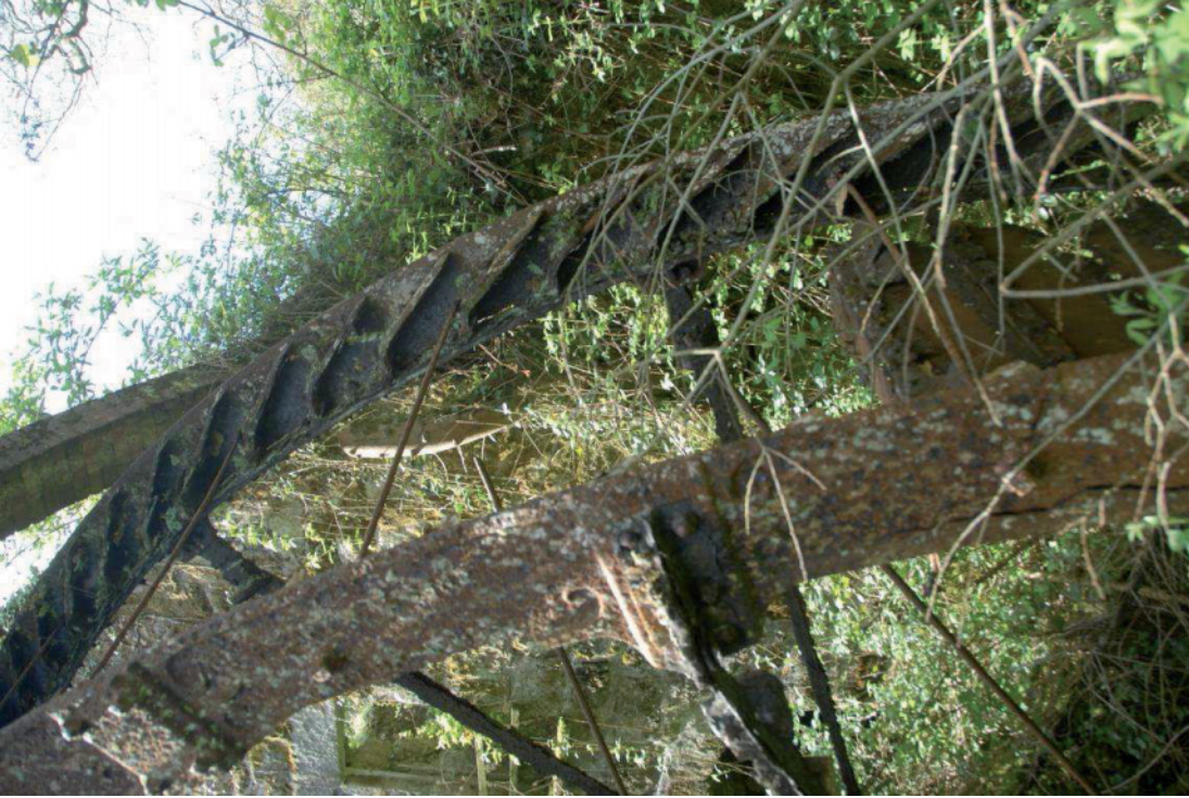
Fig 73. The now poorly-supported cast iron shrouds (rims) of the water wheel, increasingly at risk of severe damage through the likely collapse of the wheel. HE Digital Image Archive.
