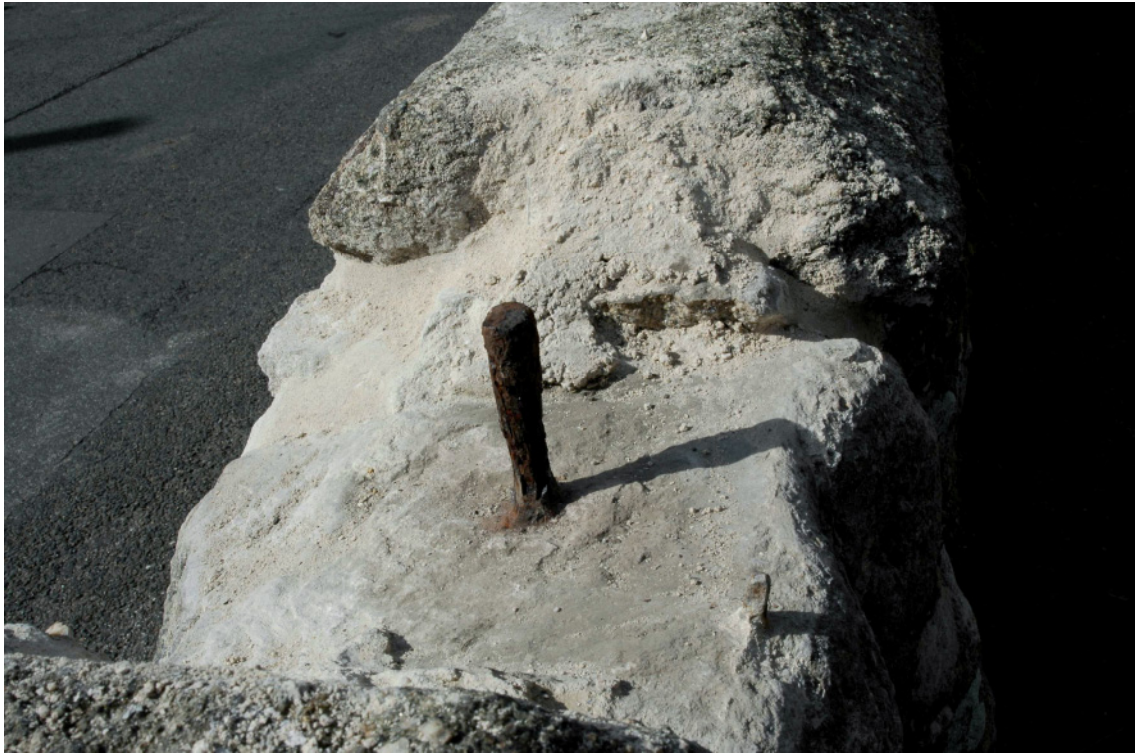
Fig 20 The rusted iron pin
