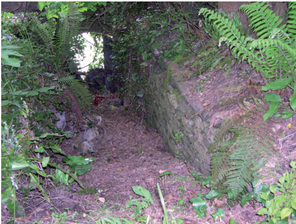
Fig 18 View down the steps to the arched Congregationalist doorway, one of the original features potentially offering rich experiences of aspects of past lives, but now disused, ruinous, unstable and possibly dangerous
