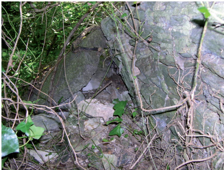
Fig 15 The boundary on the east of the Congregationalist cemetery south of its centre, showing instability, bulging and partial collapse of the walling and its granite coping, with tree and ivy growth
