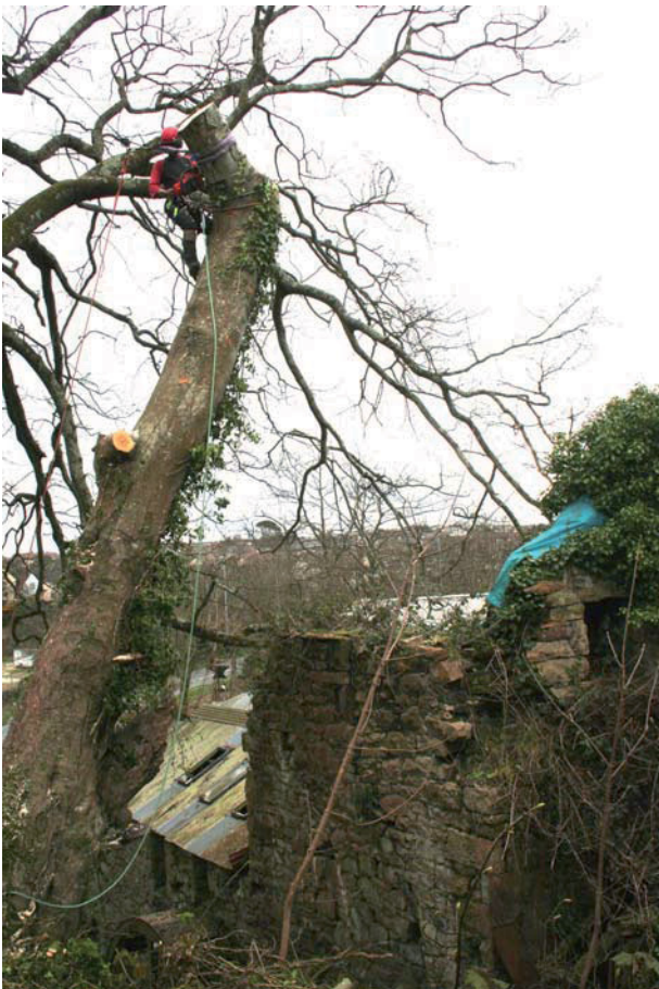
Fig 4: Extreme care was taken due to the proximity of the tree to the foundry building
