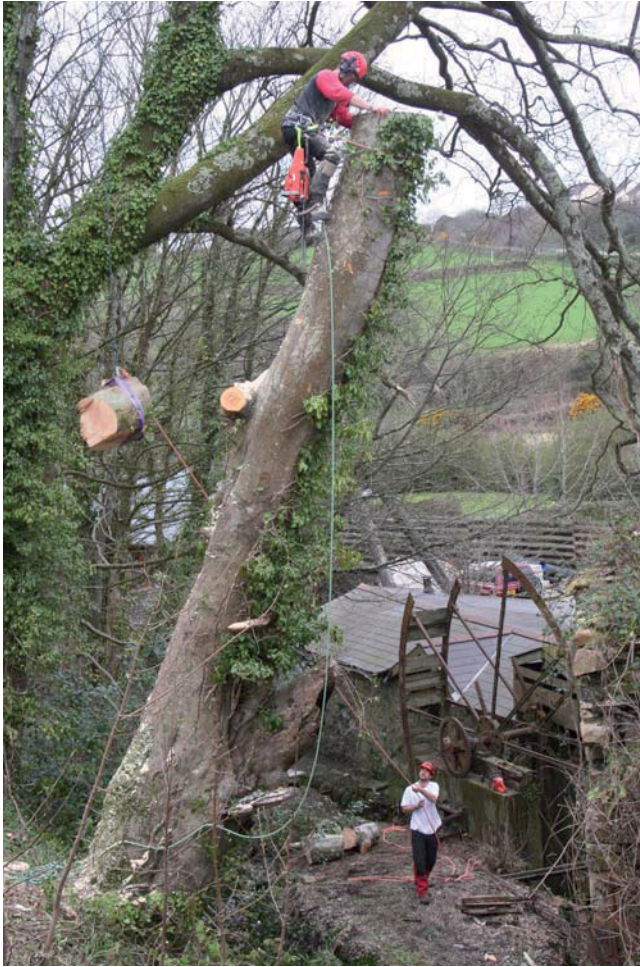
Fig 5: As felling progressed sections were lowered onto the flat area adjacent to the mill leat.
