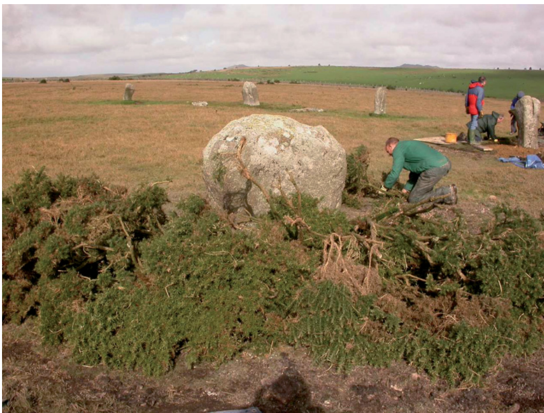
Fig 7. Gorse is tied around the repaired stones to protect the freshly-laid turf from livestock.
