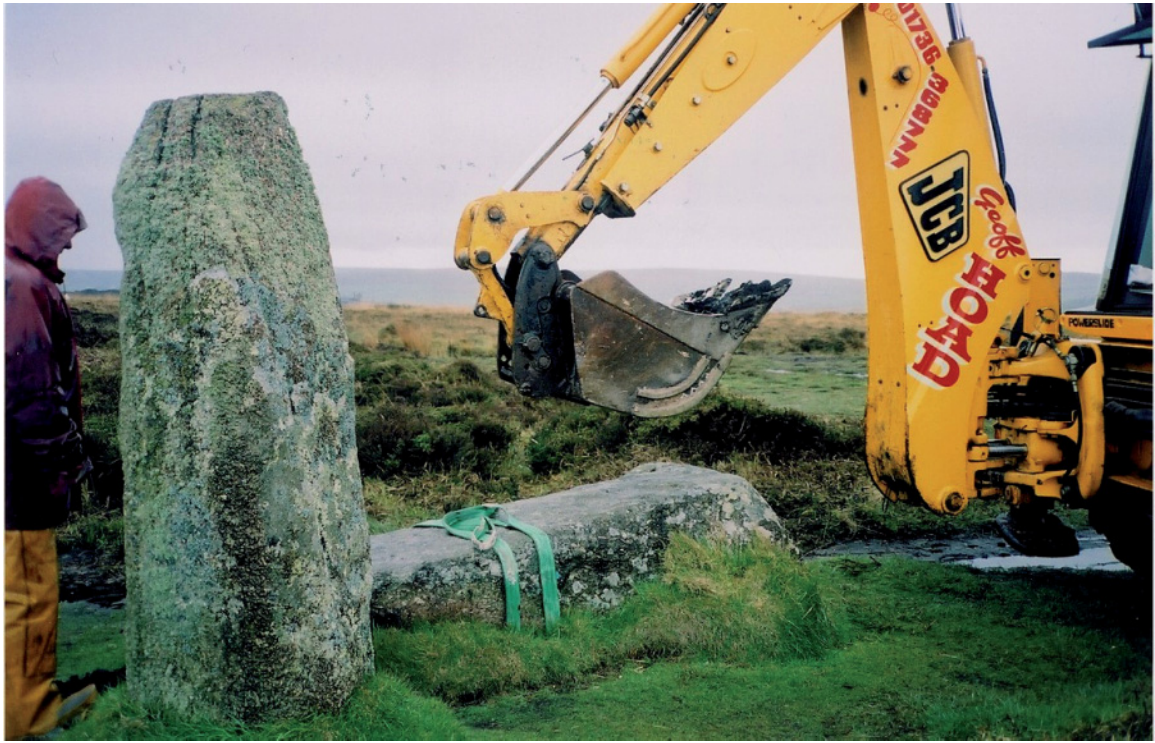
Fig 15 lifting aside a fallen stone prior to excavation to locate the stone's socket
