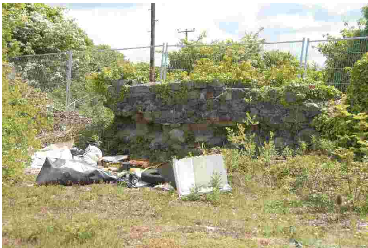
Fig 45. The eastern boundary wall of the former sawmill, constructed from a mixture of masonry and brickwork. This area next to an adjacent land is particularly prone to fly tipping.
