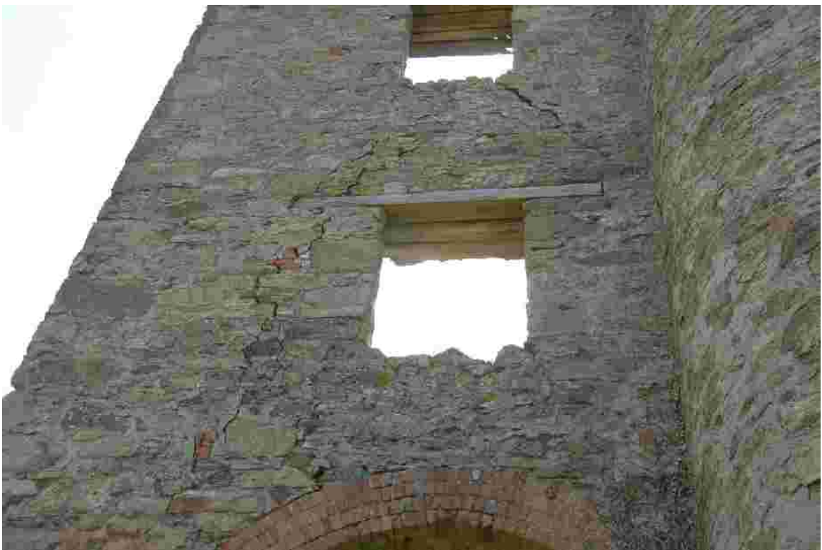
Fig 42. Failure cracking in the rear elevation of Read pumping engine house needs to be addressed soon if major parts of this wall are not to collapse.
