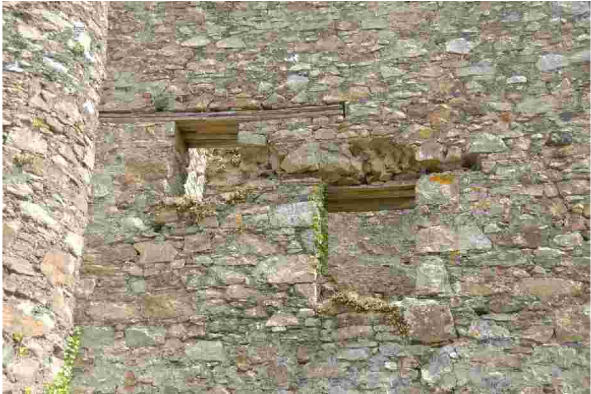
Fig 41. The decay of timber lintels on the south-western elevation of Reade's pumping engine house has resulted in the loss of masonry in the walling above.
