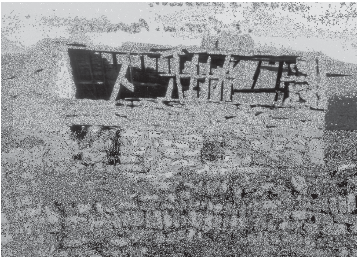
Fig 9. A view of the Chapel from the west, again probably taken during the early 1960s showing the severe deterioration of the roof structure at that date. NT Collection.
