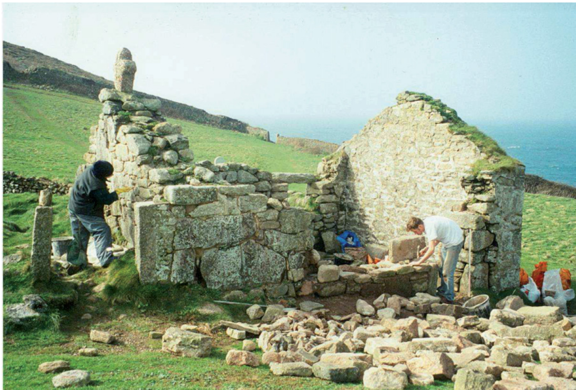
Fig 18. An early stage during the conservation works. The foundation courses of the collapsed walling have been reconstructed, whilst repointing is under way on the southern wall. HE Digital Image Archive.
