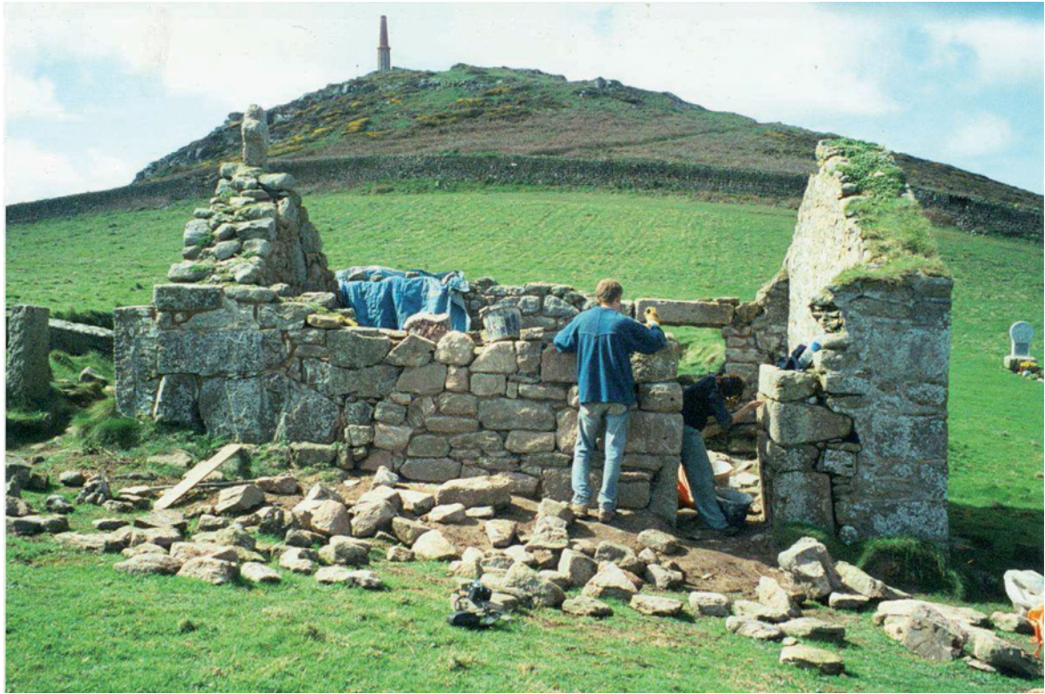
Fig 20. The reconstruction of the collapsed section of the eastern wall approaching completion. HE Digital Image Archive.
