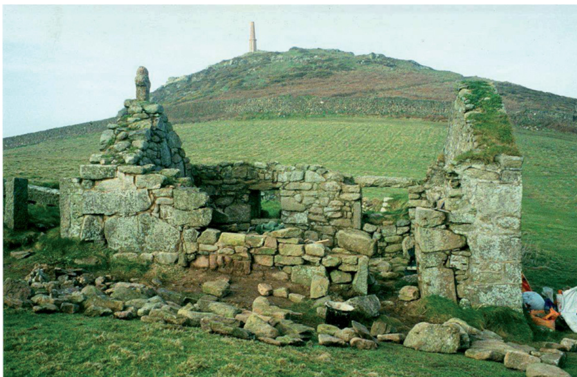
Fig 19. A later stage during the reconstruction of the eastern wall and doorway reveal. HE Digital Image Archive.
