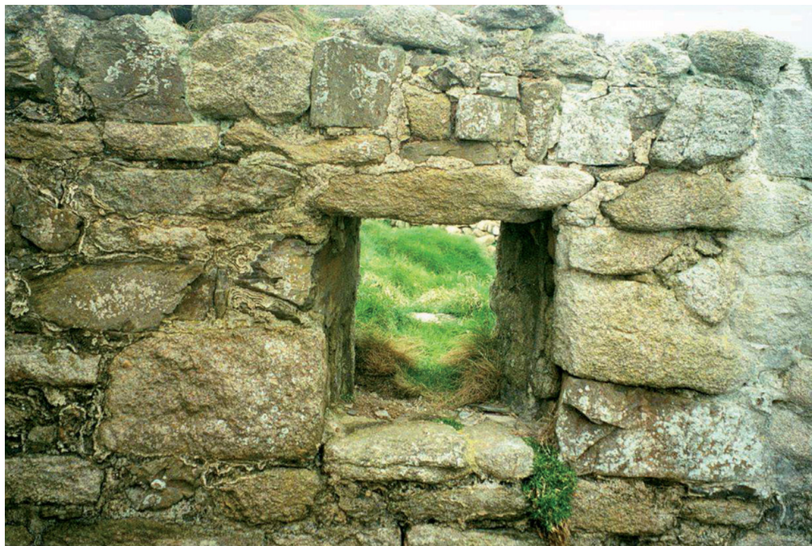
Fig 21. The masonry over the external face of the window in the western wall. HE Digital Image Archive.
