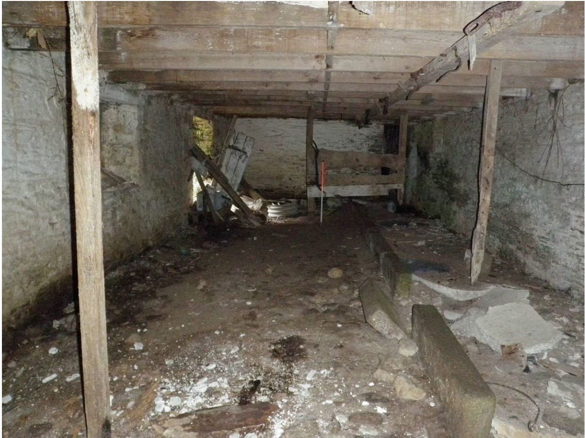
Fig 17: Ground floor in east range (former milking parlour/cow-house) showing stalls and feeding troughs
