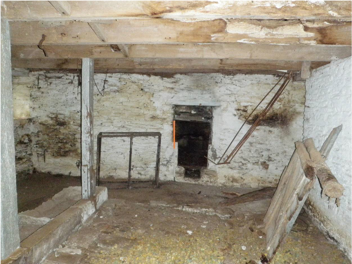
Fig 15: North-east end of ground floor in west range (former cow-house) showing machine bearing/fireplace recess
