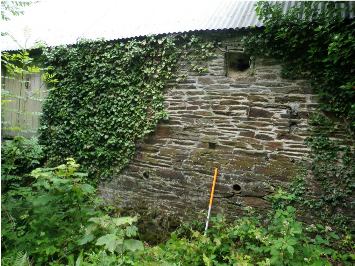
Fig 13: Section of north-east elevation of east range showing opening for horse-engine drive shaft
