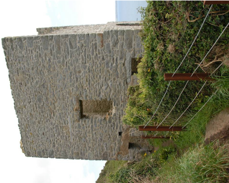
Fig 38. The conserved engine house and new safety fencing at New Engine Shaft seen from near the whim plat serving this shaft.
