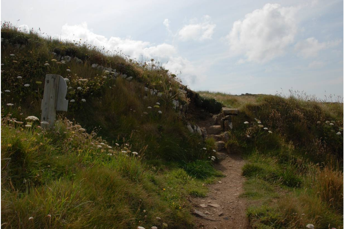
Fig 58. The boundary wall between Rinsey East Cliff and Trewavas. Path erosion on the thin cliffslope soils is a minor problem. Note also the damage to the wall where the path crosses it. This stile should be repaired.
