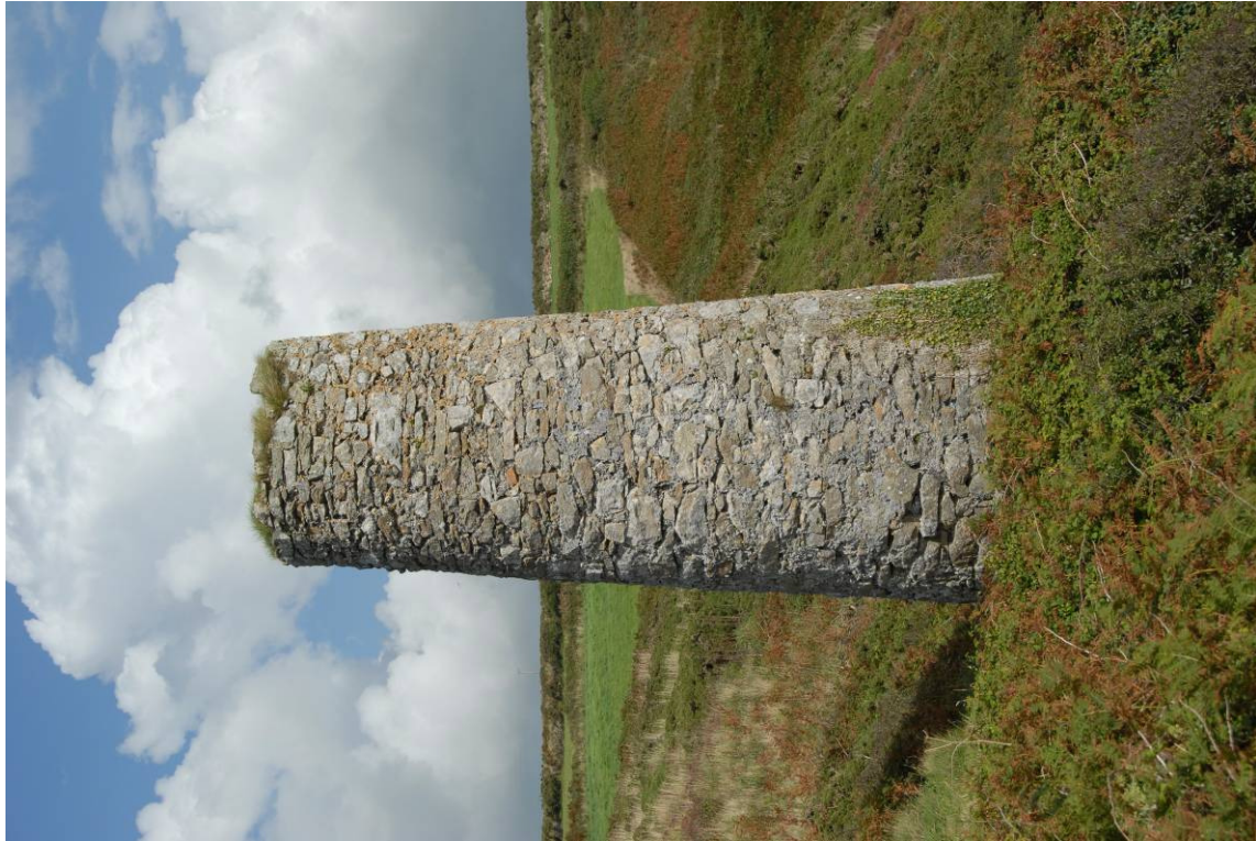
Fig 32. The clifftop chimney which served the boilers at Old Engine Shaft via a flue running up the cliffside.
