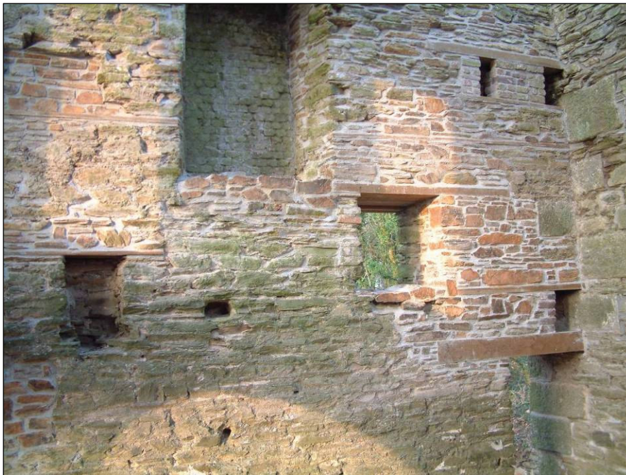
Fig 4 Internal view of Hitchen's engine house (after works) C Buck 2001 © CC CAU
