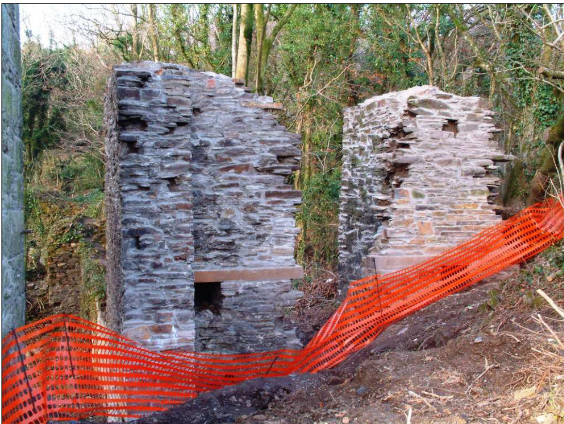
Fig 11 View of the balance bob east wall (after works) C Buck 2001 © CC CAU
