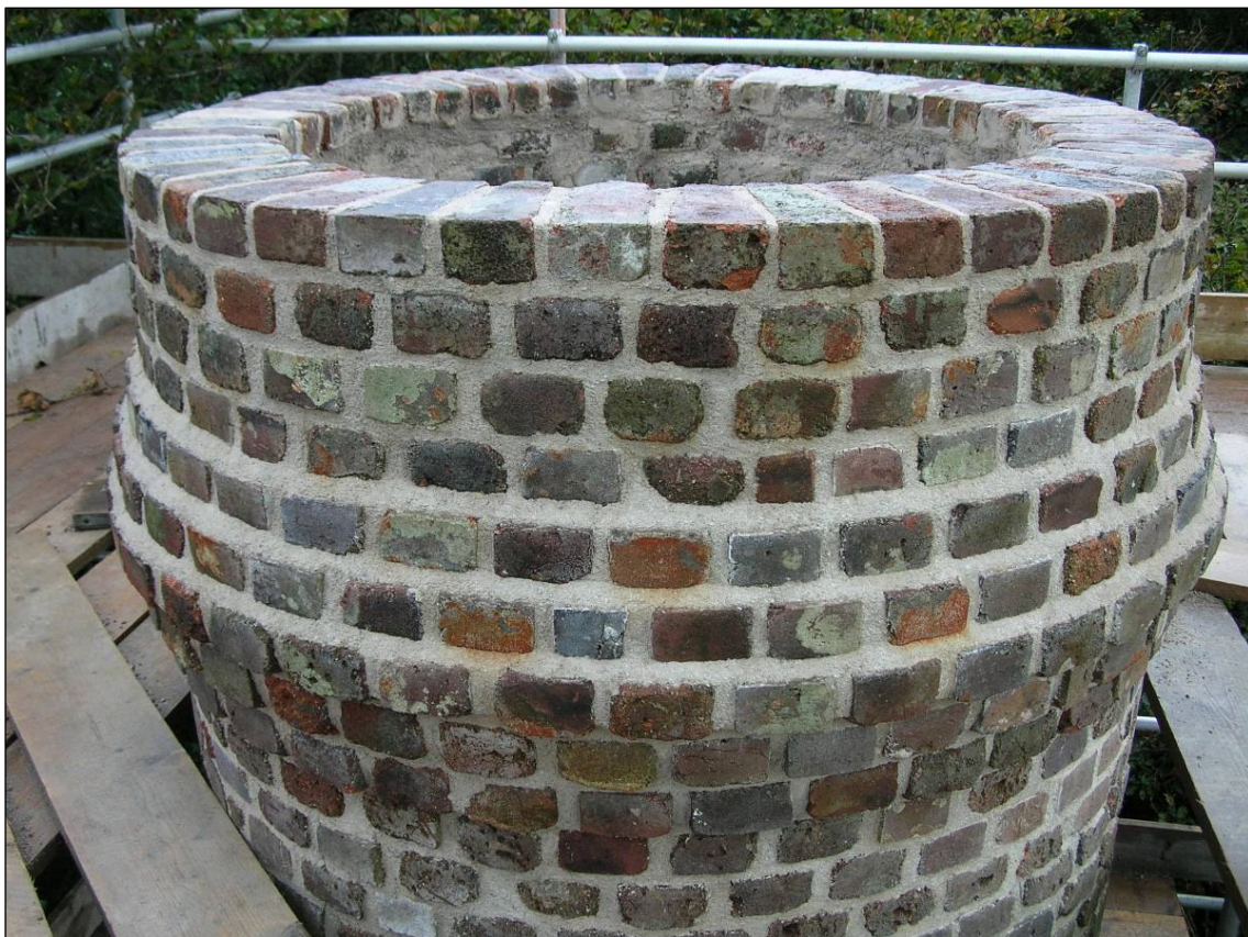
Fig 30 View of the top of the chimney (after works) C Buck 2008 © CC HE Projects
