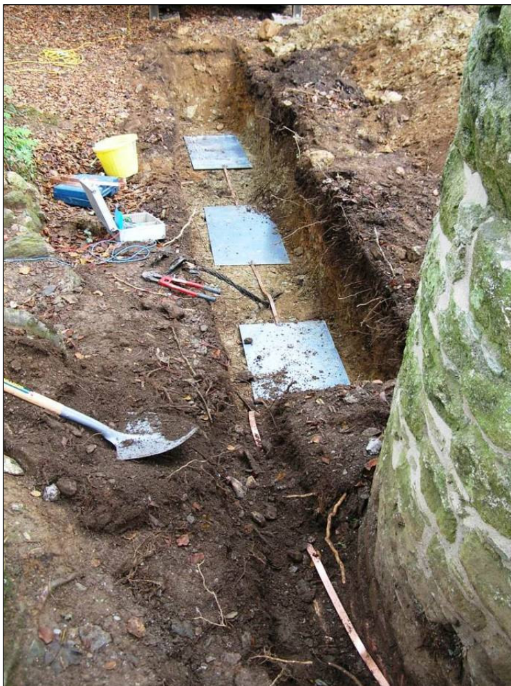
Fig 31 View of the lightning conductor earth plates (during works) C Buck 2008 © CC HE Projects
