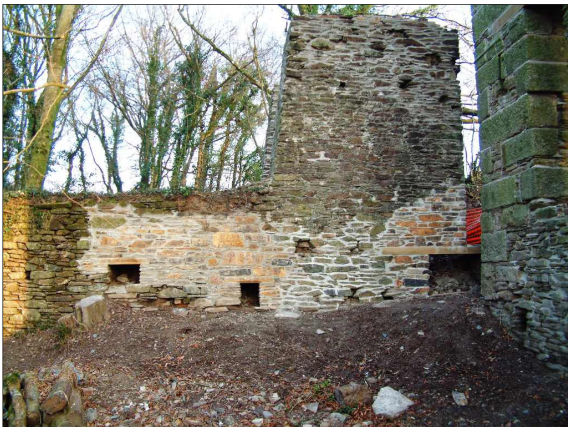
Fig 9 View of the boiler house north wall (after works) C Buck 2001 © CC CAU
