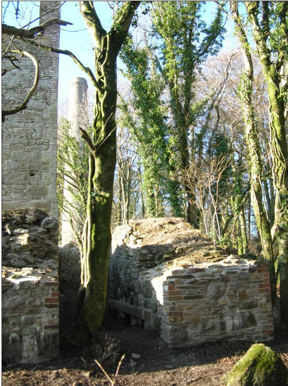
Fig 26 View of the winding engine house winder drum loadings (after works) C Buck 2008 © CC HE Projects
