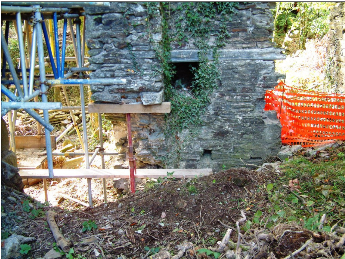
Fig 10 View of the balance bob east wall (before works) C Buck 2001 © CC CAU
