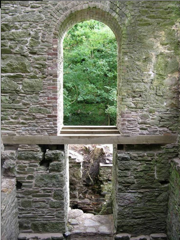
Fig 22 Internal view of the winding engine house east (bob) wall after works C Buck 2007 © CC HE Projects
