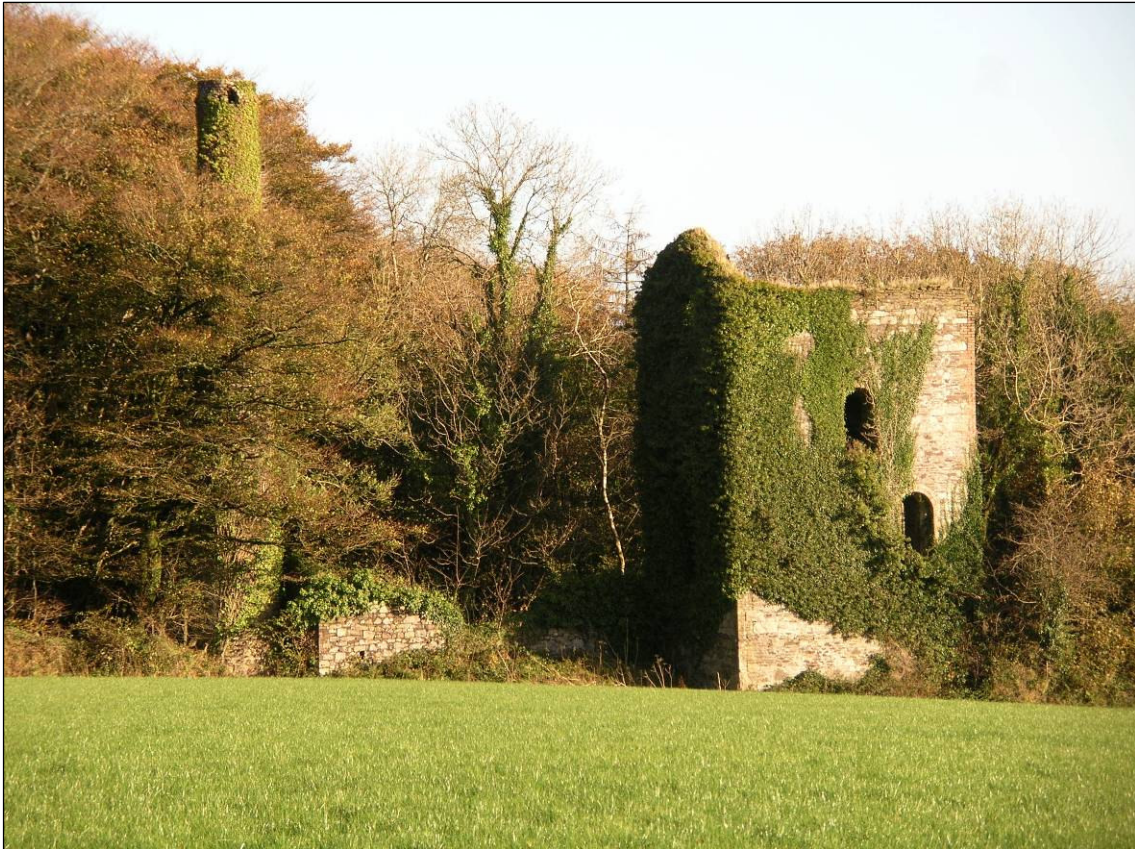
Fig 24 View of the south side of the winding engine house (before works) C Buck 2007 © CC HE Projects
