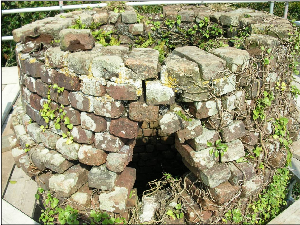
Fig 29 View of the top of the chimney (before works) C Buck 2008 © CC HE Projects
