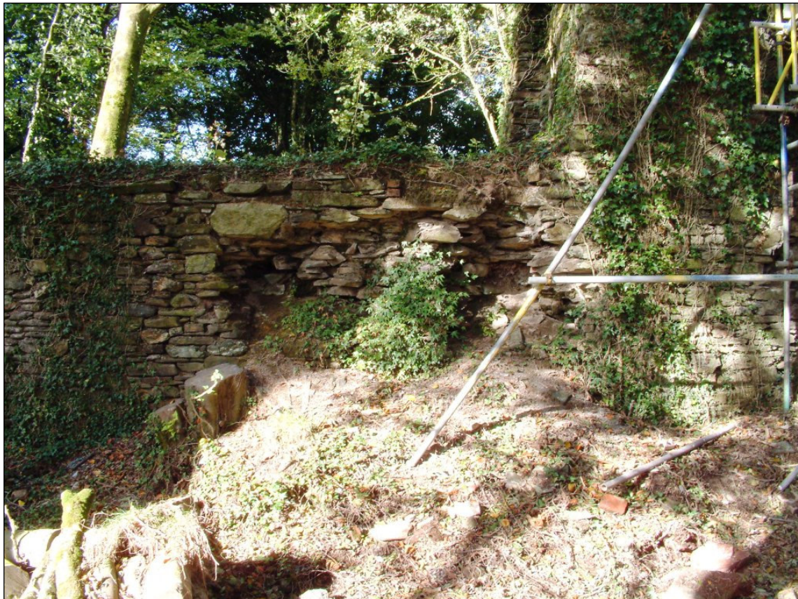
Fig 8 View of the boiler house north wall (before works) C Buck 2001 © CC CAU
