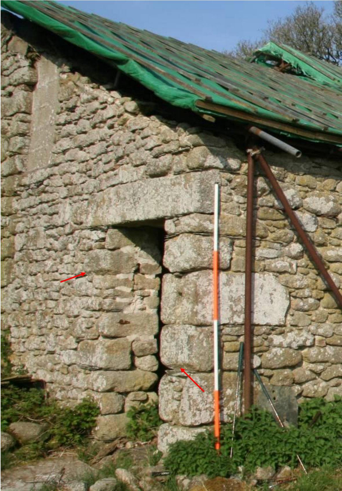
Fig 16 The later 19 th century lean-to, showing chamfered stones reused in the jamb masonry (arrowed).
