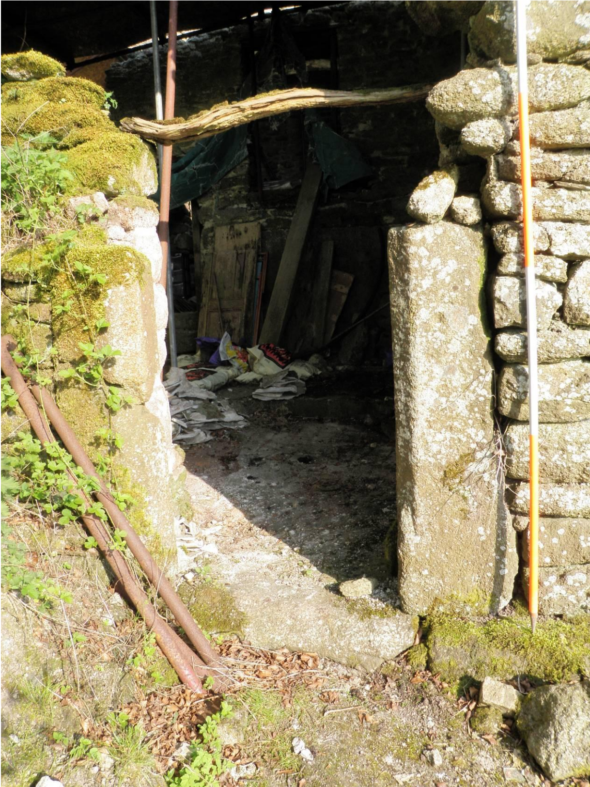
Fig 14 Detail of the present remains of the doorway. Note the remains of the timber inner lintel.
