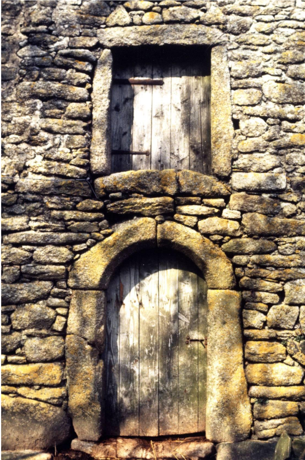
Fig 12 Detail of the lower end arched doorway and upper floor opening in 1981 (Photograph, copied from a slide, kindly supplied by Jacky Nowakowski).
