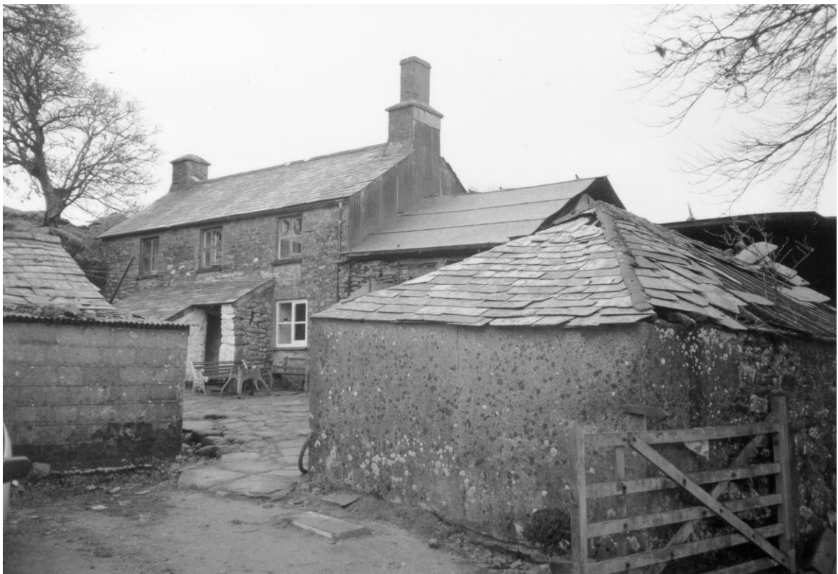
Fig 7 Codda in 1999, by which time the old roof on the lower end had fallen in, and had been replaced by temporary boarding.
