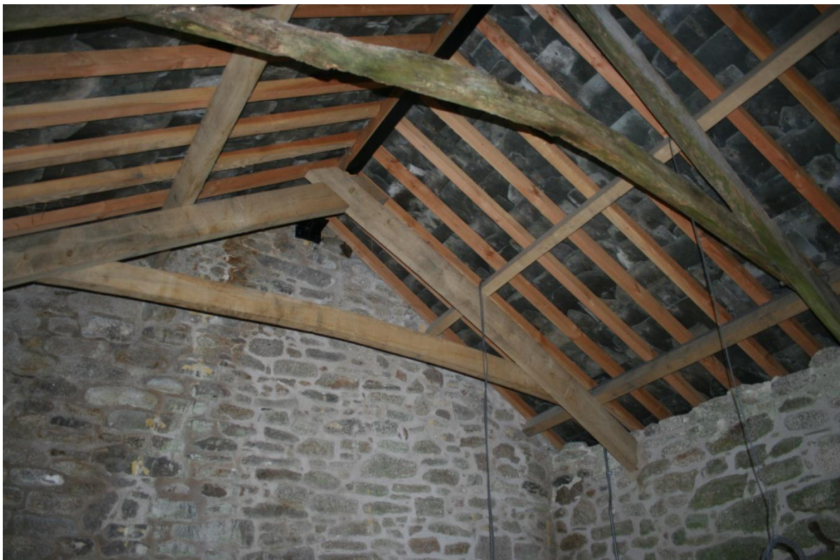
Fig 30 New roof structure above through-passage, showing earlier roof truss (in foreground) and strengthening steel purlin at apex.
