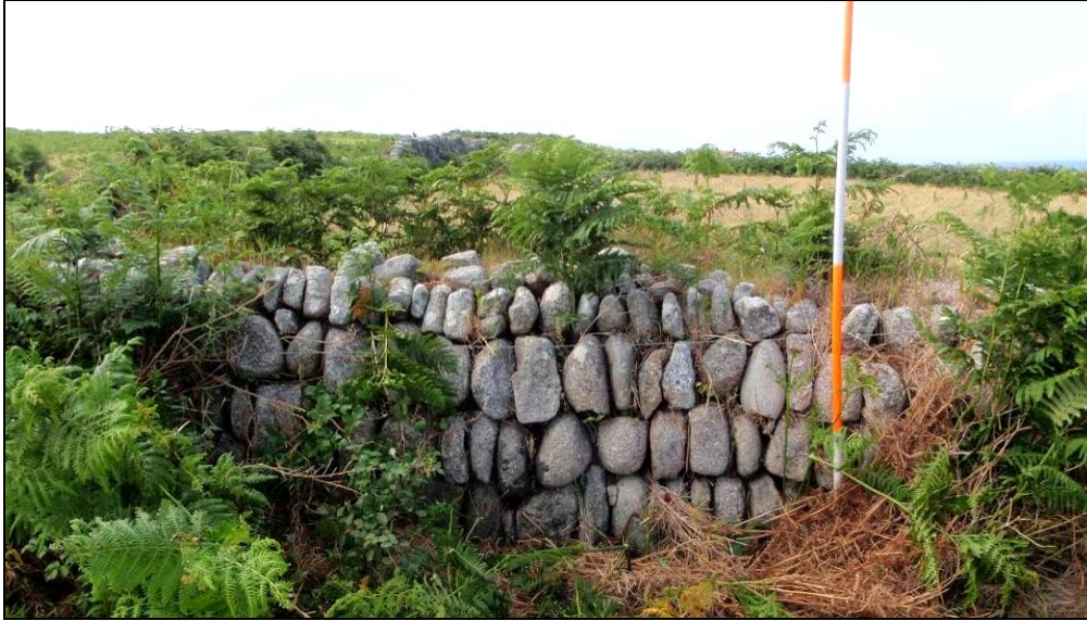
Fig 28 Boundary 66 in St Martin's 2a: a stone-faced earth wall of regular coursed and graded stonework; many of the stones are rounded and appear to be beach cobbles. The style is unusual within the survey area and emphasises the diversity of boundary types found in this block. (Photograph: Historic Environment, Cornwall Council.)
