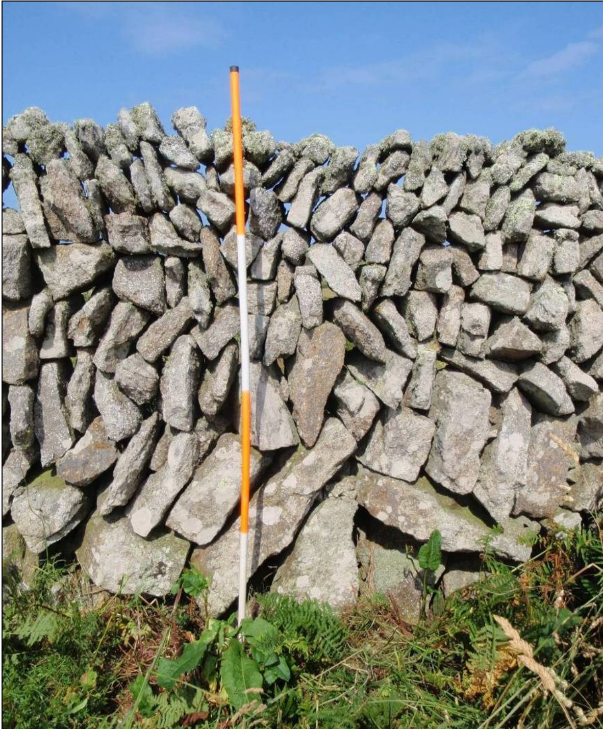
Fig 25 Dry-stone wall 55 in St Martin's 2a survey area, an example of a distinctive boundary type known to have been constructed by Sidney Bond in the 1920s (Keith Low, pers comm). These walls are based on low earth-set orthostats at approximate 2.4m intervals; one is visible just to the right of the ranging pole. (Photograph: Historic Environment, Cornwall Council.)
