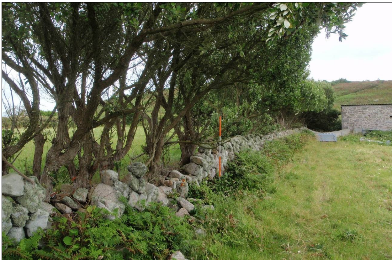
Fig 16 Dry stone wall 36 facing a low lynchet in the Bryher 3 survey area. Grown-out hedging material along the boundary is partly responsible for the instability of this and a number of other nearby boundaries. Tumble is readily apparent and repair of boundaries of this type would be relatively easily achieved. (Photograph: Historic Environment, Cornwall Council.)
