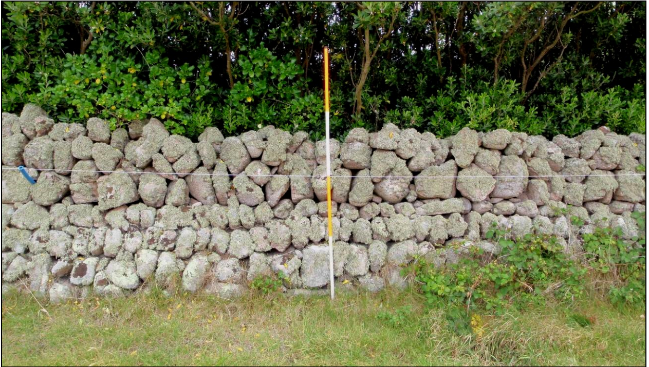
Fig 23 Stone-faced stone wall (St Agnes 2, boundary 81), probably on the line of an older boundary and re-built to shelter the vegetated 'fence' behind it when first planted, with the upper courses added subsequently in a different style. (Photograph: Historic Environment, Cornwall Council.)
