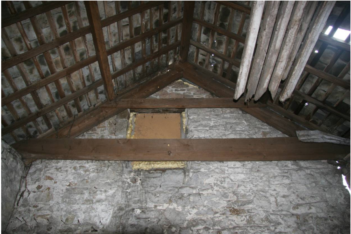
Fig 12 Gable of neighbouring building at west end, abutted by the subject outbuilding The window would have lit the loft of this structure before the later building adjoined it
