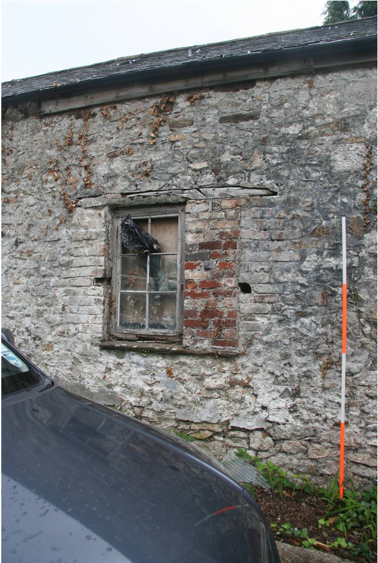
Fig 10 Partially blocked window in south wall
