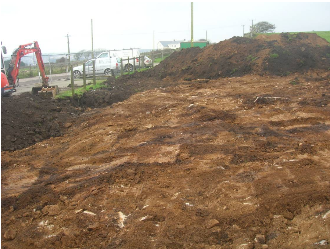
Fig 8 General view of site at end of topsoil stripping showing nature of the ground encountered, looking to the northeast.
