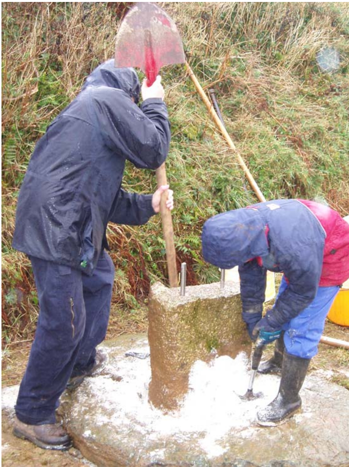
Fig 13 The restoration of the lower part of the shaft: : above, the shaft (note the stainless steel pins) is put into place and below, the shaft is mortared into the base by Reuben Butts and Tommy Rose-Jones
