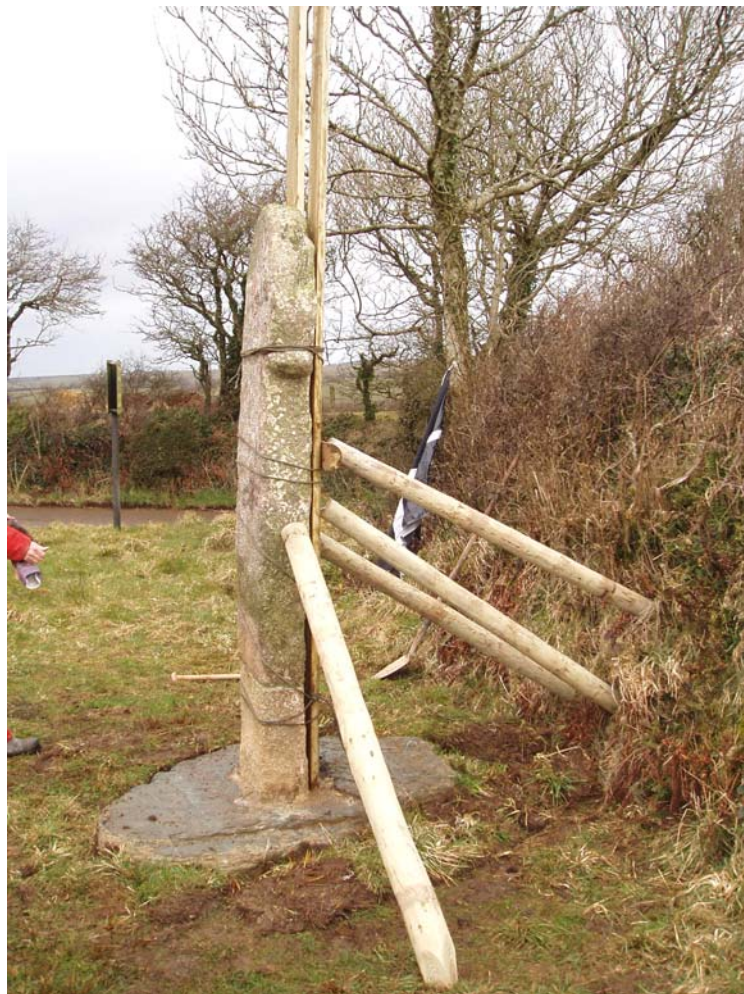
Fig 14 The restoration of the upper part of the cross.: above left, lifting the cross onto the lorry to take it to the site; above right, the two halves of the cross united and below, the restored cross, braced to prevent the new joint from moving in the wind.
