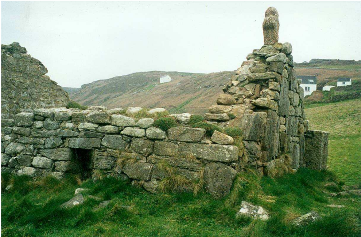
Fig 12. St. Helen's Chapel from the west-south-west before works, showing the window, the smaller size of masonry used in this wall and the deterioration of the southern wall head. HE Digital Image Archive.
