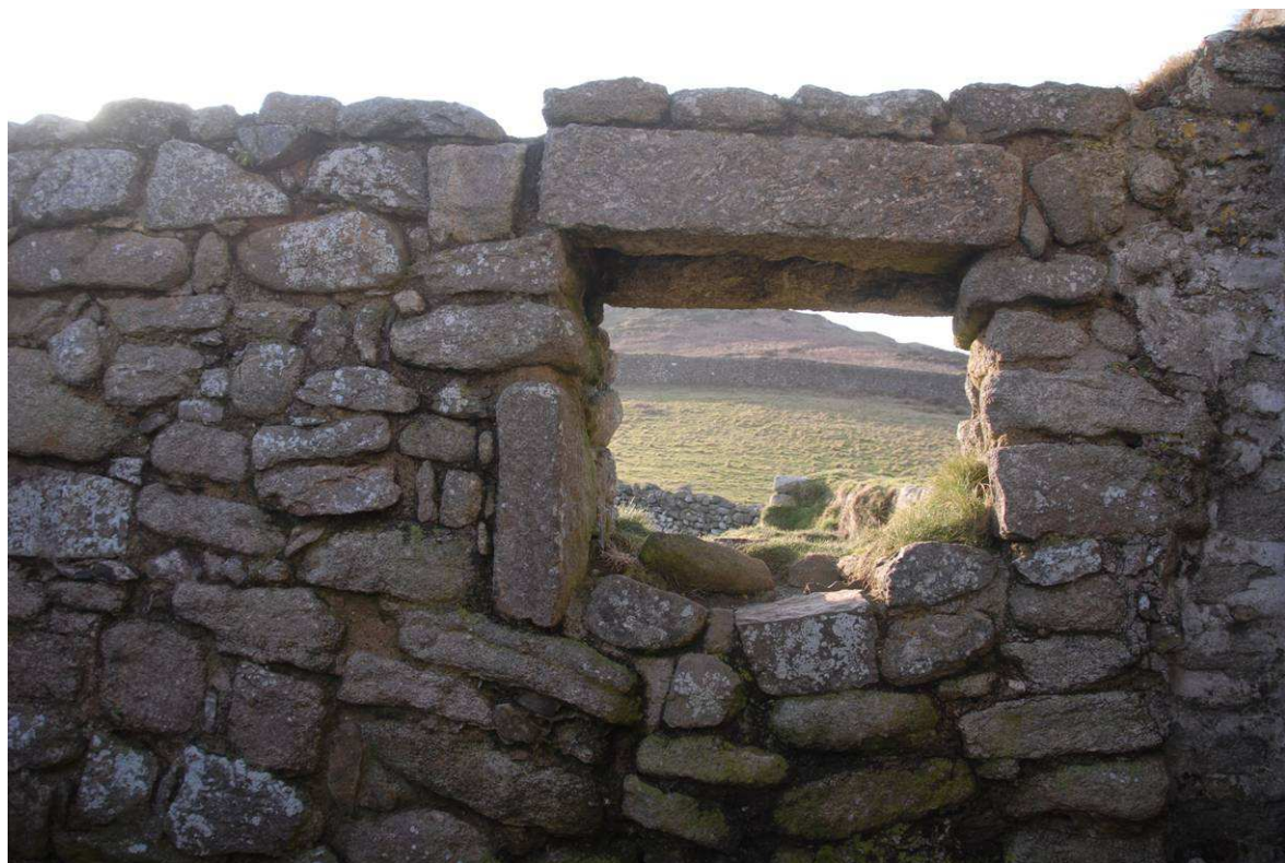
Fig 27. The internal elevation of the small window in the western wall of St. Helen's Chapel in late 2009. HE Digital Image Archive.
