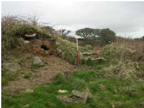
Figure 10, looking eastwards to the damage to the rampart on the south western corner of the enclosure. Note the low walling which may date to the 19 th century and the exposed rab infill of the rampart.
