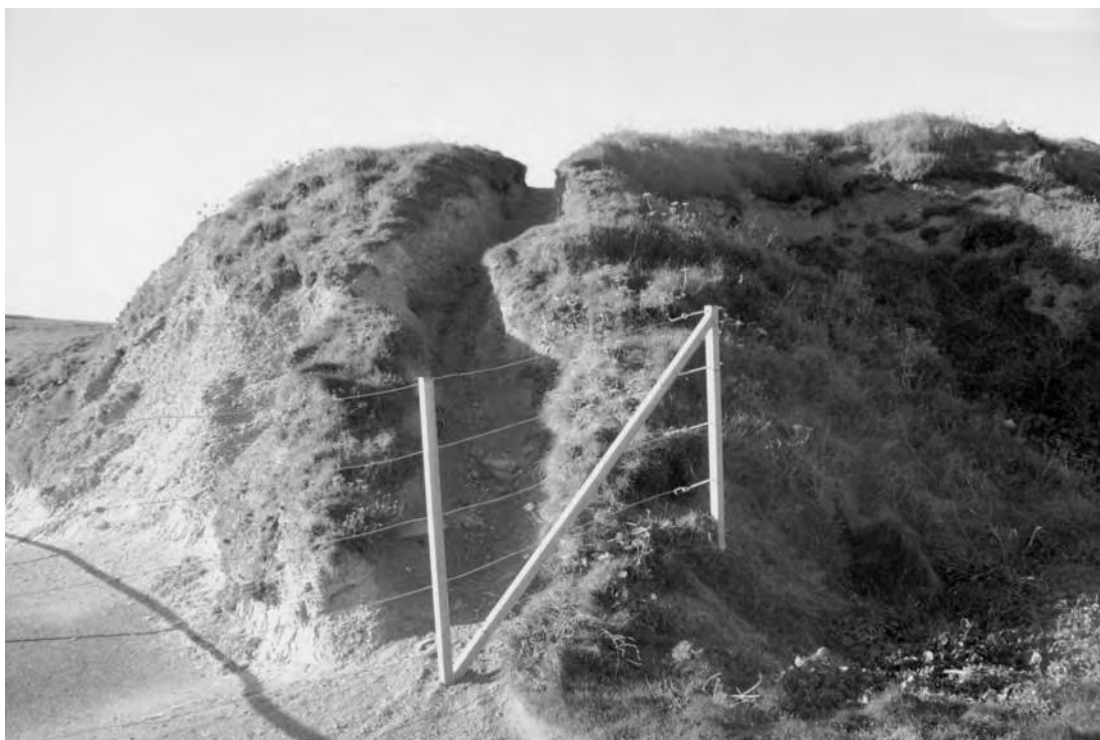
Figs. 16 Eroded scar across rampart 4, prior to works commencing. Photograph taken from the east.
