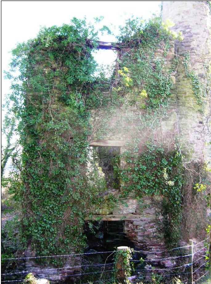
Figure 5 External north view of the rotary engine house before works © CC HE Projects 2008
