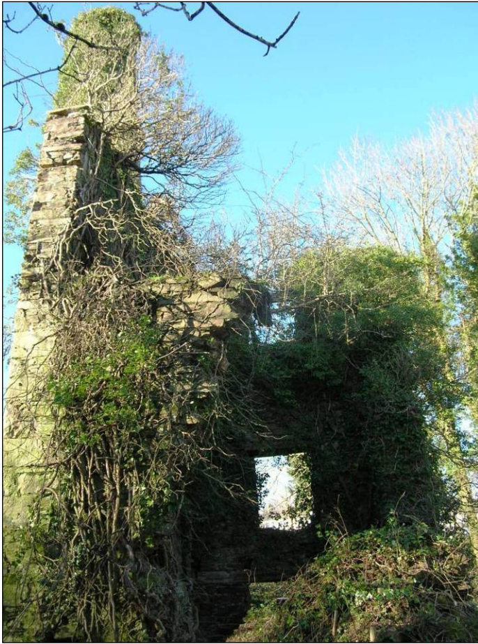
Figure 8 External south view of the rotary engine house before works © CC HE Projects 2008
