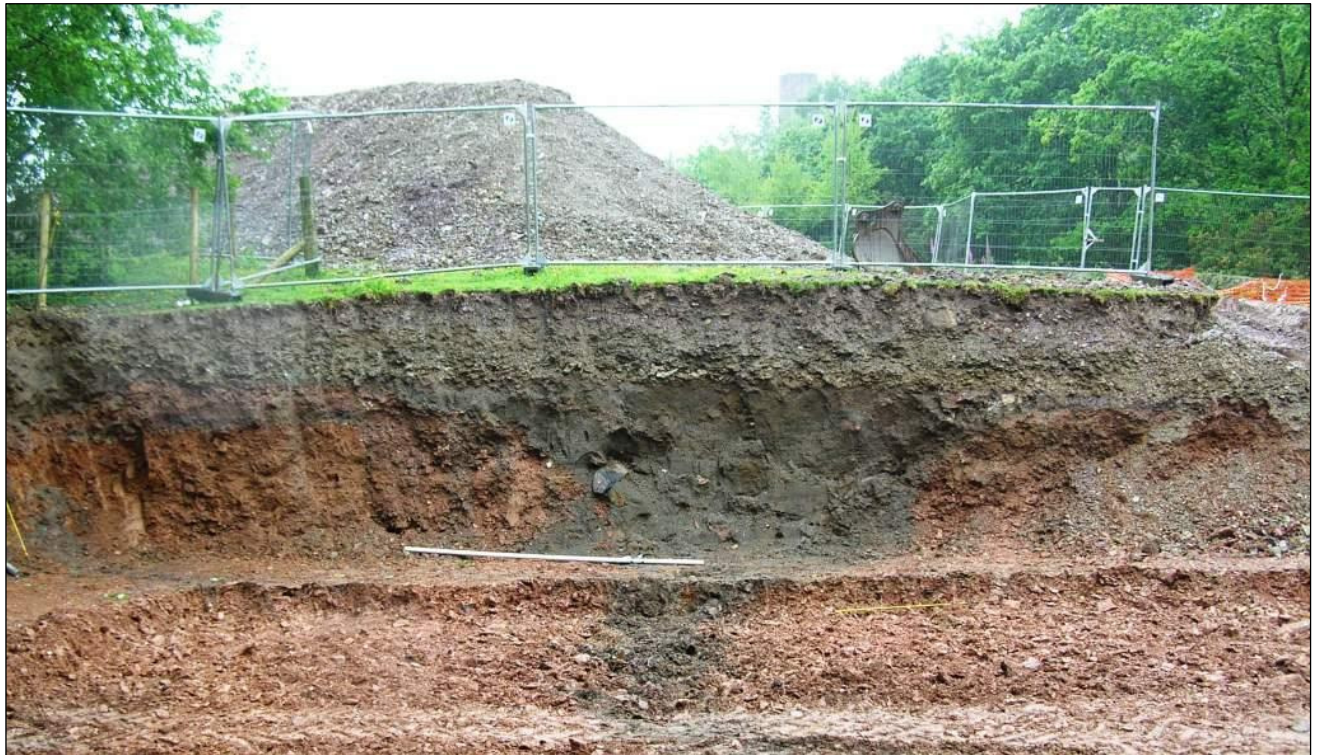
Figure 18 A view (south end) of Section A-A' from the east © CC HE Projects 2008
