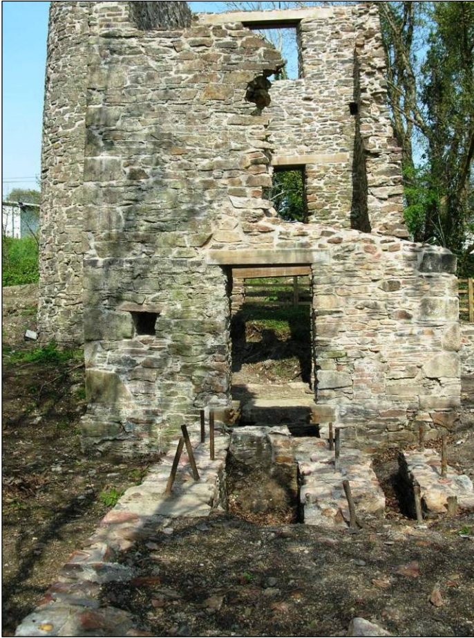
Figure 12 External south view of the flywheel loadings/crank pit after works © CC HE Projects 2008
