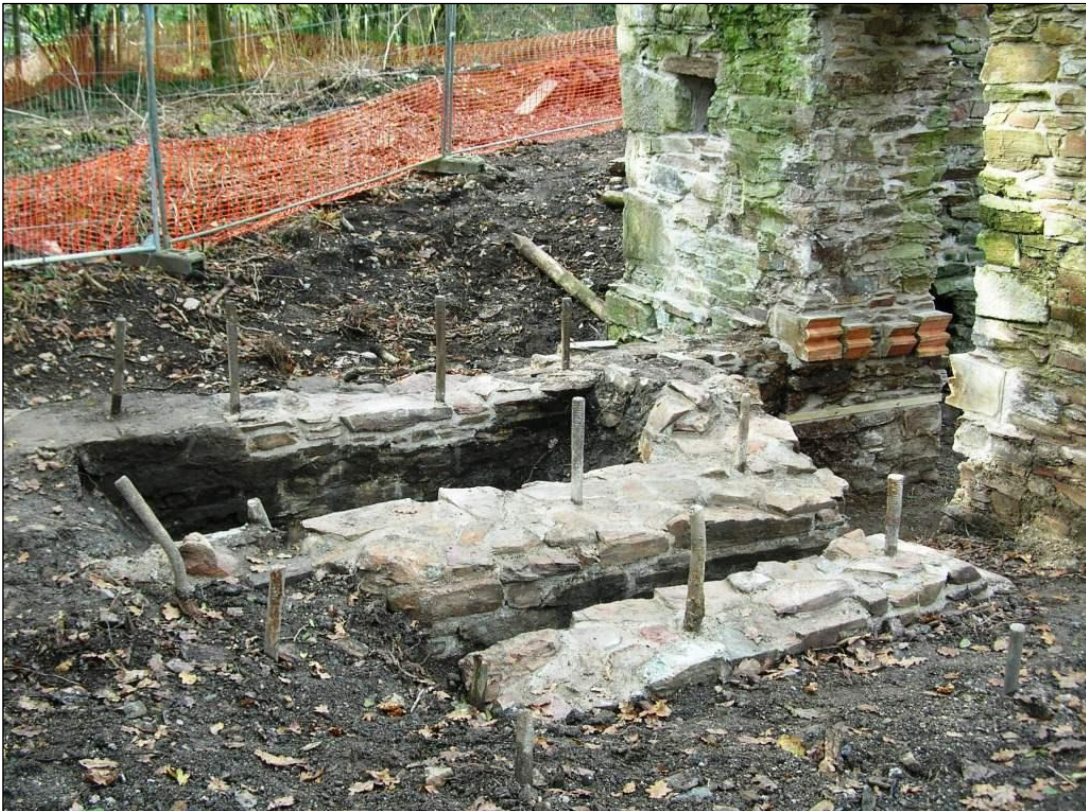
Figure 13 External east view of the flywheel loadings/crank pit after works © CC HE Projects 2008
