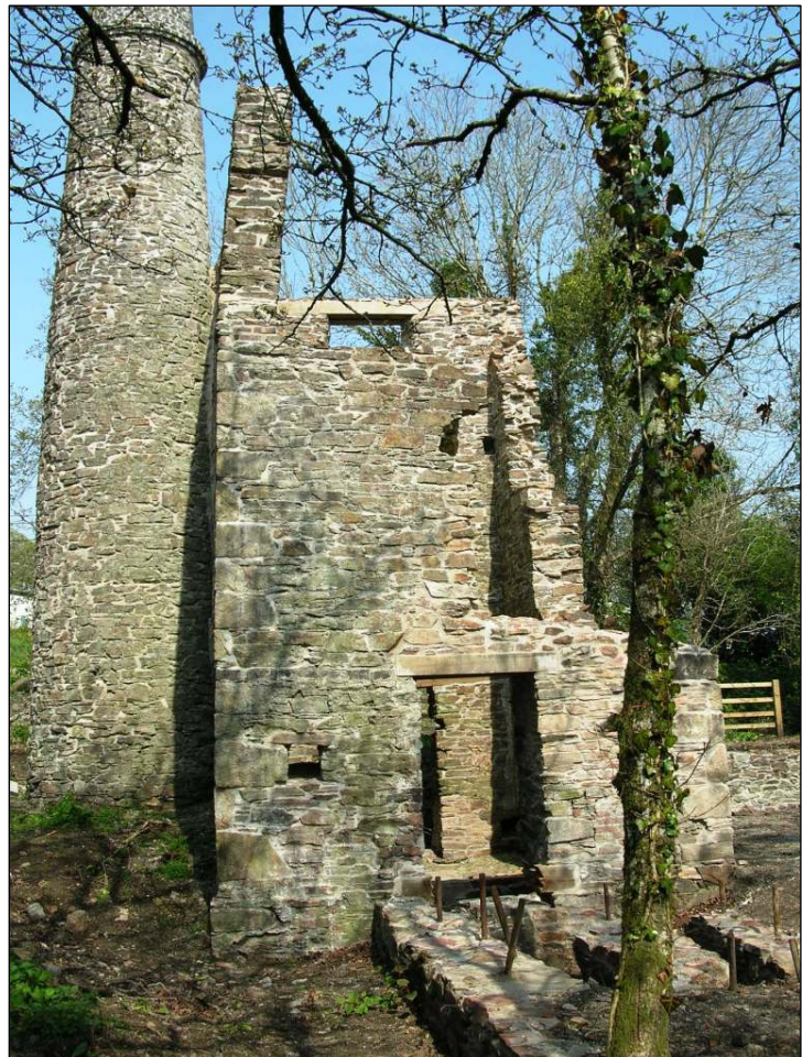
Figure 9 External south view of the rotary engine house after works © CC HE Projects 2008
