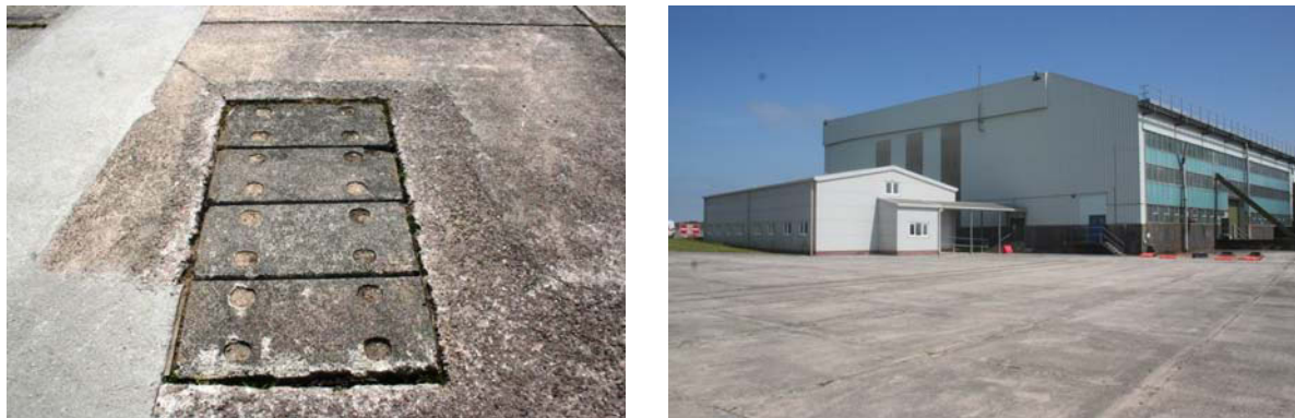
Fig 22 Detail: Concrete cover in apron allowing access to service duct (left) and new office block *43 (right)
