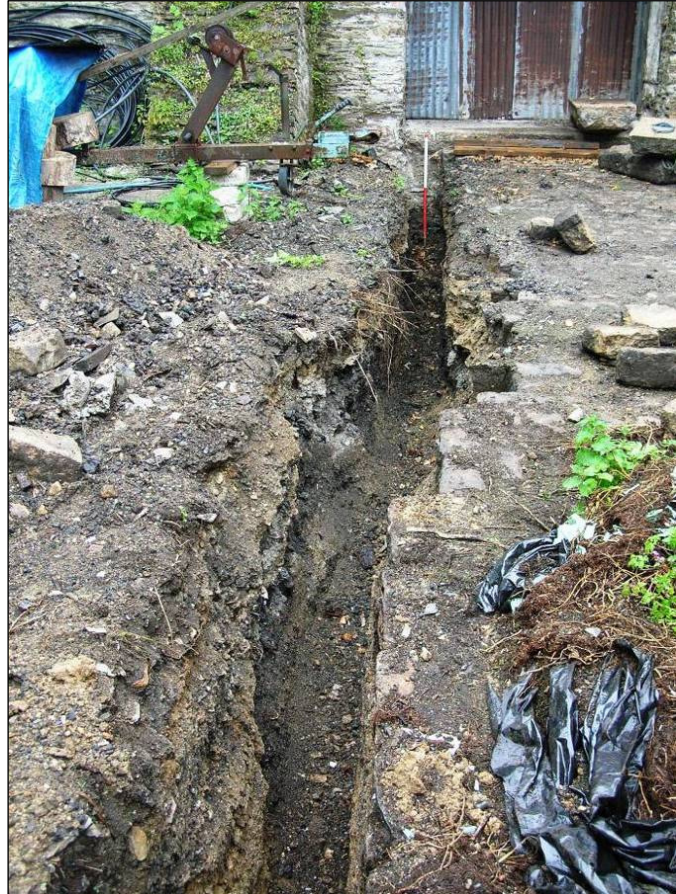
Figure 23 Photograph (looking east) of the excavated service trench across the former coal yard © CC HE Projects 19/5/2010
