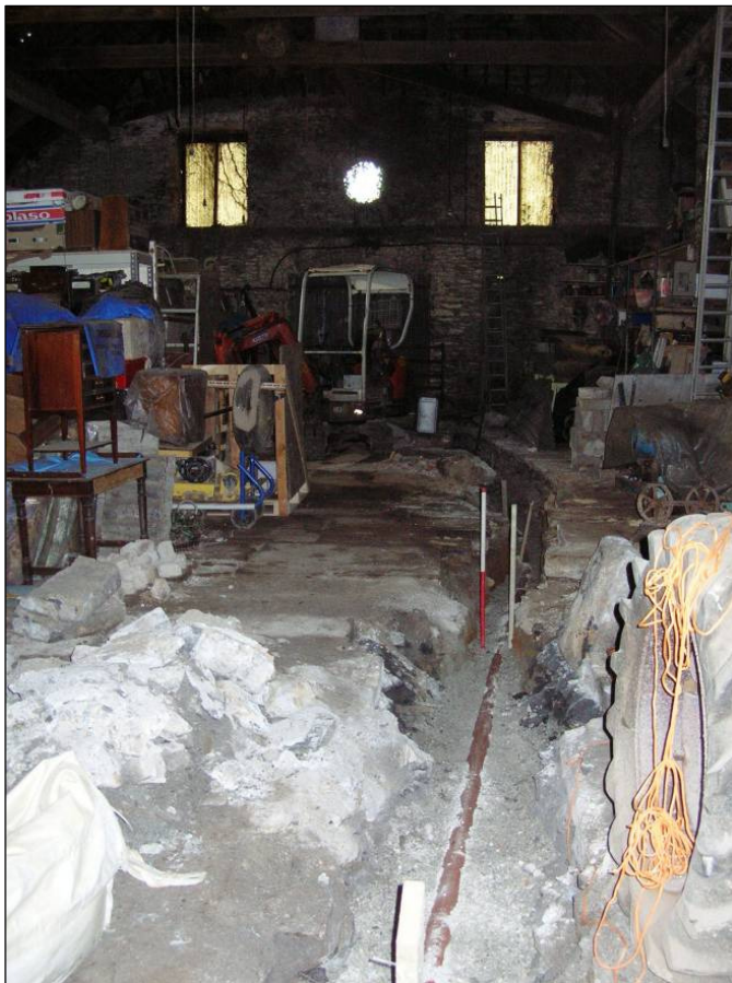
Figure 20 Photograph (looking west) of the excavated and partially infilled service trench across the former tin smelter floor © CC HE Projects 19/5/2010
