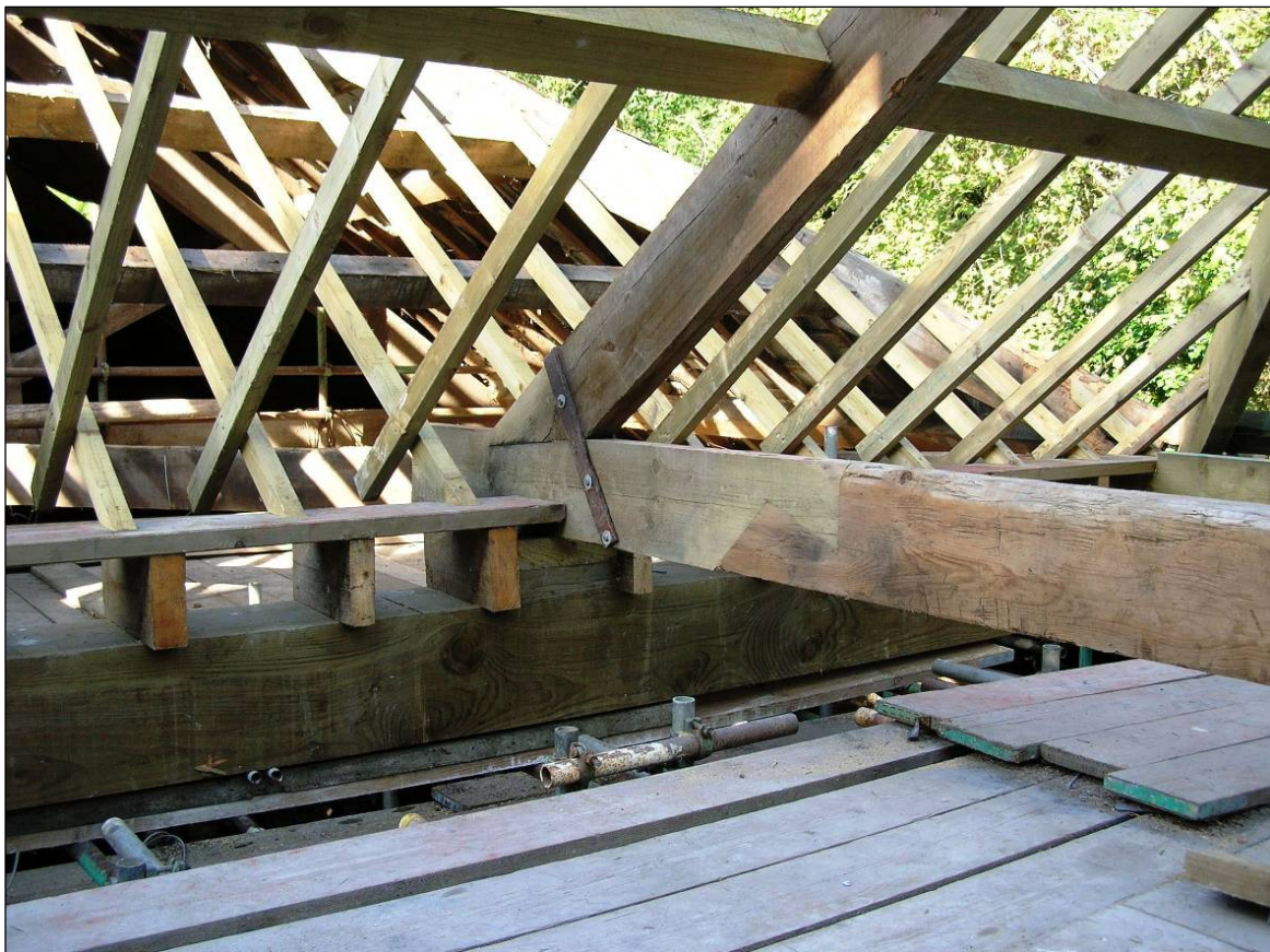
Figure 15 Photograph (looking west) of Site 41 (Smelter roof valley timber/re-scarfed 'A' frame truss) during roof rebuilding works © CC HE Projects 25/9/2009
