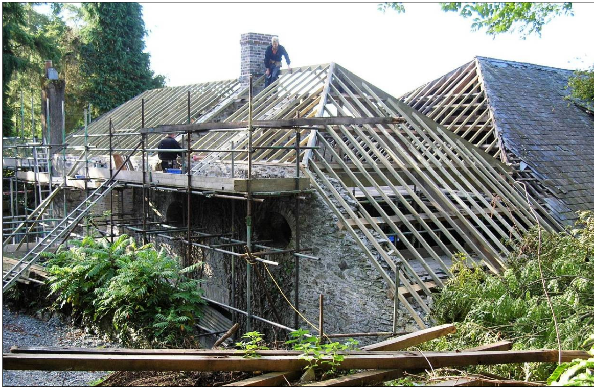
Figure 14 Photograph (looking south) of Site 41 (Smelter roof) during major roof rebuilding works © CC HE Projects 25/9/2009
