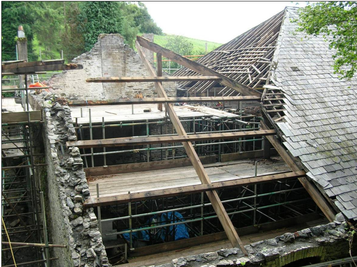
Figure 13 Photograph (looking south) of Site 41 (Smelter roof) during major roof rebuilding works © CC HE Projects 25/8/2009
