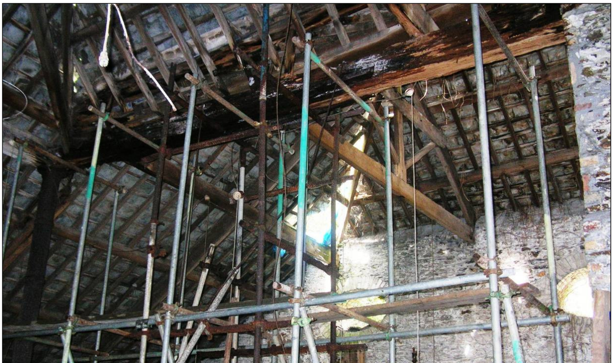
Figure 12 Photograph (looking north east upwards) of Site 16 (Smelter roof/wet main valley timber) before roof rebuilding works © CC HE Projects 14/7/2009
