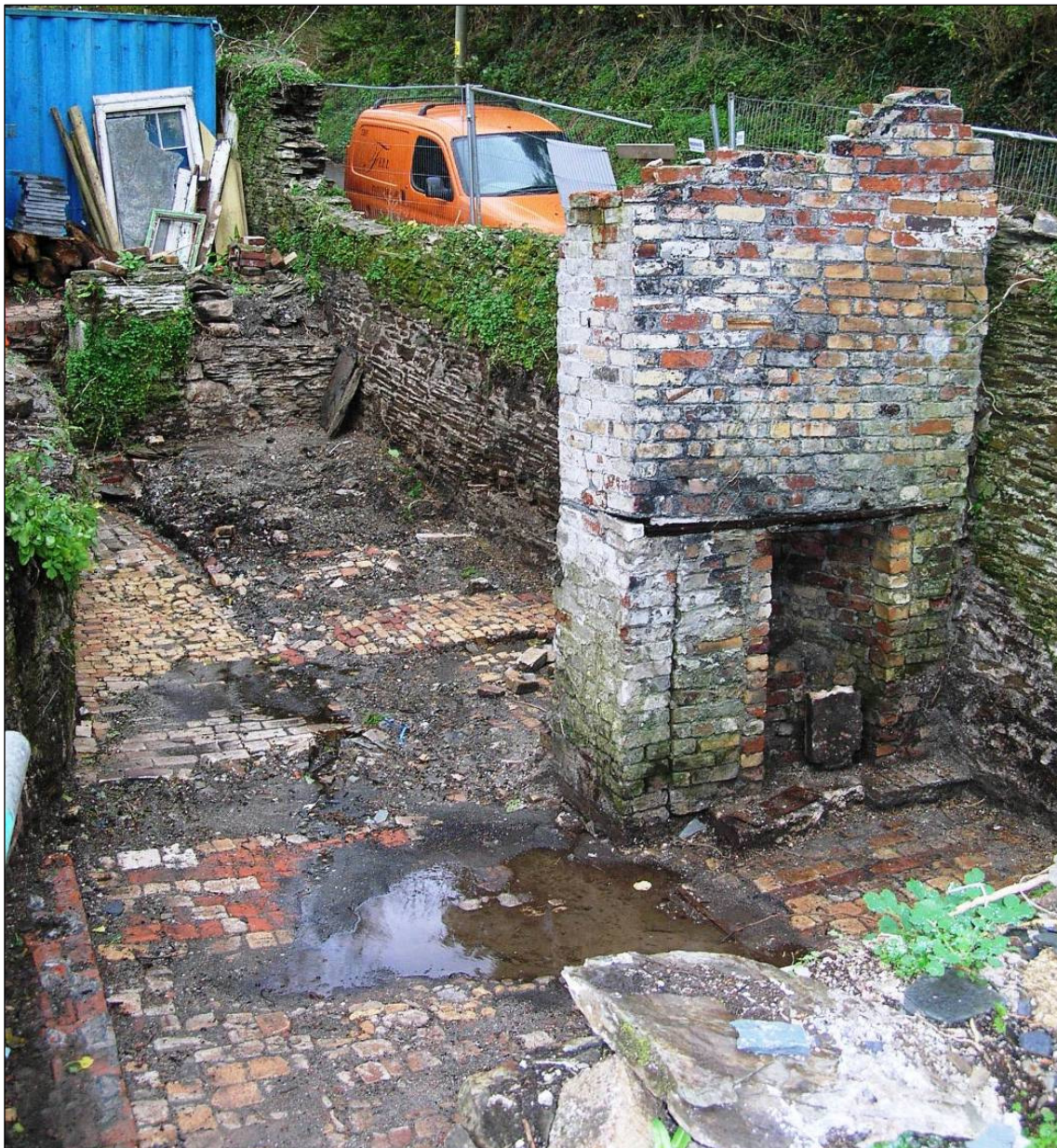
Figure 18 Photograph (looking east) of Sites 8 & 9 (Outhouses) after roof removal and prior to major rebuilding and groundworks © CC HE Projects 18/11/2009
