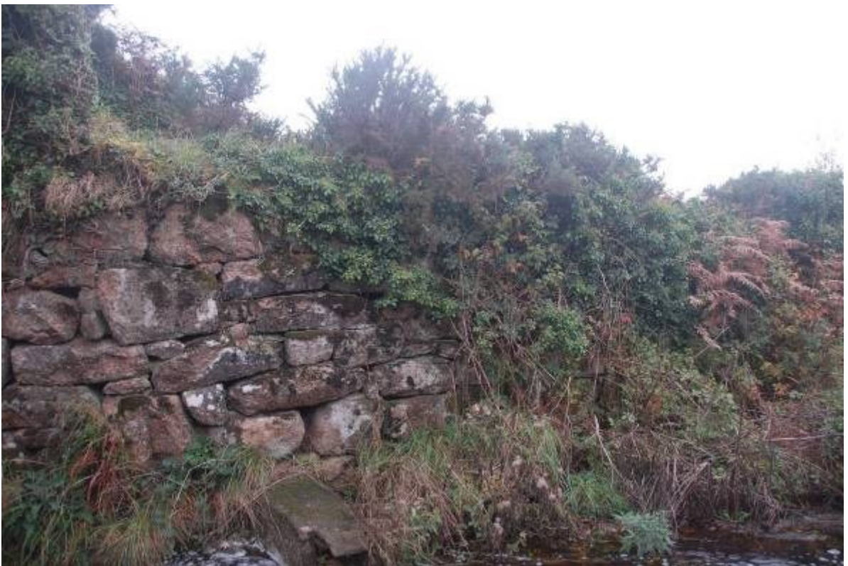
Fig 19. Looking across the stream to the wheelpit walling prior to the clearance of some of the obscuring vegetation. The concrete dam is just left of centre at the base of the wall.
