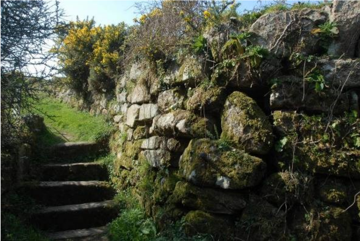
Fig 16. Looking west along the Church Path, showing the West Penwith stile and the poor condition of the corner of the spalling floor walling at this point.
