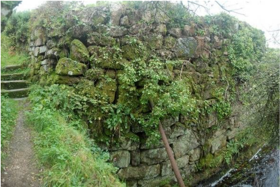
Fig 14. A composite image of the revetment walling to the spalling floor from the north-east showing the Penwith type stile on the Church Path (left) and the steel prop installed in 1987.
