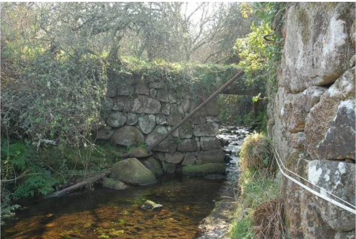
Fig 17. Looking south along the course of the stream showing the masonry buttress for the Church Path bridge and the tubular steel struts installed in the 1980s (one has now fallen into the stream).
