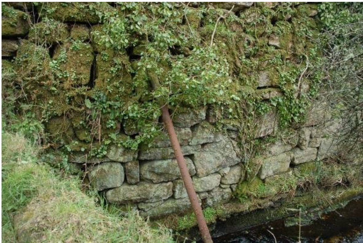
Fig 23. The lower section of the spalling floor wall adjacent to the bridge, showing the more open jointed and partly dislodged masonry in the upper part of the wall, the surviving steel strut, and the band of mass concrete along the foot of the wall.
