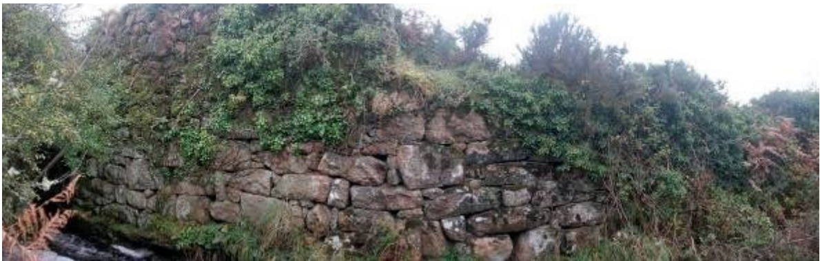
Fig 15. A composite image of the walling of the spalling floor (left) and wheelpit (right) from the east prior to vegetation removal in the winter of 2011/12.
