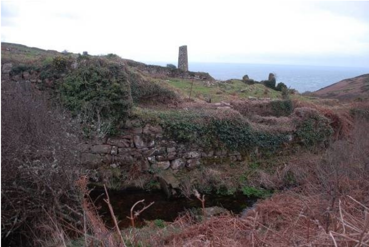
Fig 20. The spalling floor and wheelpit walling from the east following the removal of some of the obscuring vegetation by NT volunteer Rangers.
