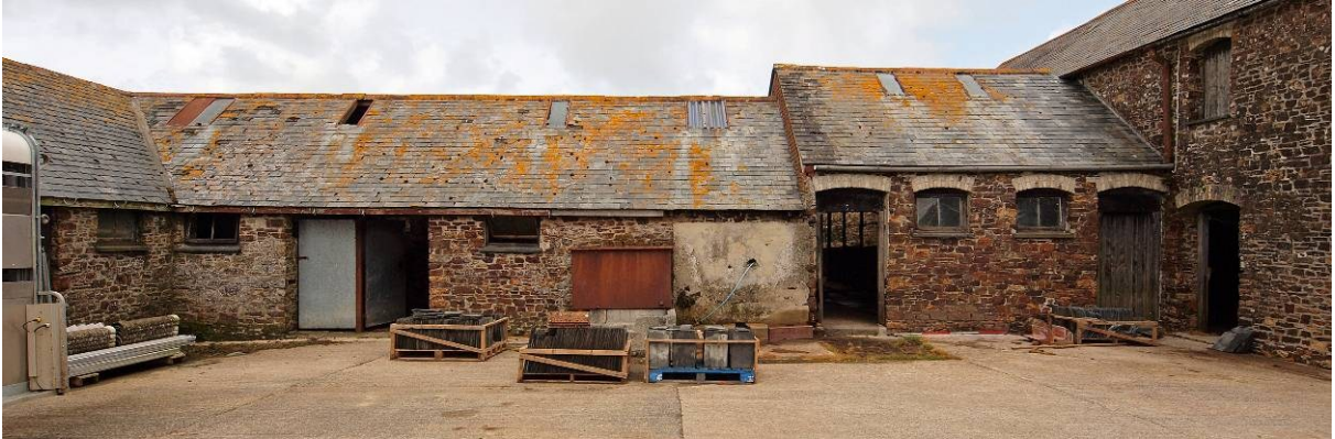
Fig 9 Building 3 (shippon- left) and the yard front of Building 5 (probably originally stables but later enlarged as a shippon- right)
