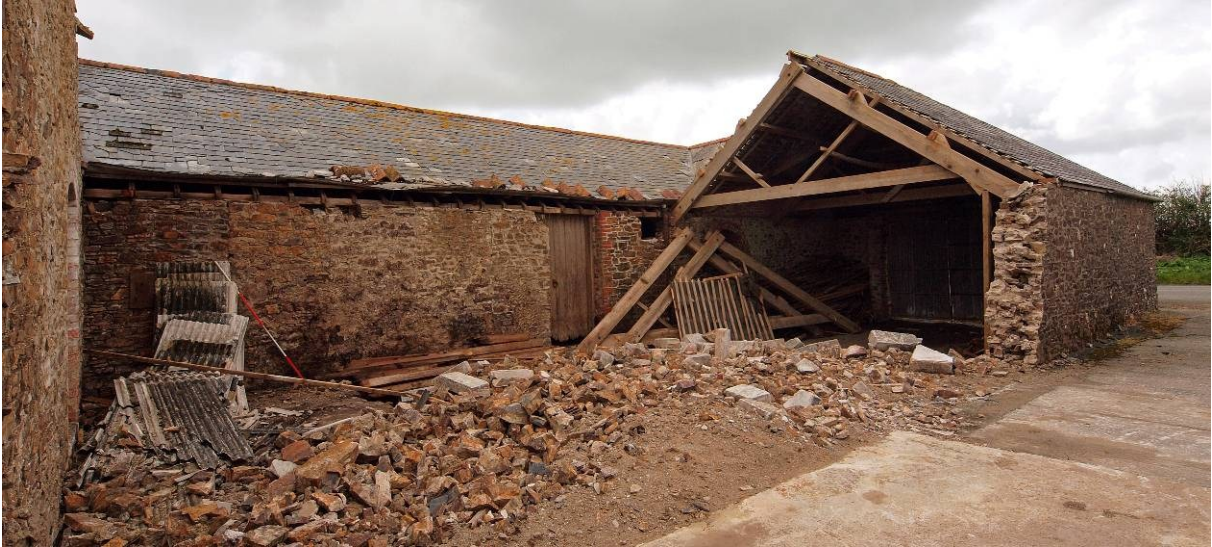
Fig 10 Building 3 (shippon) and partly demolished Building 4 (cartshed and probable dung store) from north
