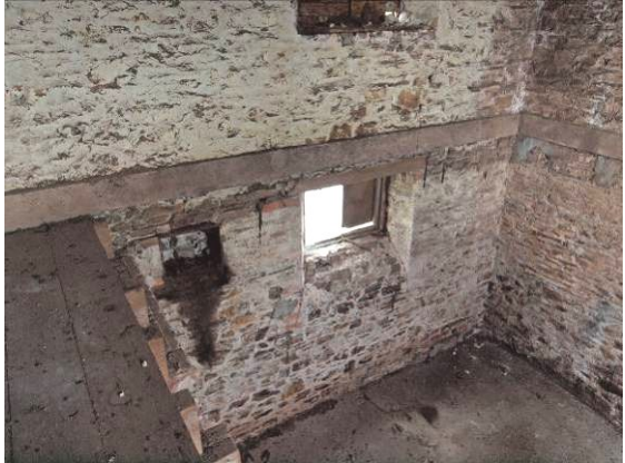
Fig 26 Building 1 E corner (remains of machinery)
