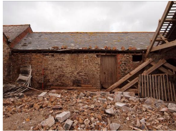
Fig 63 Building 3 (shippon) with evidence for former adjoining Building 4
