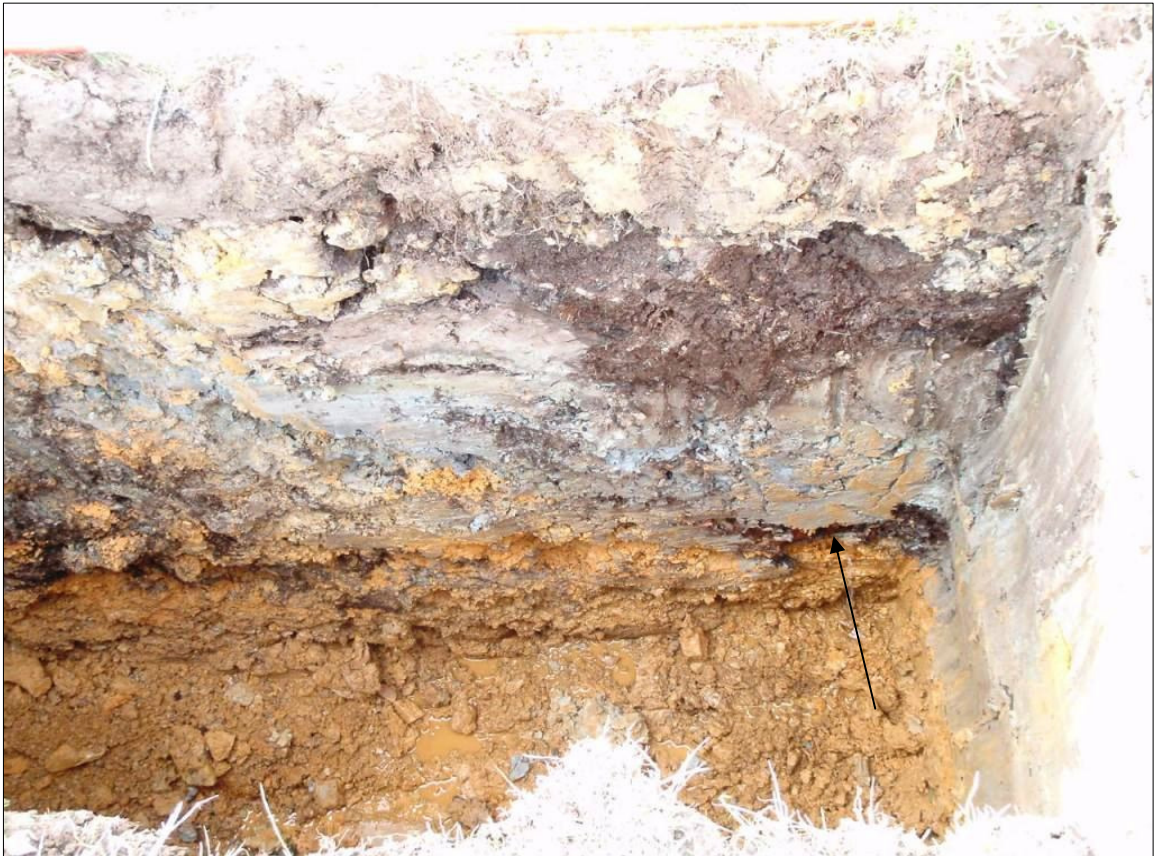
Fig 2 Trench 8 post-excavation: South facing section looking north into trench (approx 2.2m deep). Note, the very mixed nature of soil infilling the large cut for the land drain. An arrow marks the location of land drain. (Ranging rod lying at top of trench bleached out in image by strong sunshine).
