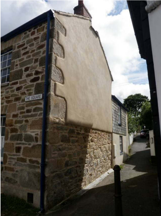
Fig 9 North-west external elevation showing stone masonry at ground floor level and cob at first floor level, also service wing extension to the rear
