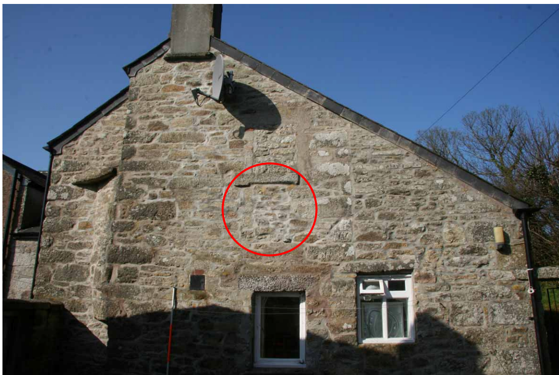
Fig 10 Gable of farmhouse rear wing, with 19 th century dairy lean-to towards the right A blocked earlier window is shown circled (and is also marked in green on Fig 39)
