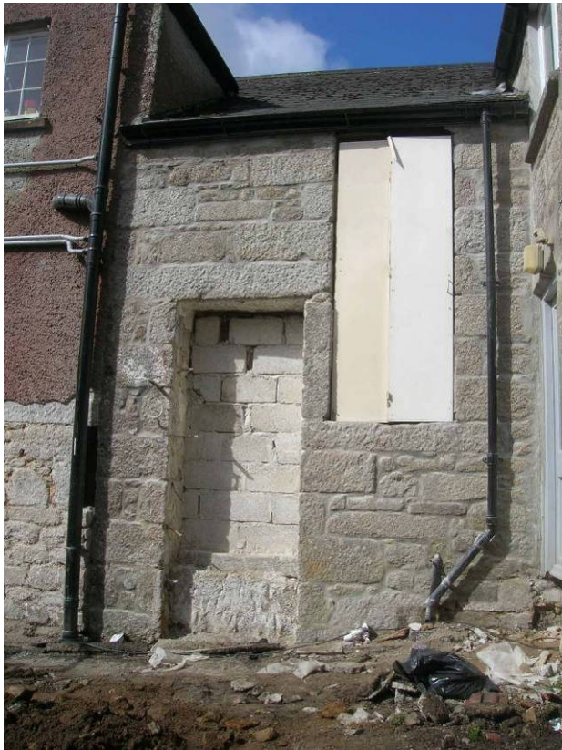
Fig 11 Rear stair hall of farmhouse, masonry exposed after removal of modern roughcast render
