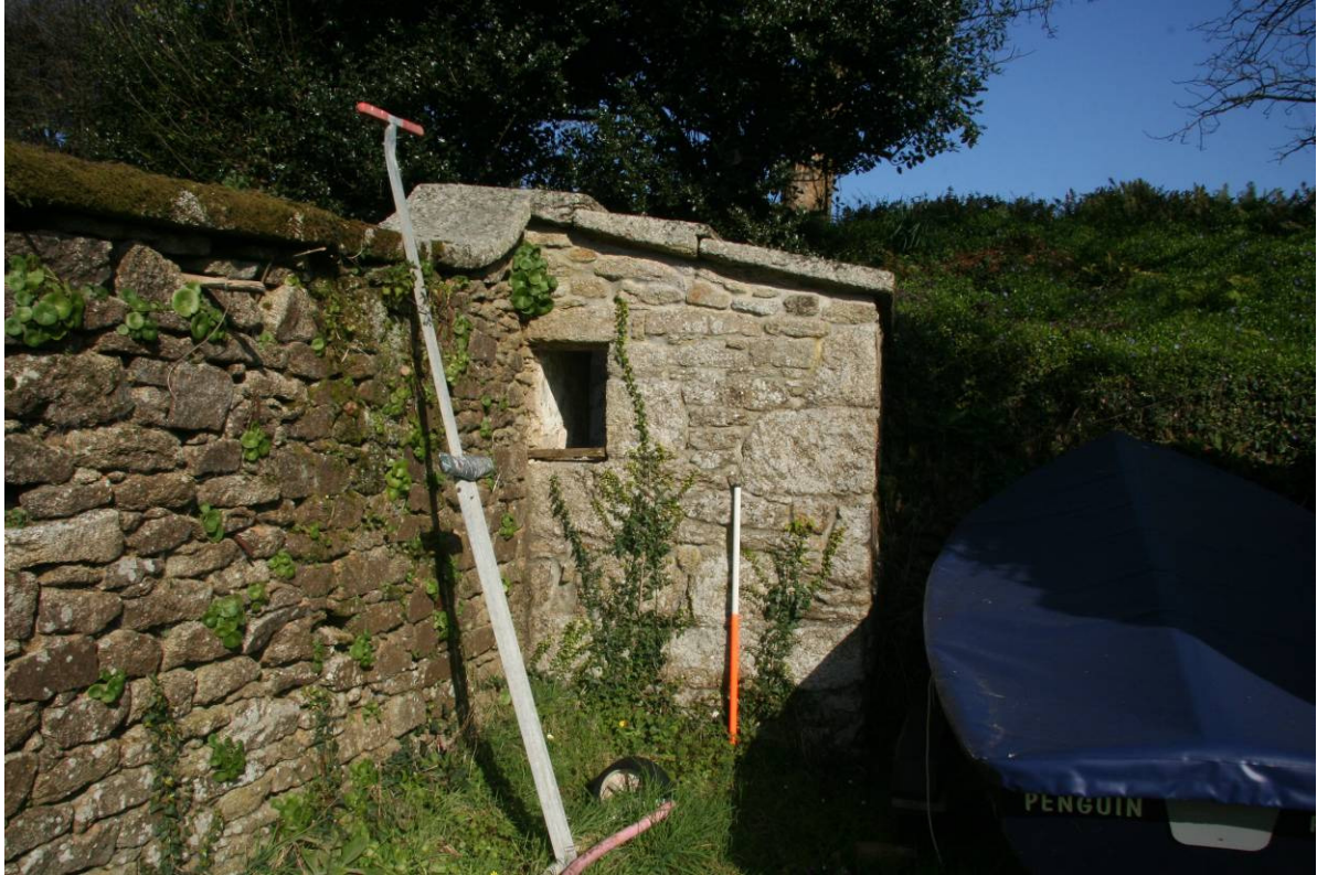
Fig 15 The earth closet, viewed from the farmyard, with kitchen garden wall to left Note the very unusual, if not unique, overlapping granite slab roofing
