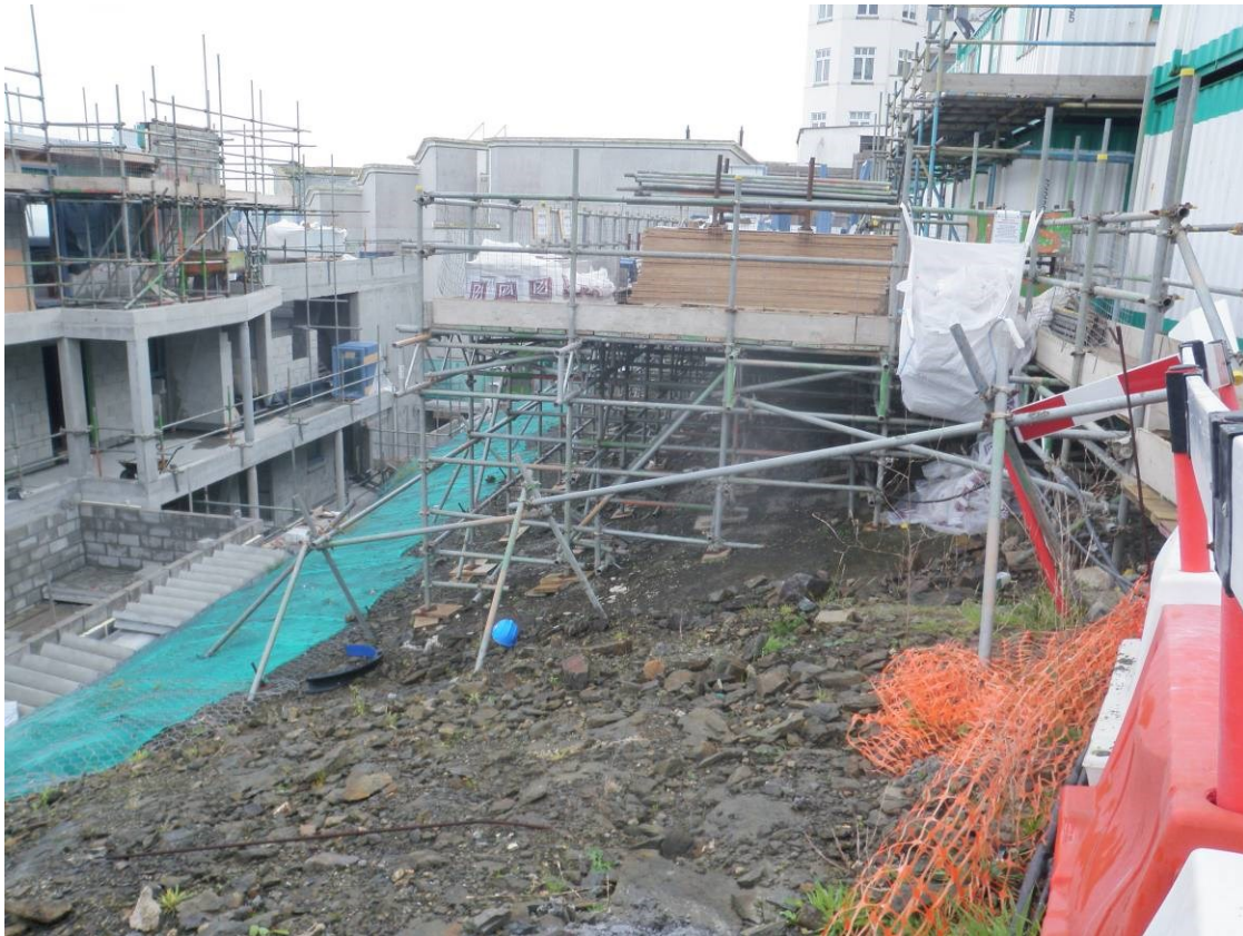
Fig 11 View of the northern half of the development area (excavated down to bedrock) looking east
