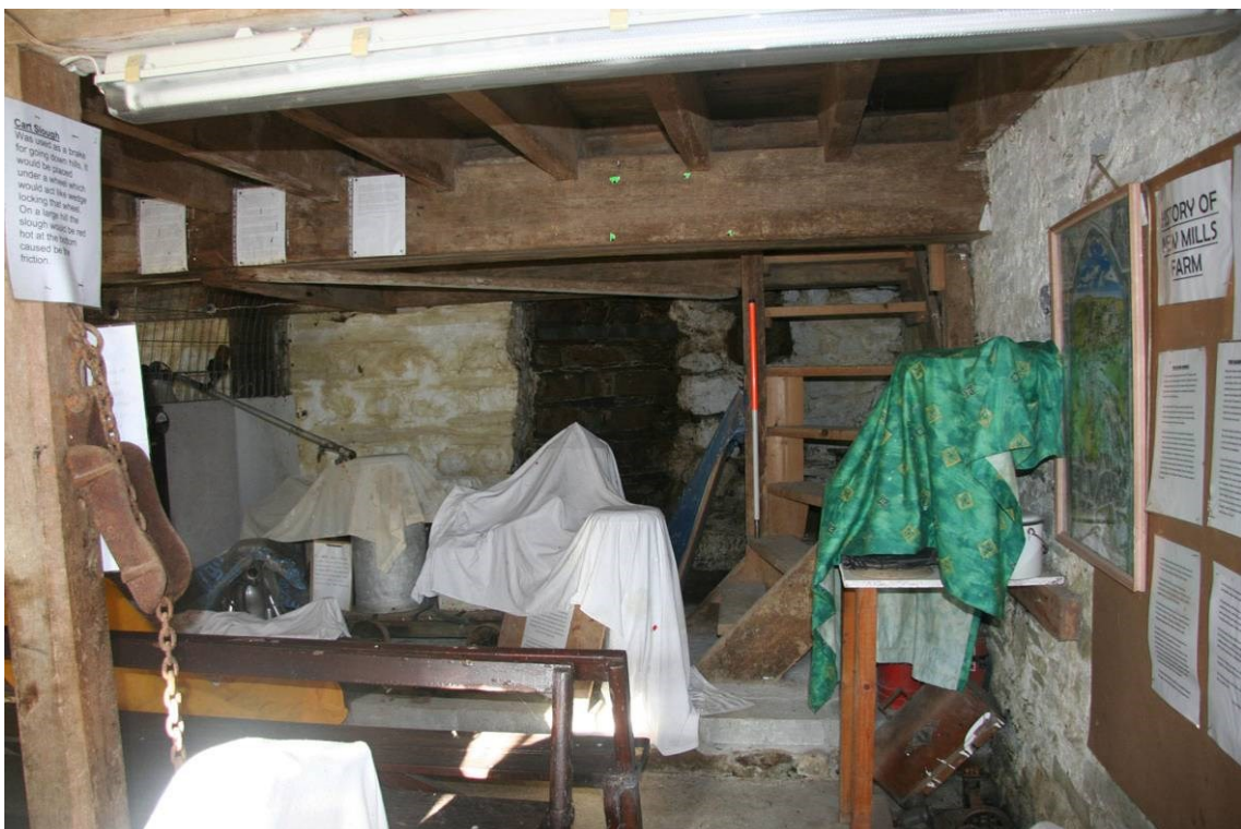
Fig 24 Ground floor of the mill, showing winder stairs to the stones floor (on the right)
