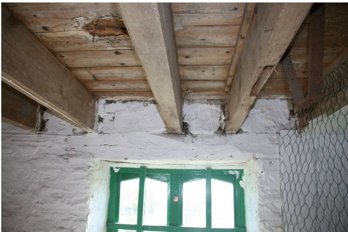
Fig 36 Another axle support bracket on the south side of the first floor This part of the mill probably once contained cleaning/grading machines
