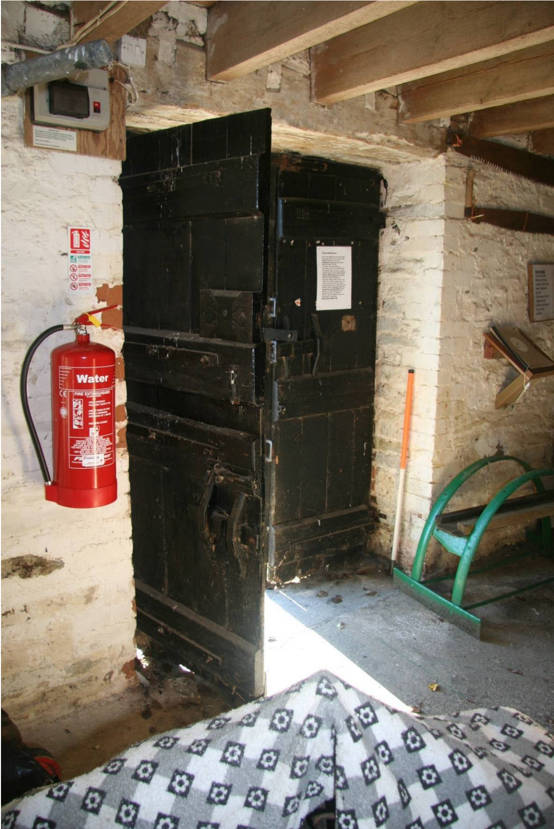
Fig 22 The main entrance of the mill, with a split door in the foreground showing latch and lock detail
