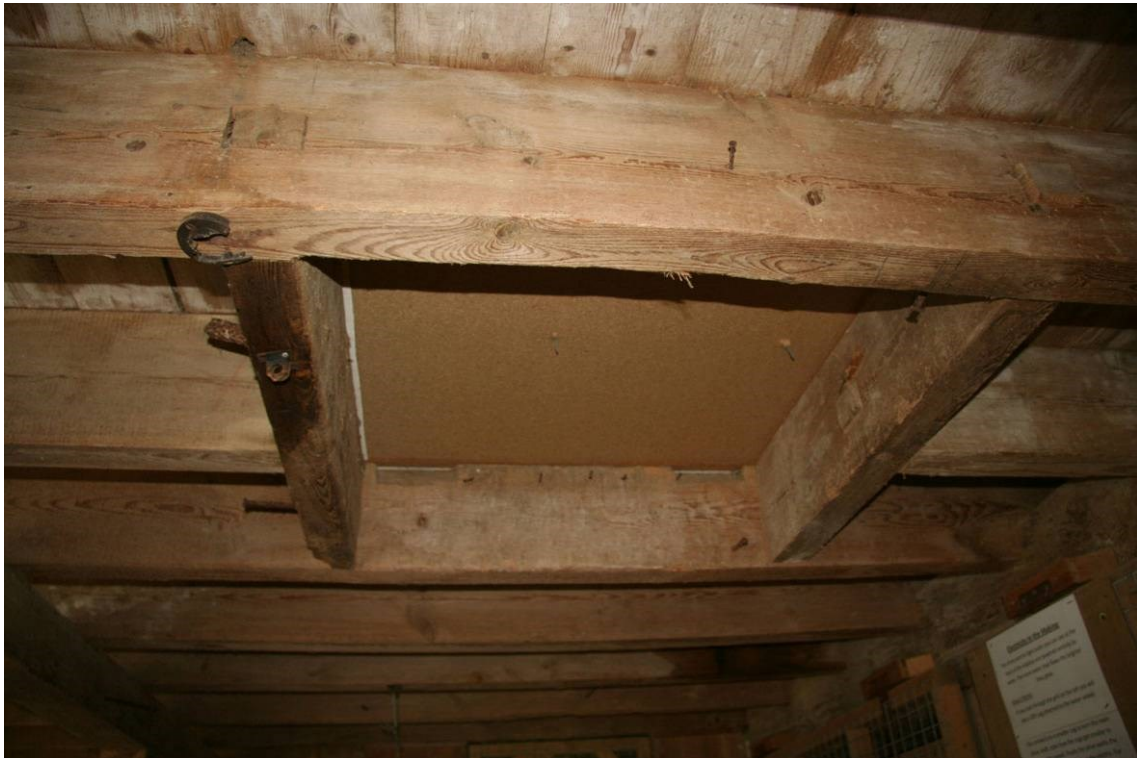
Fig 27 Sack hoist hatch between the ground and first floors Note the shallow cut-outs for the hinges of the trapdoors
