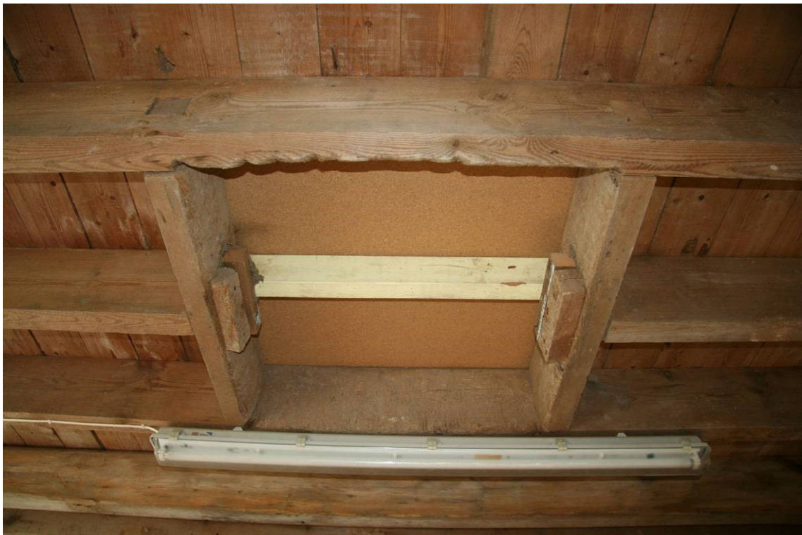
Fig 28 Sack hoist hatch between the first floor and loft level Note the wear on the floor joists caused by the ropes when the hoist was in use
