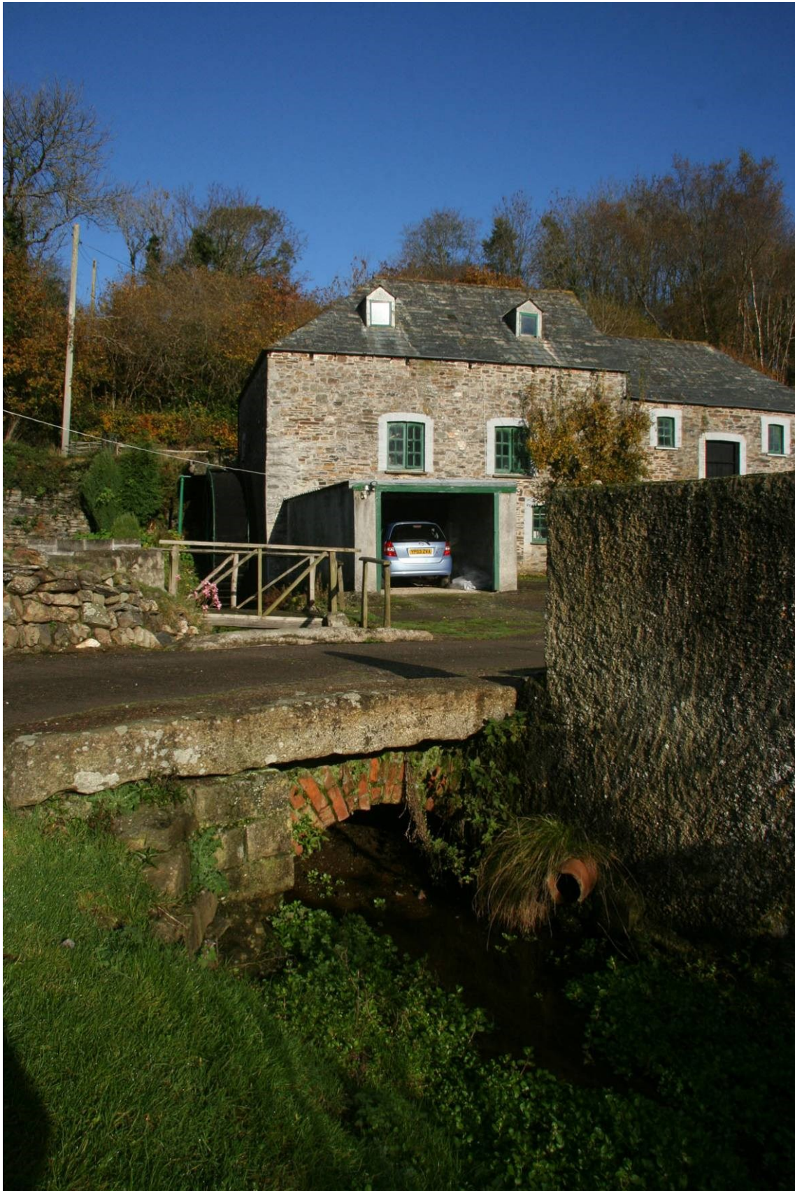
Fig 21 A brick arched bridge carries the mill access track over the tailrace channel
