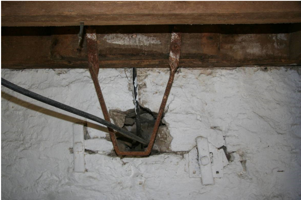
Fig 35 Axle support bracket (and hole through the wall) for line shafting to subsidiary machinery
