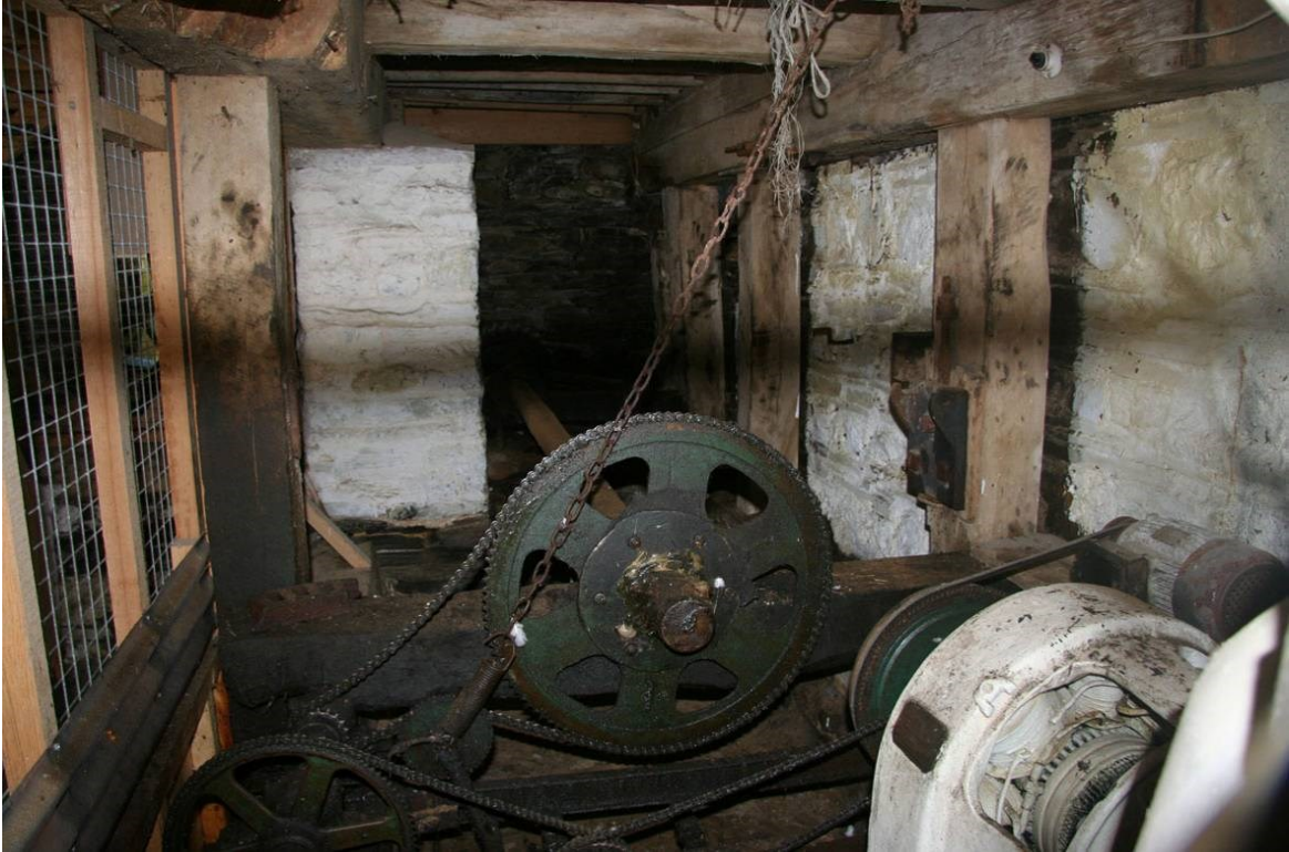
Fig 25 The end of the countershaft (centre), now driving a dynamo via chains and sprockets
