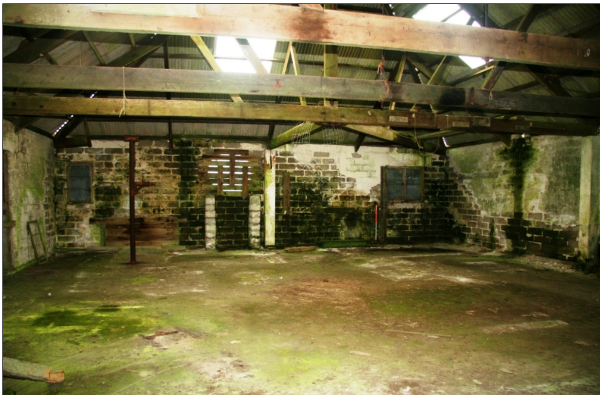
Figure 28 An internal view of the diesel engine house (Site 7) looking westwards towards the site of the two engines (© CC HE Projects)
