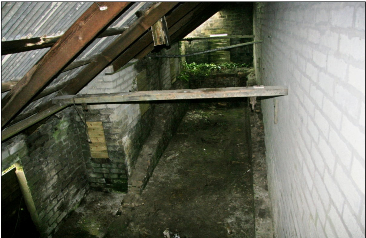
Figure 25 An internal view of the Boiler House (Site 3.2) from the north (© CC HE Projects)
