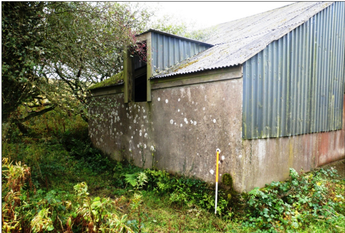
Figure 31 Winding engine house complex (Site 41) east side showing the opening for the winding wire (© CC HE Projects)
