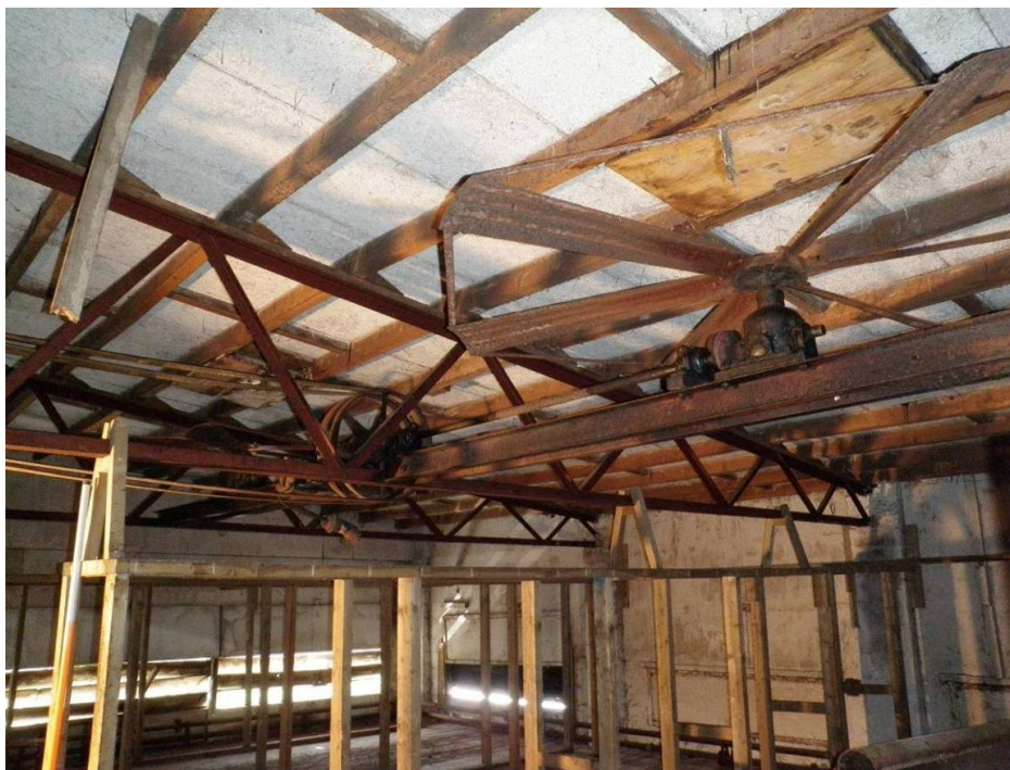
Fig 40 Building 5, first floor interior showing drying loft fan, drive wheels and belts looking north-west
