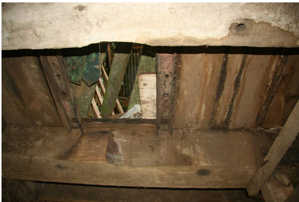
Fig 73 Building 11b, hatchway in first floor and worn beams associated with former Valonia mill above
