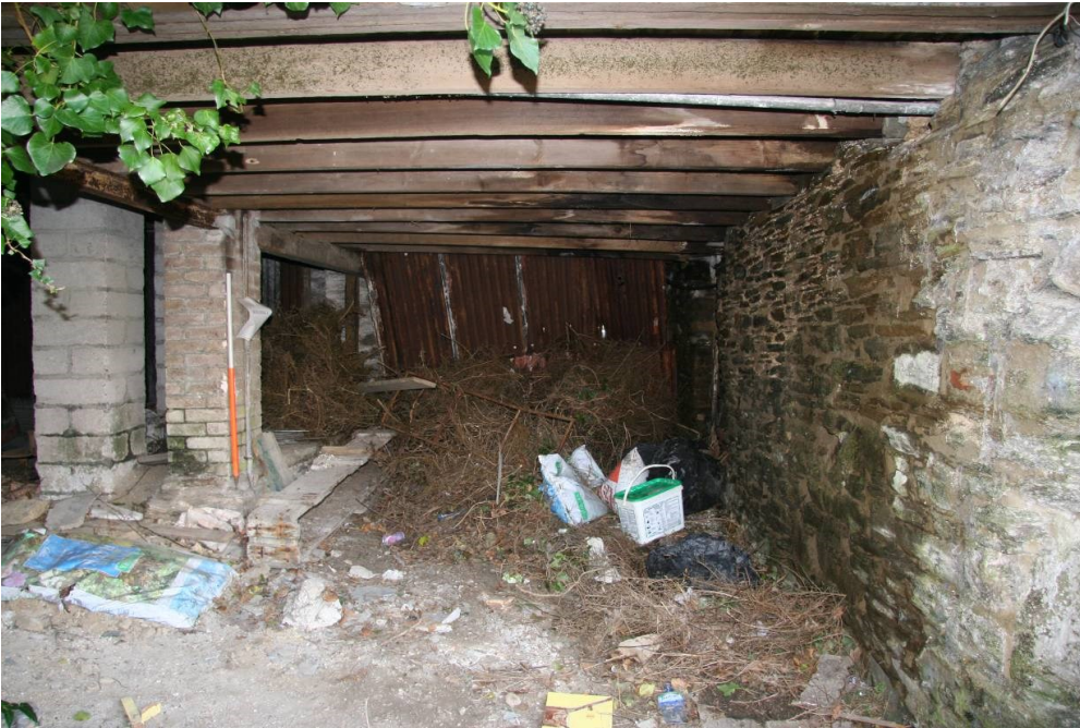
Fig 34 Buildings 3/4, ground floor interior looking south. Site of former lane between Buildings 3 and 4.
