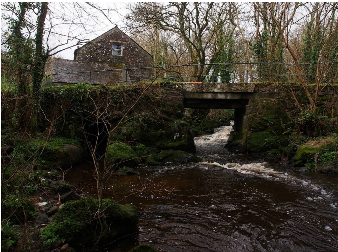
Plate 15 View from below the bridge. The left hand (mill tailrace) opening appears to be the earlier part of the structure
