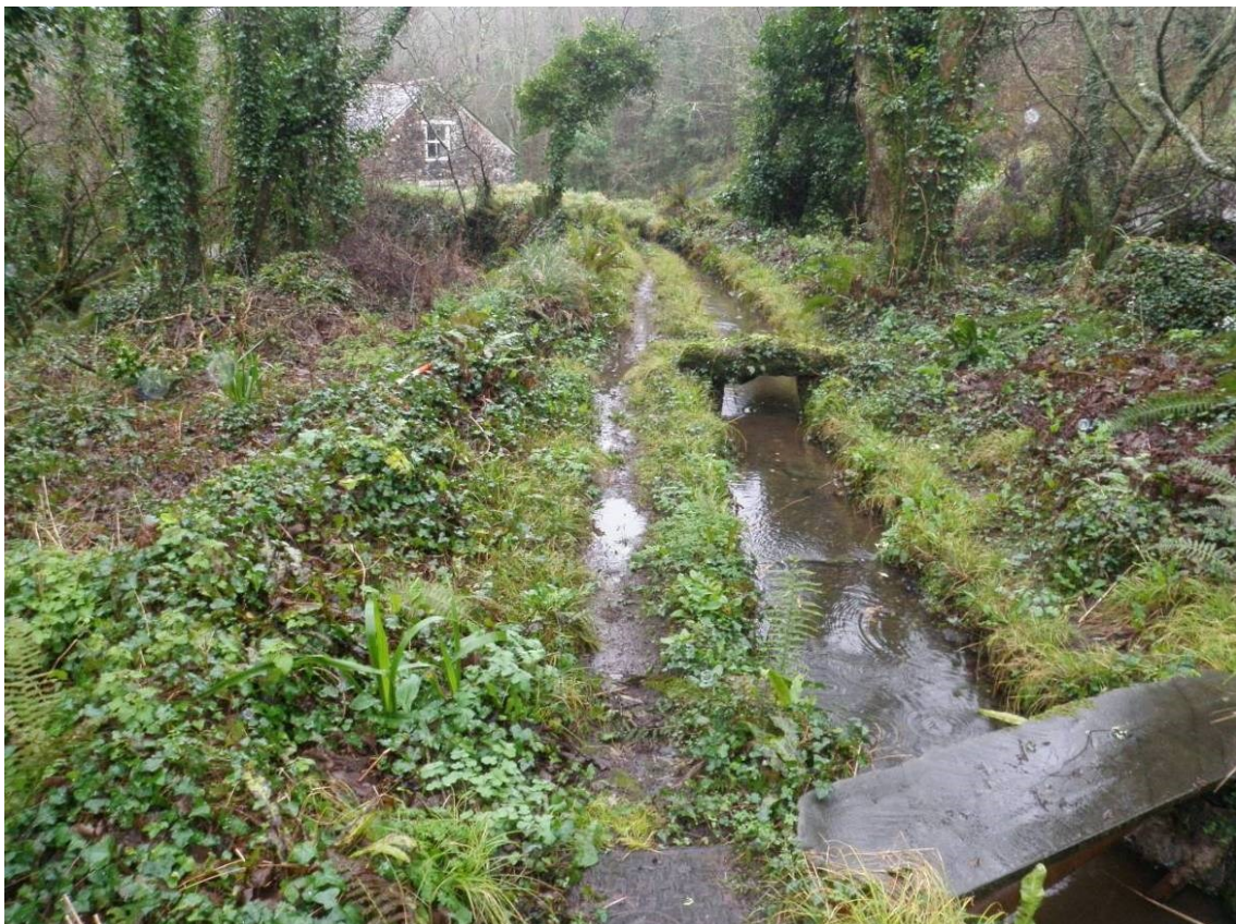
Fig 25: Poltesco Mill leat 92520 set on top of serpentine rubble-retained bank looking east
