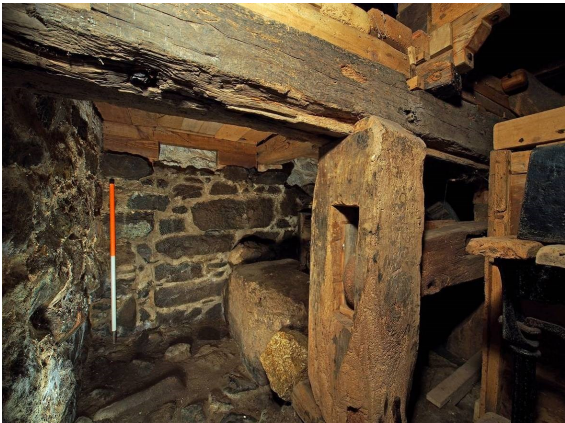
Plate 28 Blocked vertical slot in NW corner hints at earlier arrangement of bridgework
