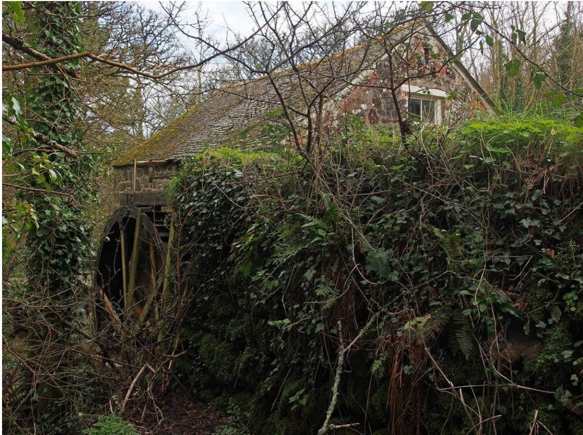
Plate 7 Rear view of the mill, showing (to the right) the wall supporting the leat
