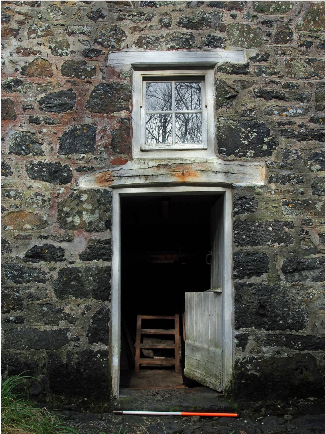
Plate 16 View of the main doorway into the mill, with ladder stair to upper floor visible inside. Note the OS Bench Mark cut into the wall at lower right of the doorway, and the iron tethering ring
