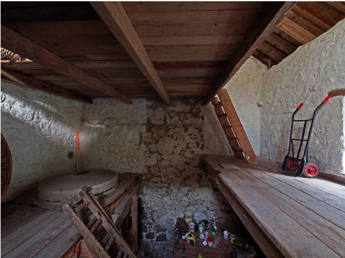
Plate 32 View towards the NE wall at first floor level. Note the change in build and narrowed wall thickness (above the scale bar)
