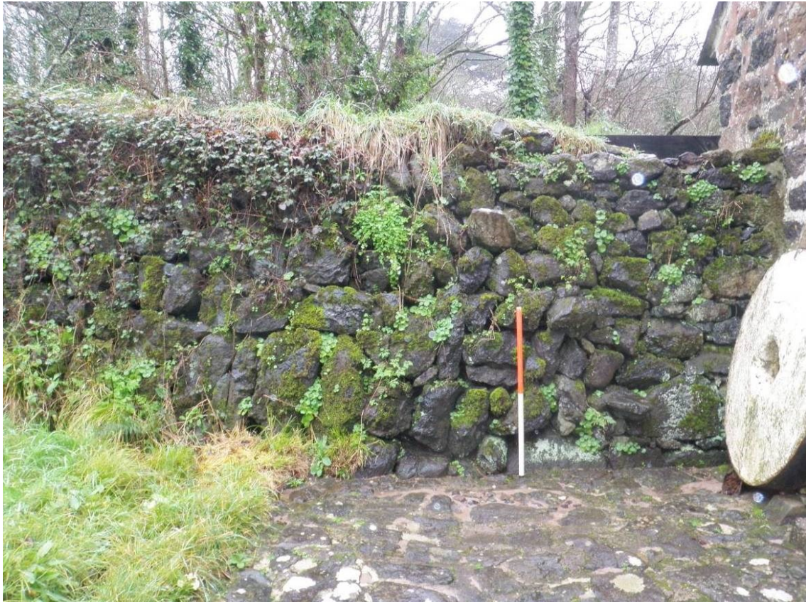
Fig 24: Poltesco Mill leat 92520 set on top of serpentine rubble-retained bank looking north-west
