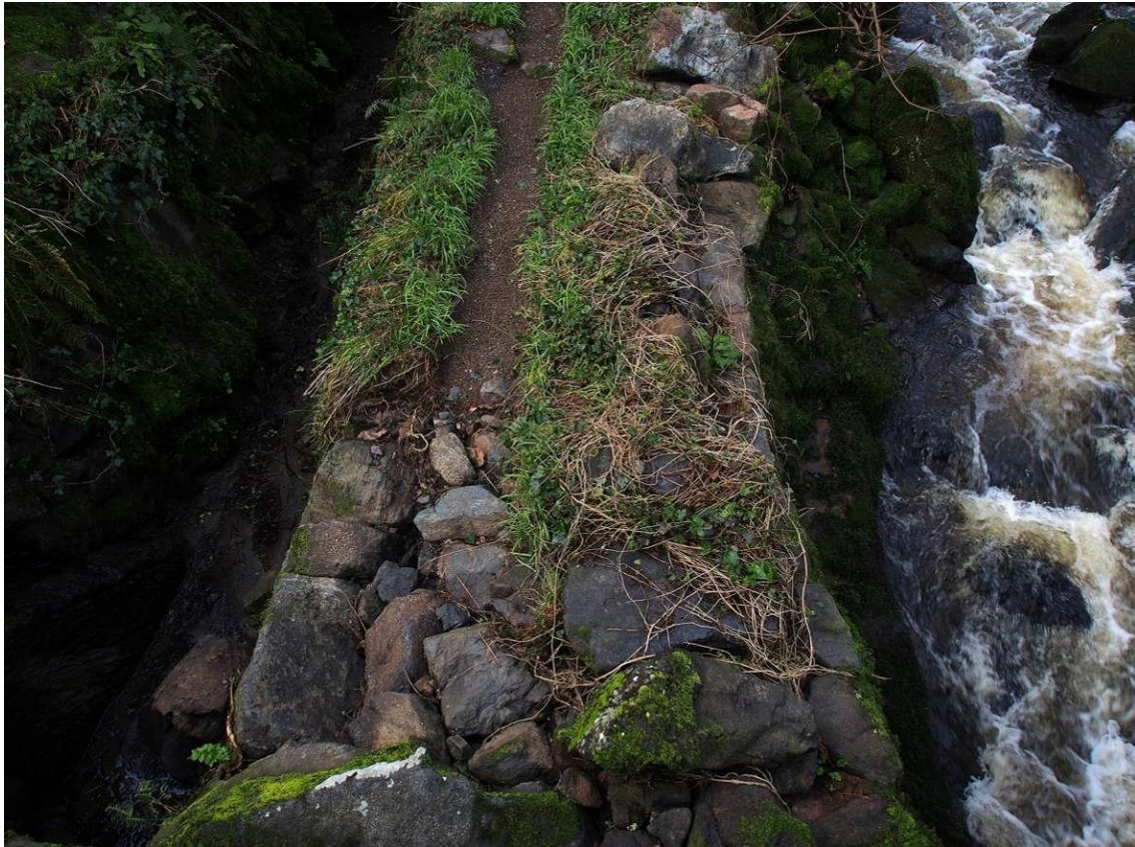
Plate 14 The wall separating the tailrace from the adjacent stream. Flood damage in November 2012 has displaced the upper course of stones (left)
