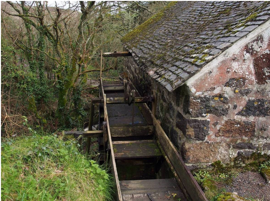
Plate 10 View of the launder feeding the wheel (note missing boarding caused by flood damage in 2012)
