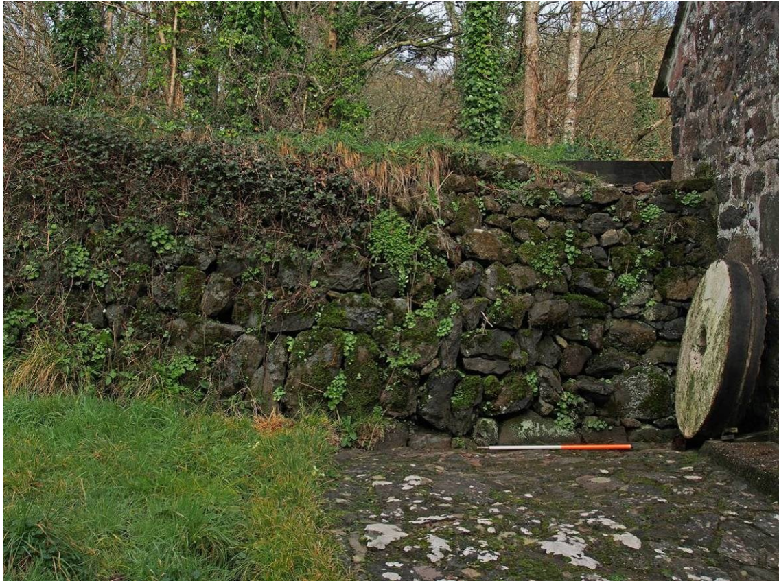
Plate 11 The wall supporting the leat adjoining the mill building. A step-stile has been incorporated into a rebuilt section of the wall towards the right. This rebuild would appear to date from the time the mill was extended towards the SW
