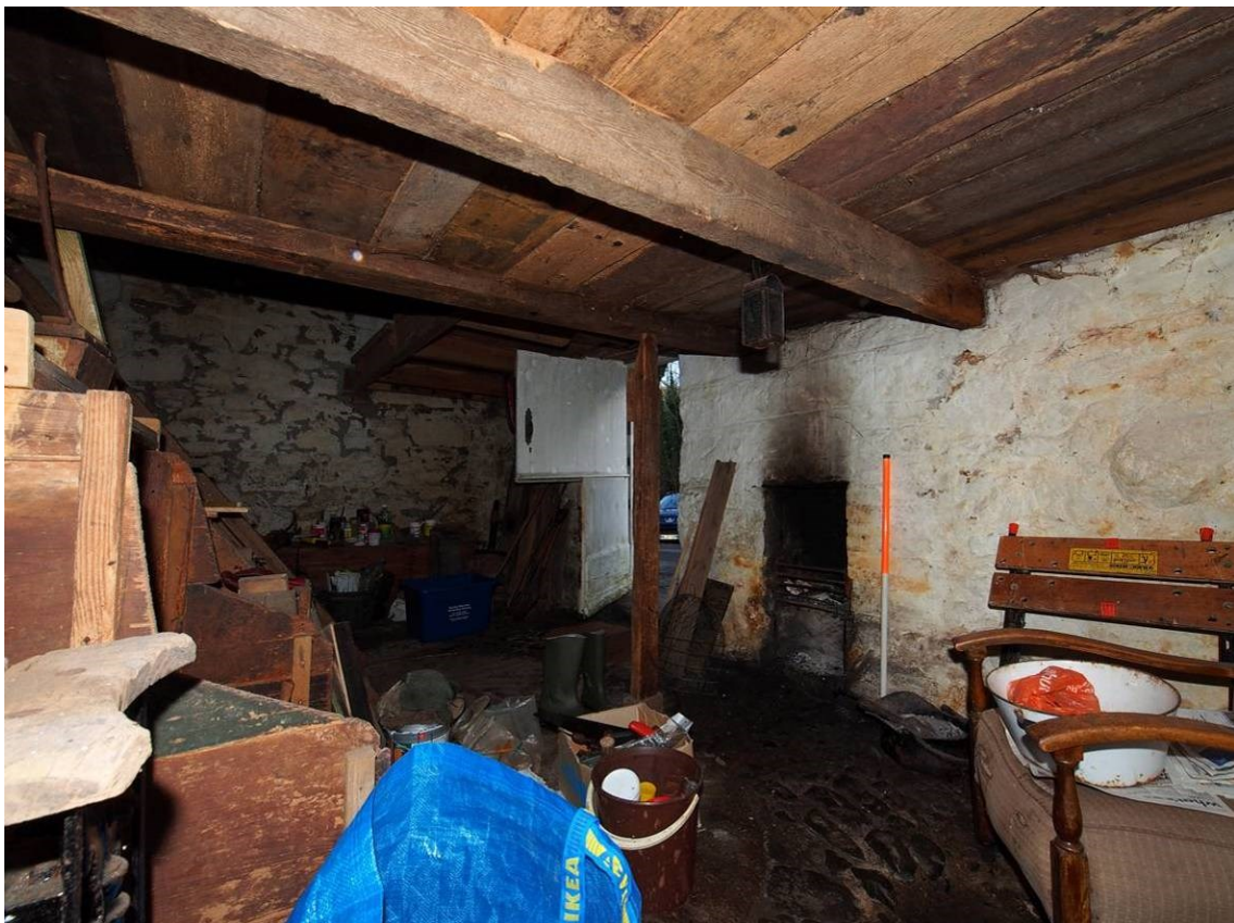
Plate 22 The ground floor of the mill, with the fireplace towards the right
