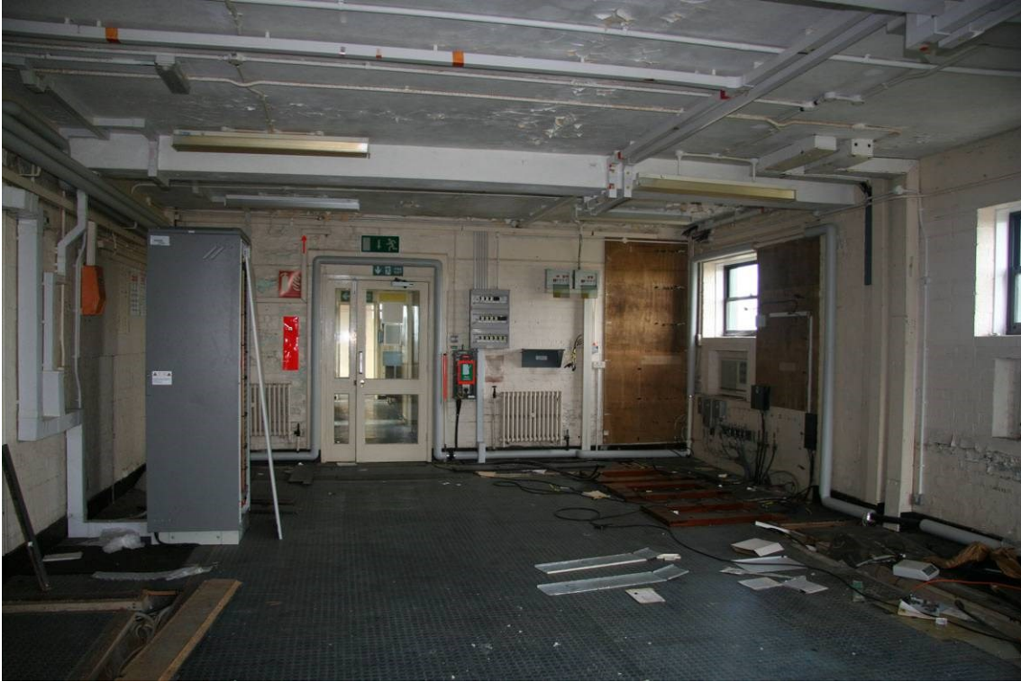
Fig 26 Radio Equipment Room, looking northwest
