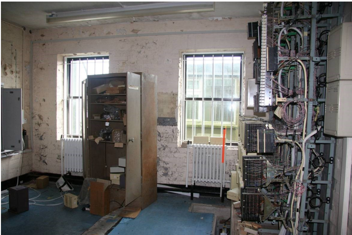
Fig 24 Frame Room on ground floor, with remains of telecom panel to right
