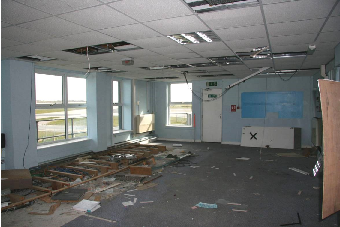
Fig 54 Radar Control Room, looking east
