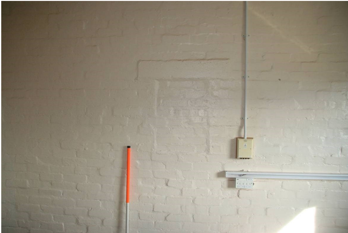
Fig 41 Blocked serving hatch within Senior Met Forecaster's Office (from mess room behind)
