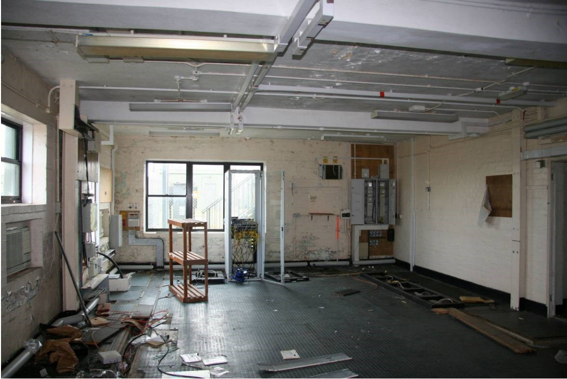
Fig 25 Radio Equipment Room, looking southeast
