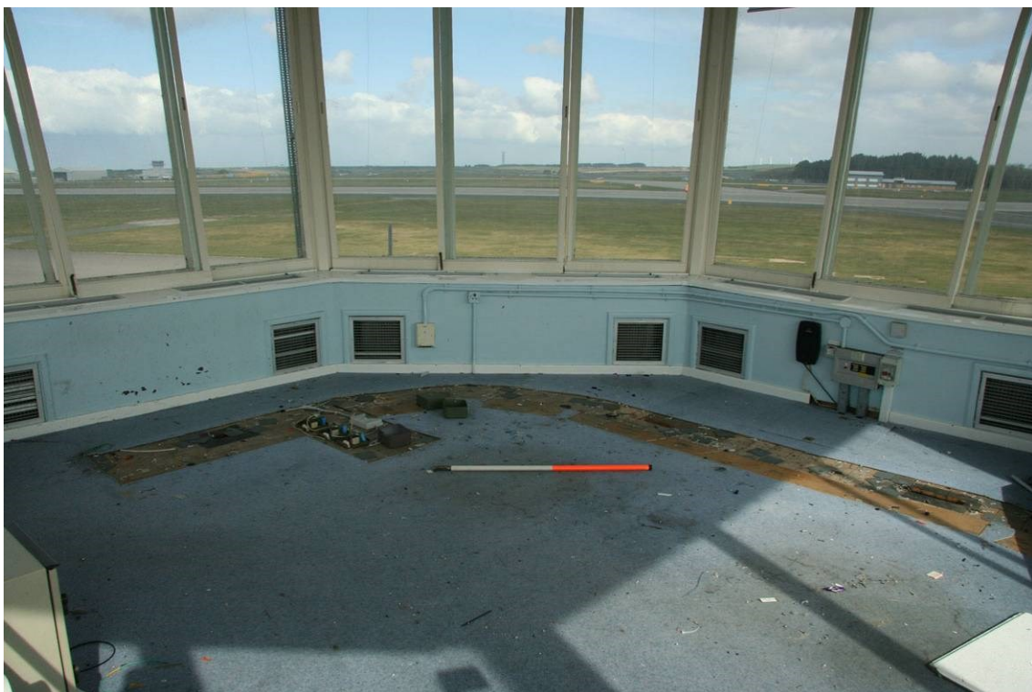
Fig 57 Interior of the Visual Control Room; the ghosting on the floor indicates the position of the desk
