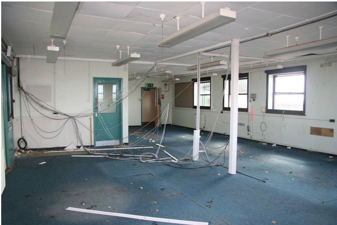
Fig 48 Met Office Forecasters' Room, looking southeast
