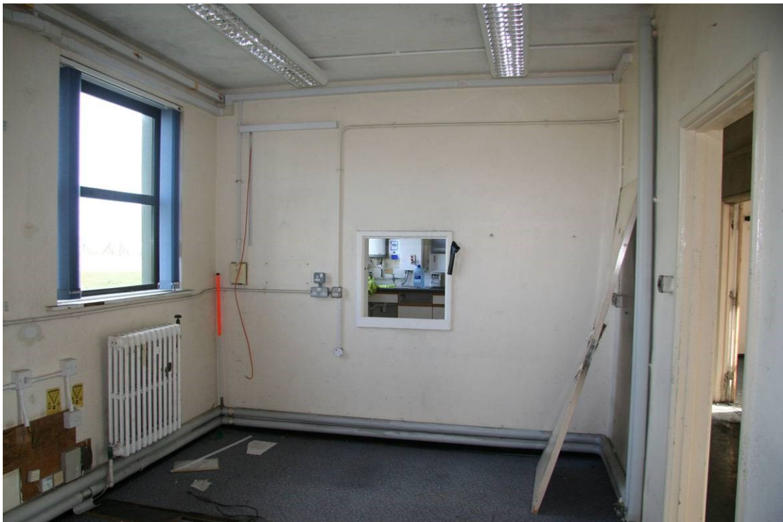
Fig 28 Eng Control room, probably a former mess room connected by a hatch, within the NW Wing
