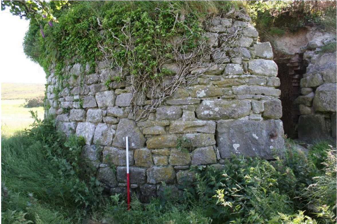
Fig 23 South-east elevation of kiln. The ranging rod is resting on top of the possible below- ground flue which may connect to the former chimney
