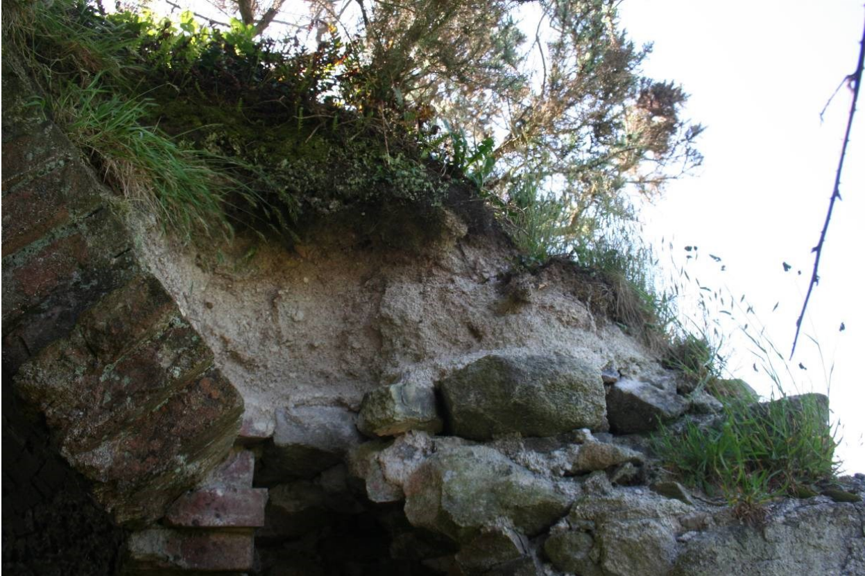
Fig 25 Detail of render roof covering bridge the angle between the top of the stone wall and the brick roof structure
