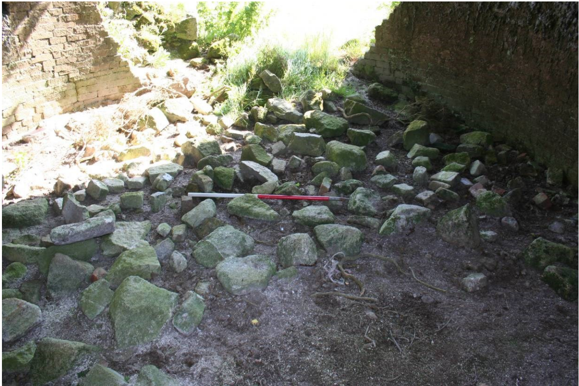
Fig 31 Collapsed rubble and earth covering the interior floor surface
