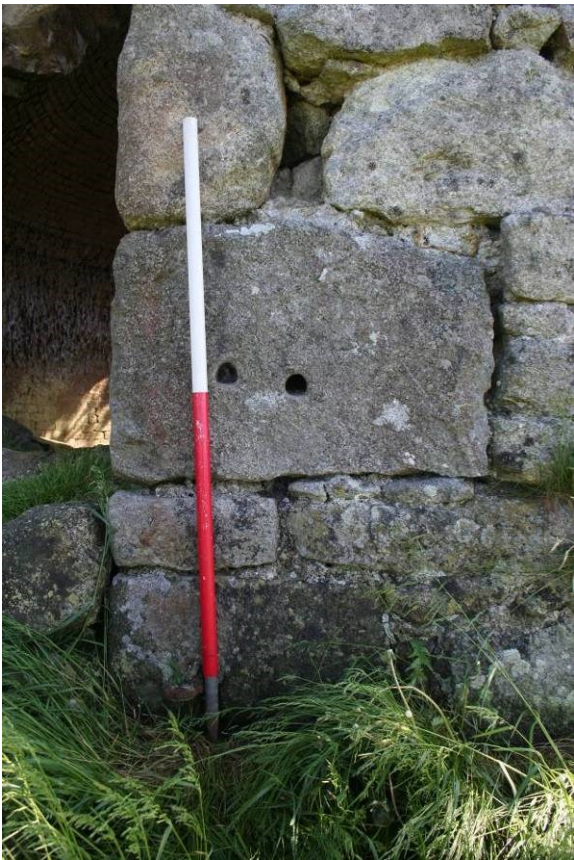
Fig 14 North jamb of north-east loading door with drill holes and iron pin below for fittings
