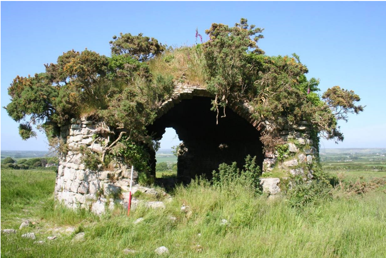
Fig 18 South-west elevation of kiln showing collapse around former loading door
