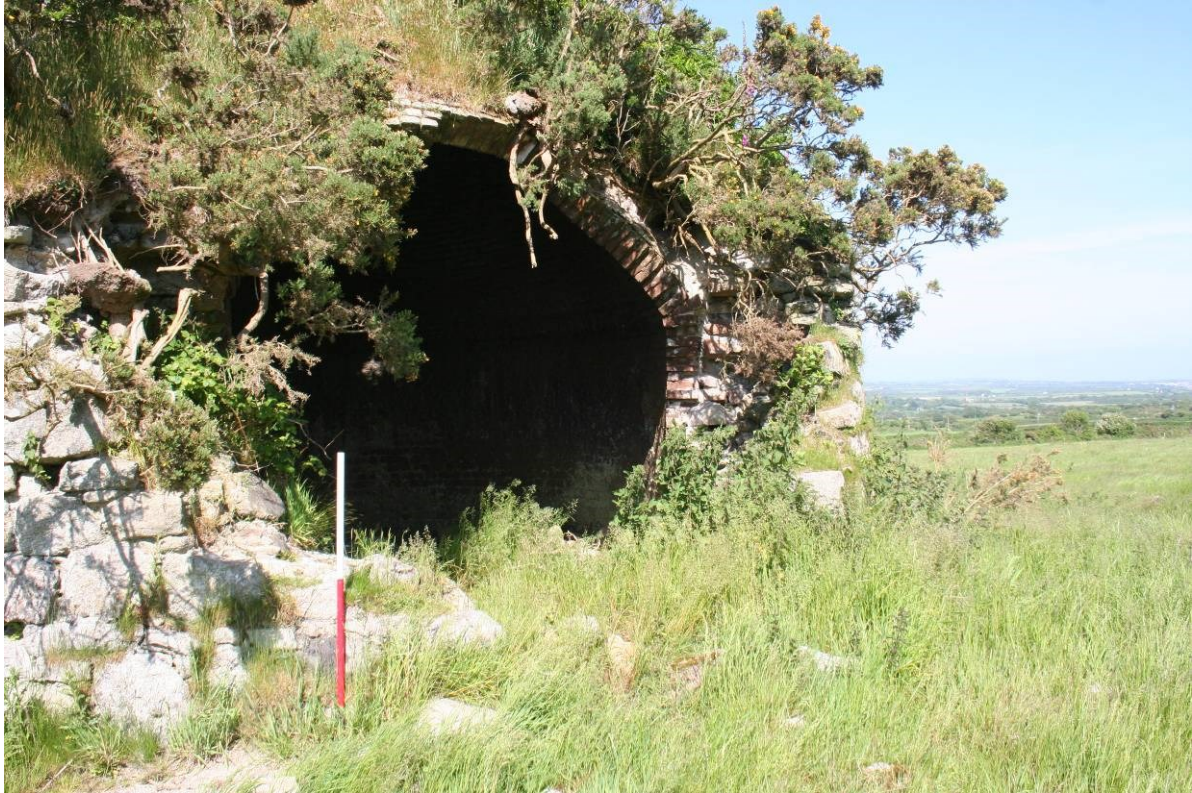
Fig 19 Collapse around former south-west loading door showing section through stone wall with brick lining
