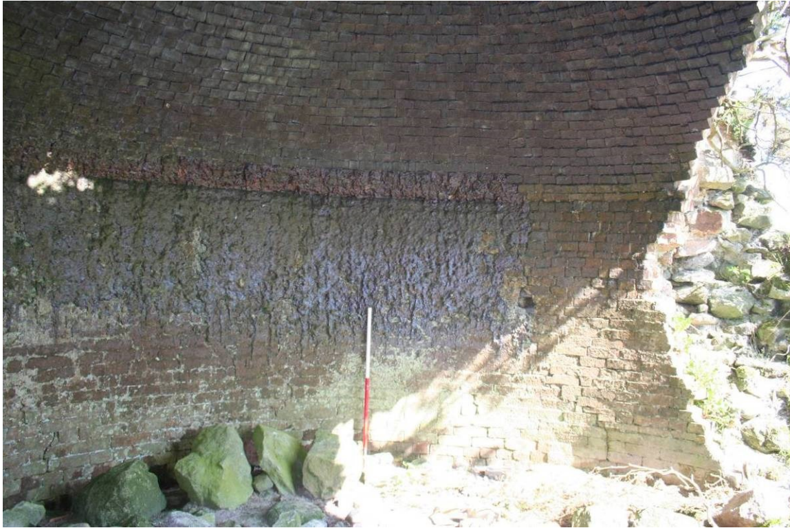
Fig 27 Interior of south wall of kiln showing vitrified brickwork in the upper half of the wall and a replaced section of brickwork to the right
