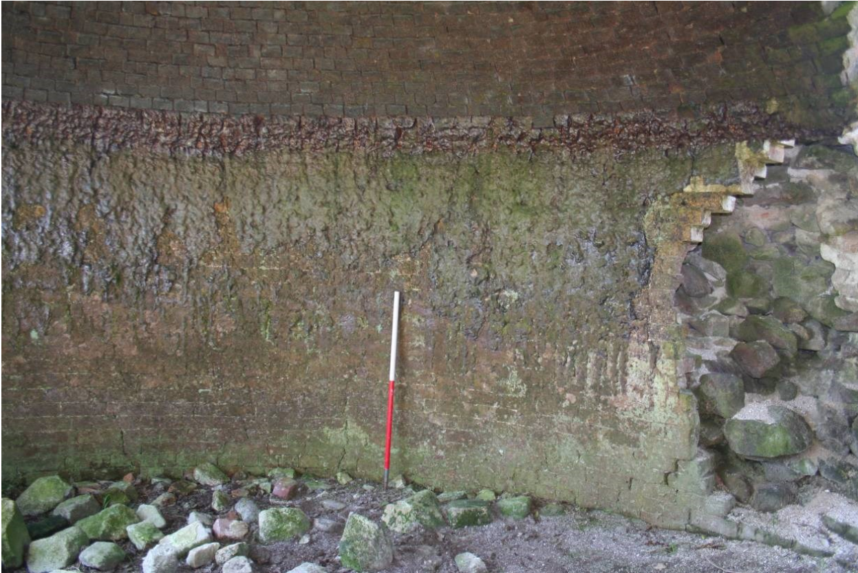
Fig 26 Interior of north wall of kiln showing vitrified brickwork in the upper half of the wall
