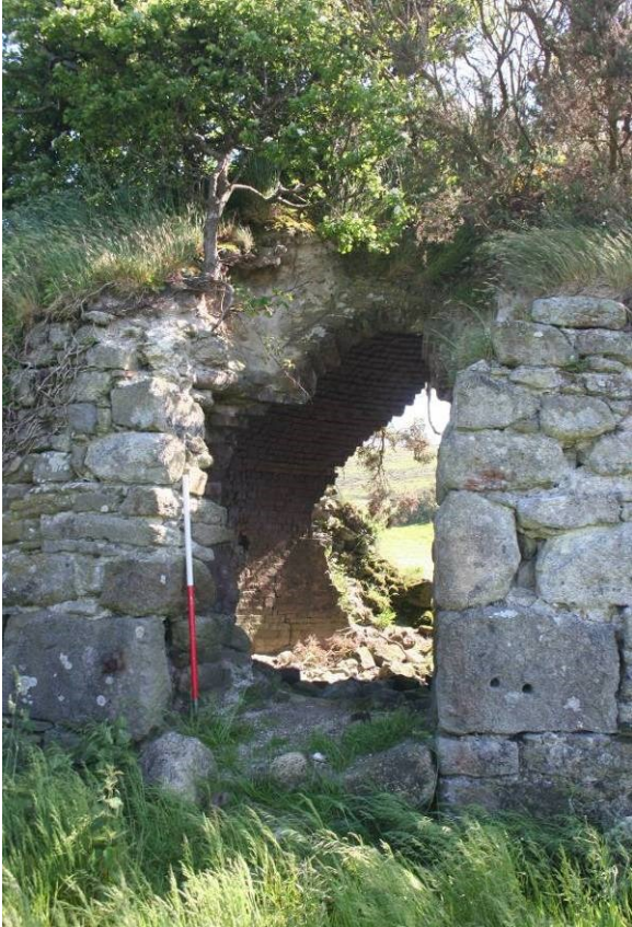
Fig 13 North-east loading door with collapsed arch and evidence for iron fittings
