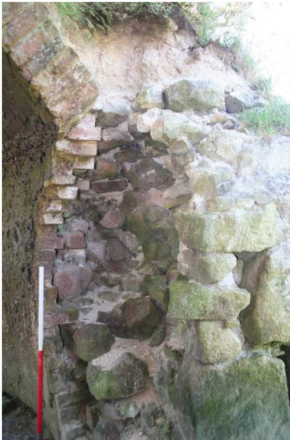
Fig 24 Collapse around north jamb of north-east loading door showing section through stone wall with brick lining and render roof covering
