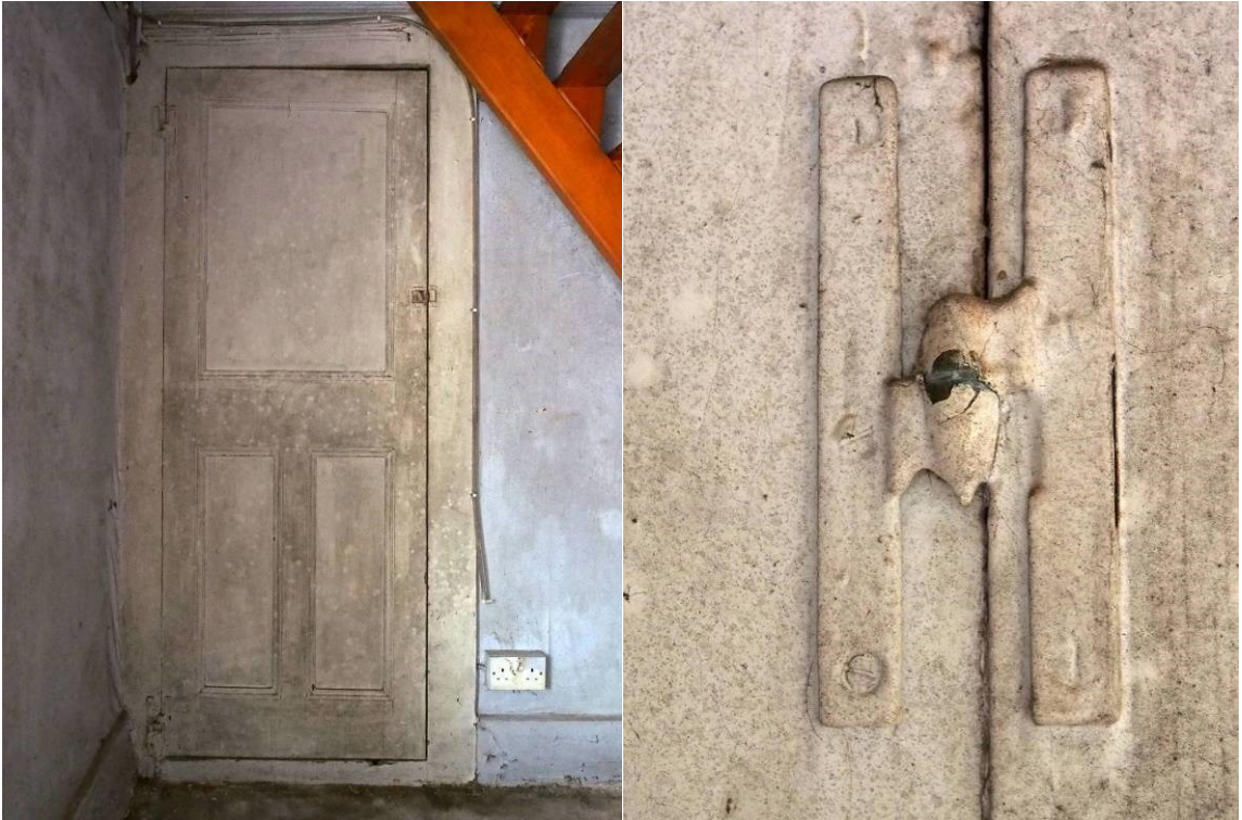
Fig 28 Ground floor former larder cupboard door and detail of eighteenth century H hinge
