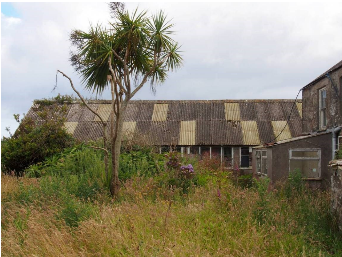
Fig 14 Part of the abandoned rear garden, with the flower packing shed in the background
