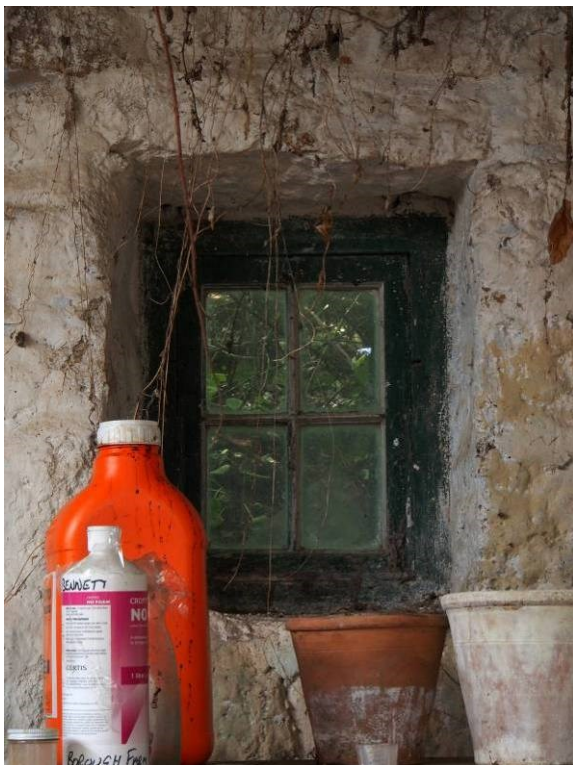
Fig 42 Original rear wooden window of cart house The window is designed to open on a central horizontal pivot
