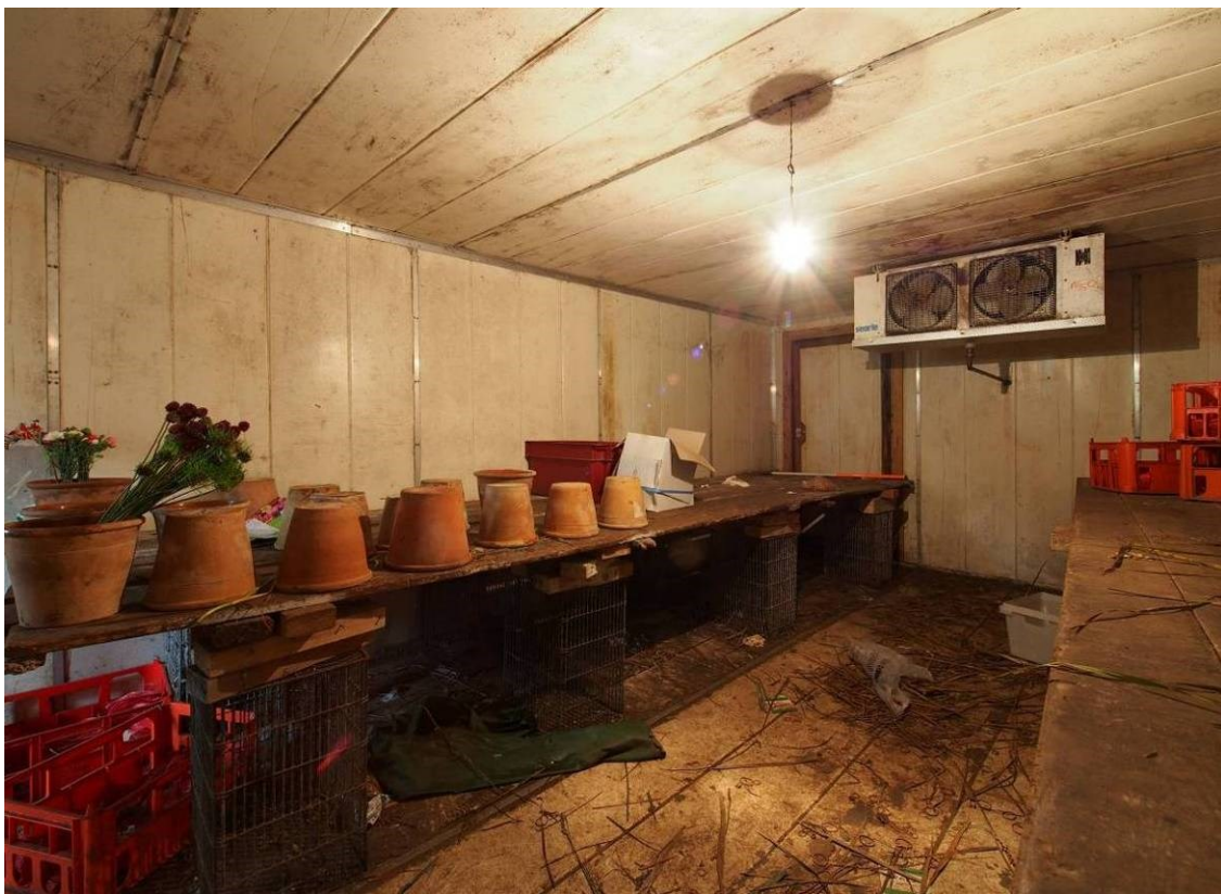
Fig 40 Interior of bulb cool room
