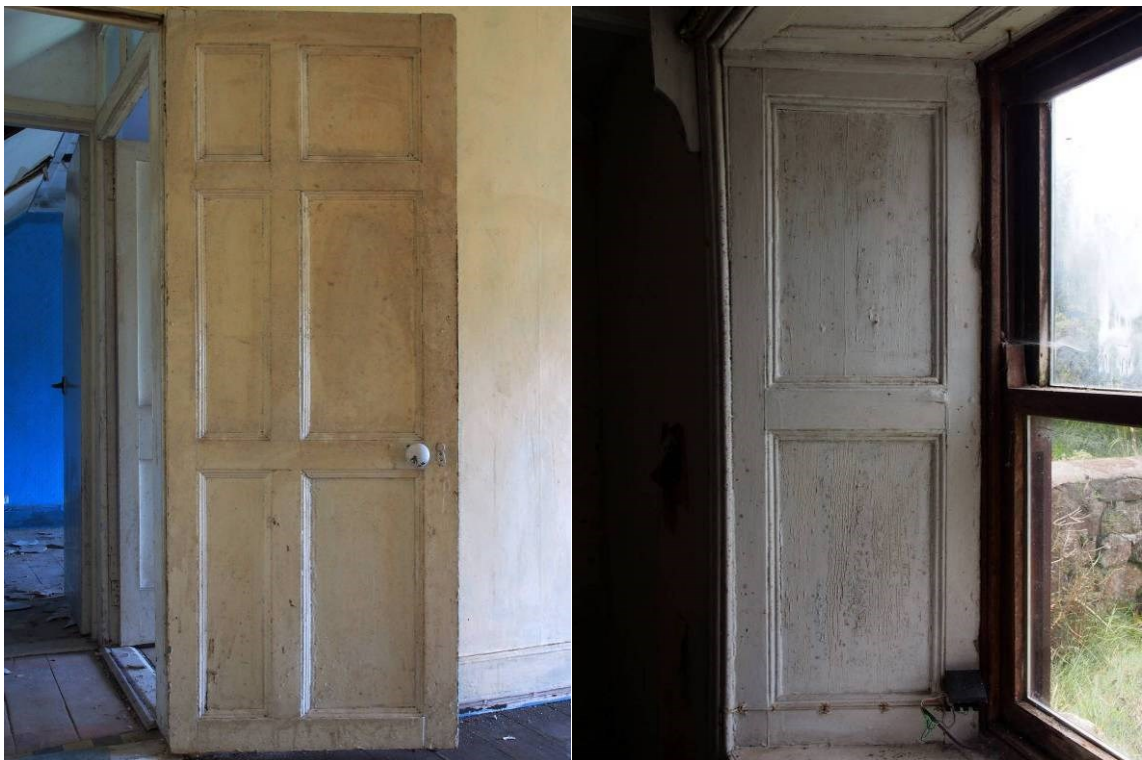
Fig 30 Examples of carpentry: reused (and narrowed) 6-panel door and double inset panels within front window reveals
