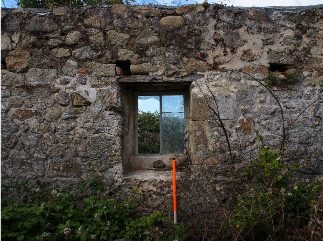
Fig 47 Interior of 'Fish house' showing reduced size of window frame and sockets for loft timbering
