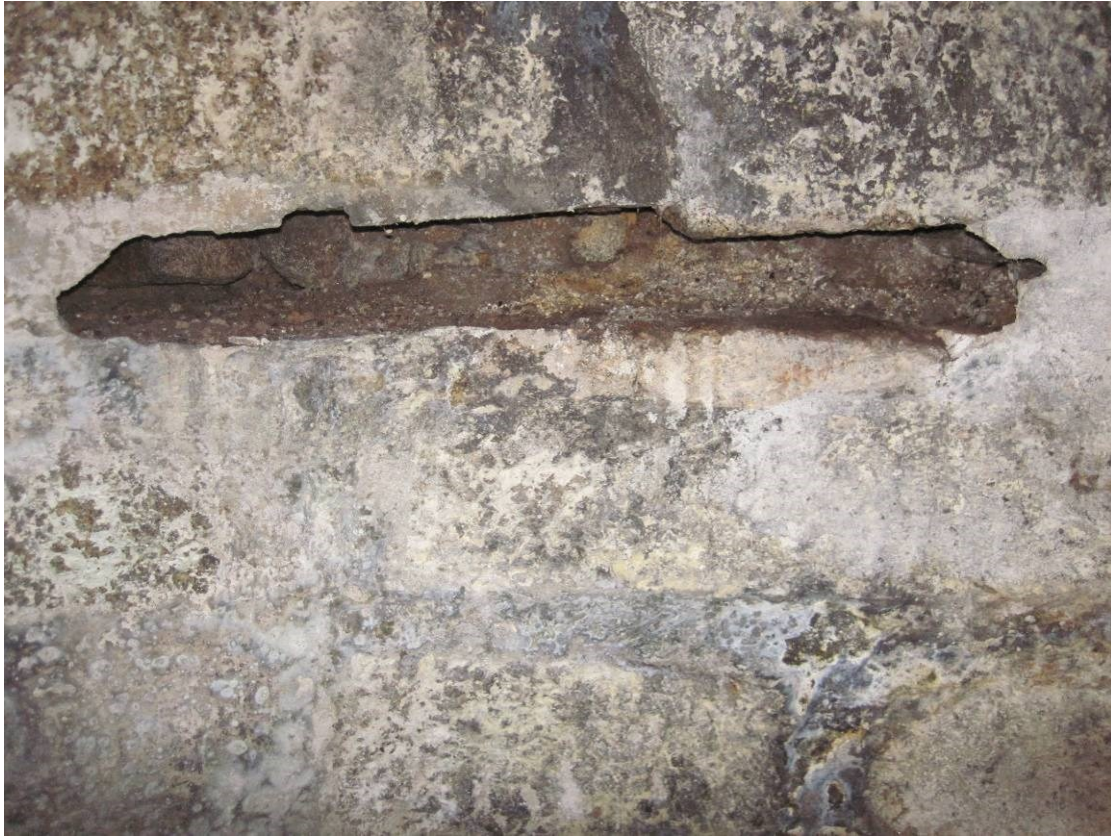
Fig 15 Possible shipwreck timber in second floor wall
