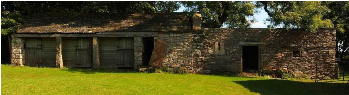
Fig 11 Barn 2: early 20 th century cartshed (left) and early 19 th century barn (right)
