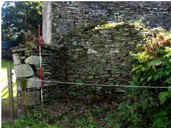
Fig 26 Remaining walling of former mid C19 building close to Barn 2, from W
