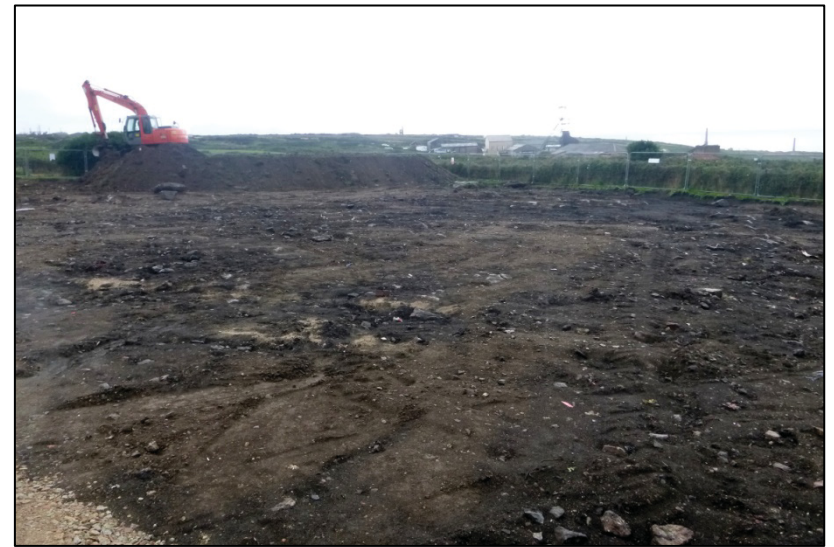
Figure 8. View of site after stripping showing nature of materials, view toward south west
