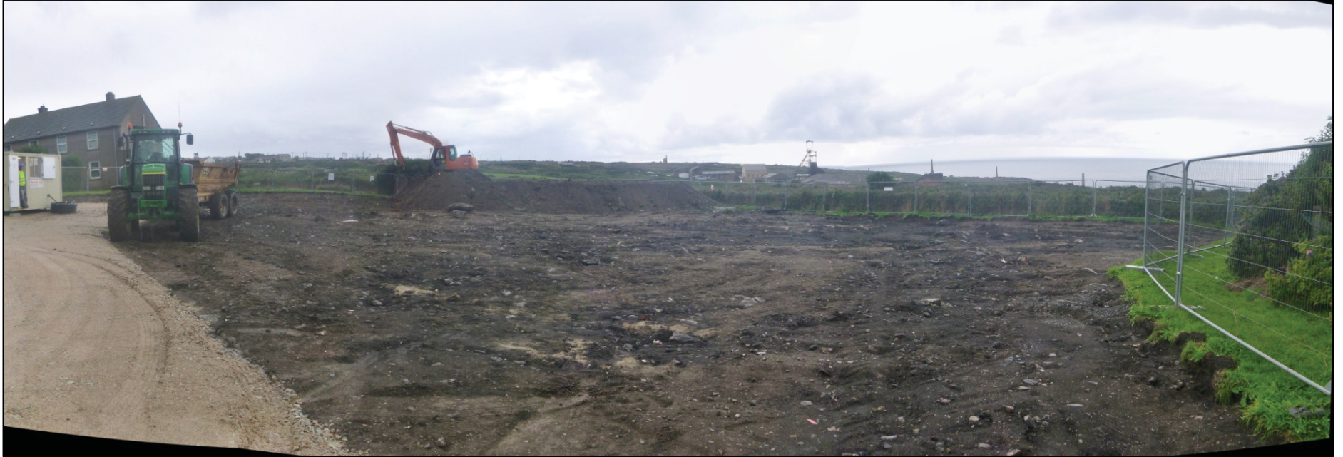
Figure 9. General view of site after stripping (View from NE corner looking south west)
