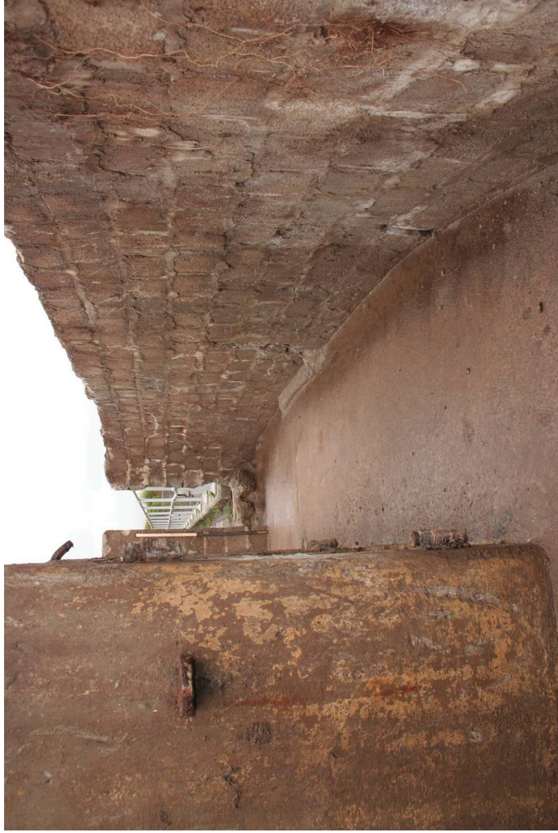
Fig 16 Passage along north side of emplacement, and north western entrance, facing west. The blockwork wall represents one of the modifications to the original layout of the gun pit (1m scale)
