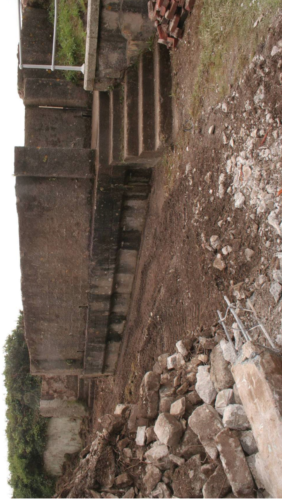
Fig 30 Northern exterior wall and north western entrance, facing south east (1m scale)
