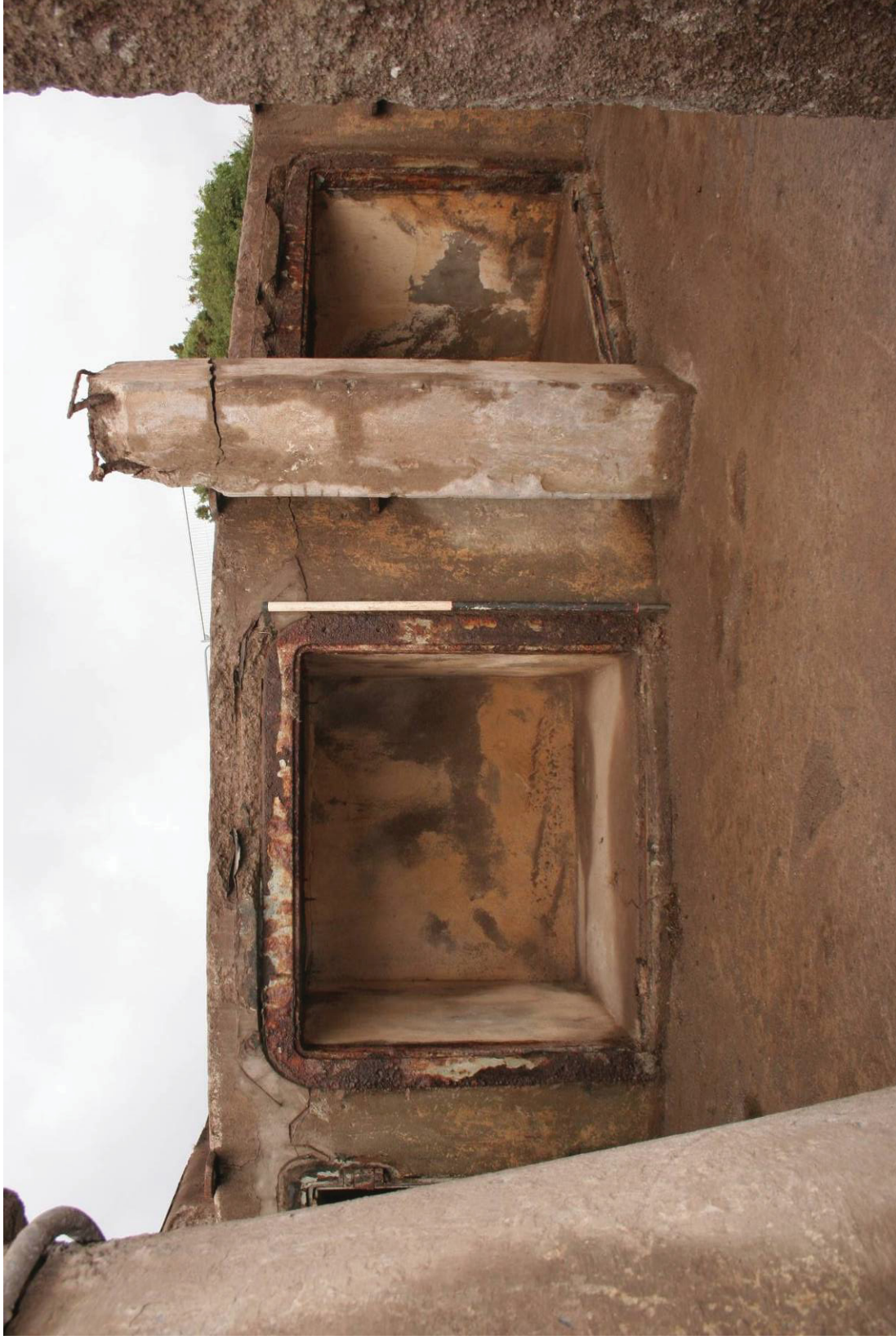
Fig 15 Stores 6 and 5 (l-r) and an anti-strafting roof pillar (r), facing west (1m scale)
