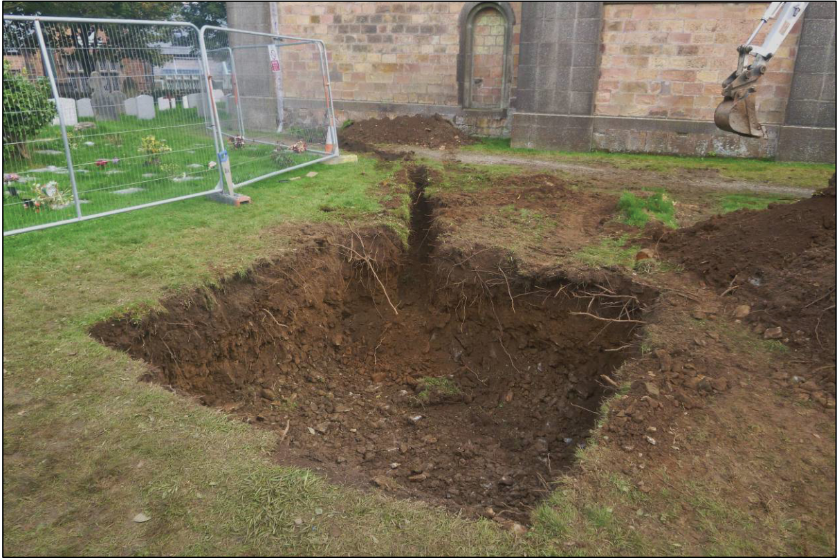
Figure 7. View looking east of completed excavation of soak-away with new the drainage trench.
