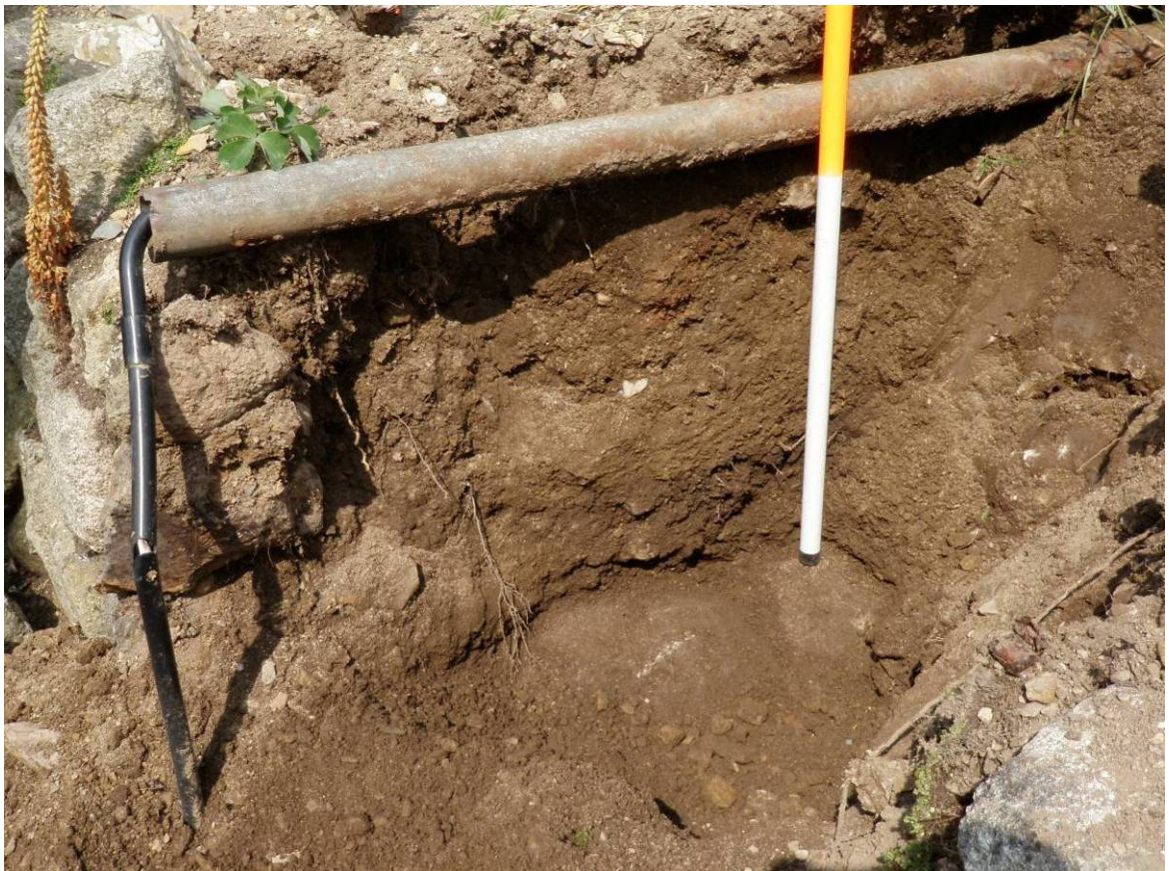
Fig 24 Slot cut into the lower terrace, showing probable paving at base of section
