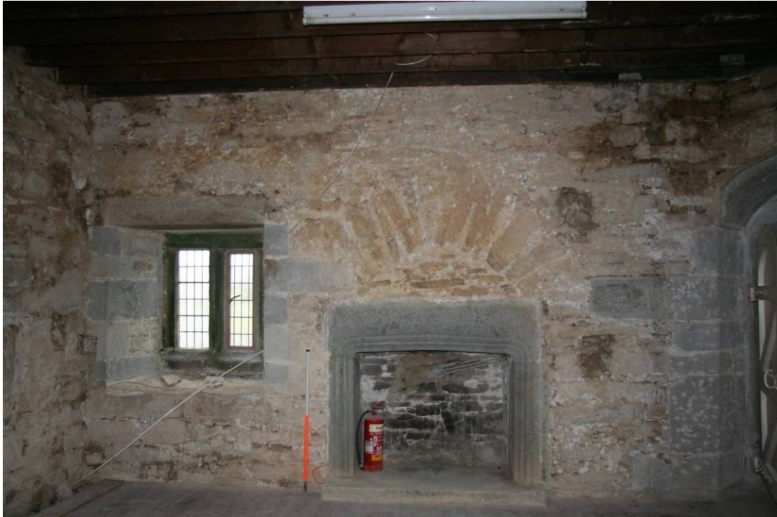
Fig 26 View of the third floor fireplace in the tower after modern finishes had been removed
