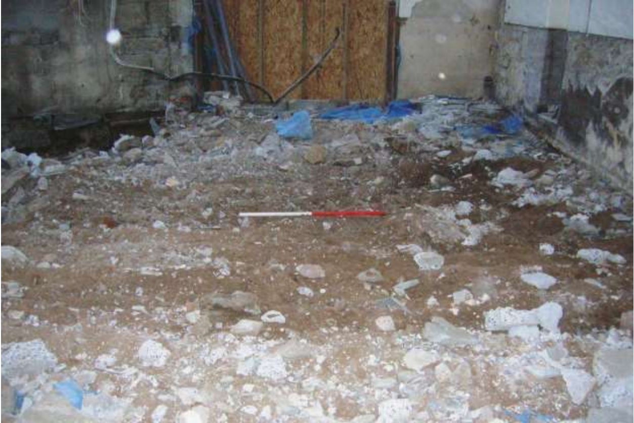
Figure 3: Looking northwest over the area of ground reduction at the rear of the building which shows modern building rubble and debris.
